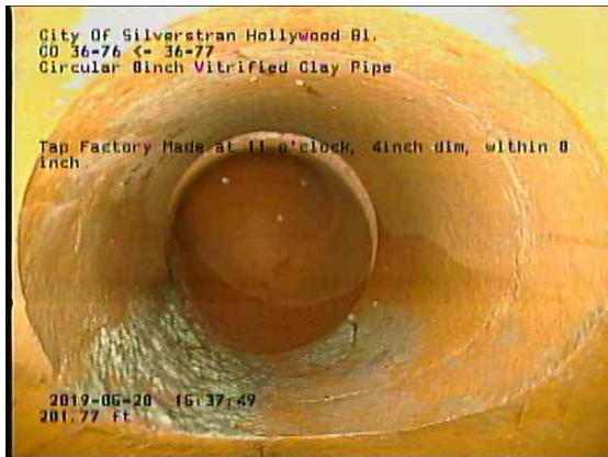
e01ae605-7b1c-4f82-a557-841566f7a1df_20190528_154023_715.jpg, 00:11:02, 201.77ft Tap Factory Made at 11 o'clock, 4inch dim, within 8 inch
