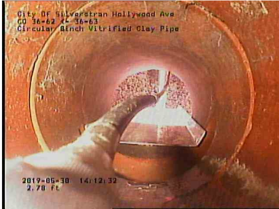
237c298d-27cc-4d5d-982f-701468cccc89_20190530_141507_842.jpg, 00:01:47, 0.21ft Tap Factory Made at 6 o'clock, 8inch dim, within 8 inch
