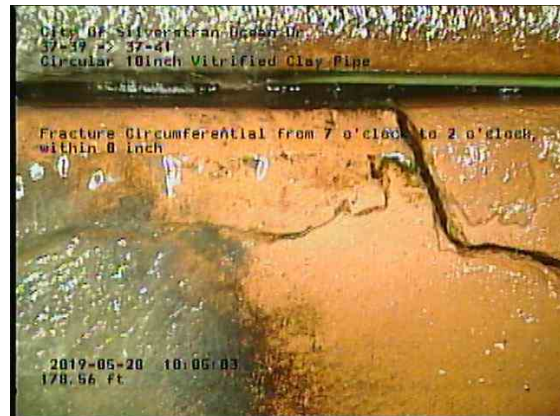
0558077d-a71c-4ded-8ecf-4fe194e68169_20190528_100736_645.jpg, 00:10:54, 178.56ft Fracture Circumferential from 7 o'clock to 2 o'clock, within 8 inch
