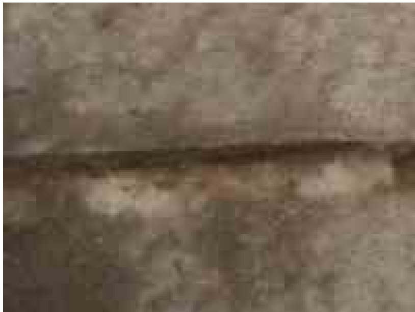
28-09_649da561_021a_4b6c_b8b5_5695380ff438_4699b76d-f272-4f57-a29f-4c5b9f8f7dc2_P11.jpg, , 2.65 Surface Reinforcement Corroded, from 04 to -01 o'clock, within 8 inch
