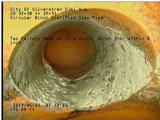
9b72aa8f-d123-40a2-9a05-904d3c504334_20190523_074654_672.jpg, 00:07:38, 125.55ft Tap Factory Made at 11 o'clock, 4inch dim, within 8 inch
