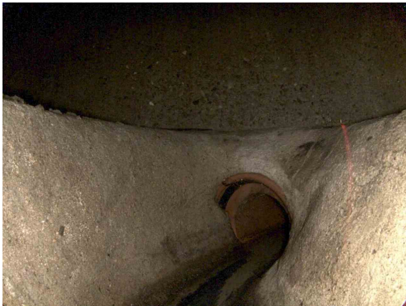
23-01_e8346f74_246f_46bb_9af3_39d1c680baea_4d0ccea5-eda1-4597-84ae-9c8824a08b4b_PI2.jpg, , 5.52 Surface Aggregate Visible from 4 o'clock to 7 o'clock, within 8 inch
