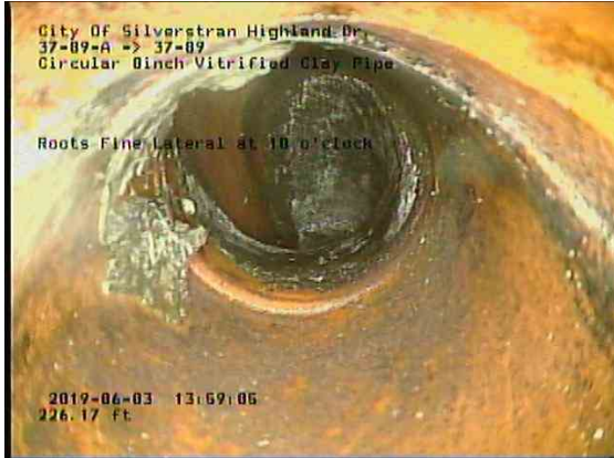
dac9128a-1ea4-4697-93ec-026bac764715_20190603_140142_324.jpg, 00:21:02, 226.17ft Roots Fine Lateral at 10 o'clock
