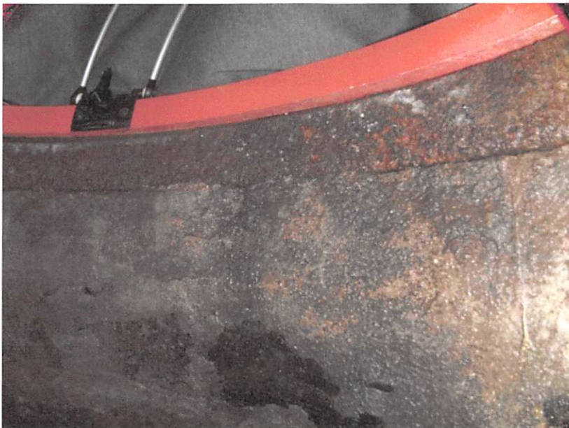
37-68_bc075bf7_3f28_485d_aaf8_7573fec9cbd6_262a9dd1-a25a-4fe9-a0ff-bd526de4f044_P12.jpg, , 0.16 Surface Roughness Increased from 12 o'clock to 12 o'clock, within 8 inch, Start
