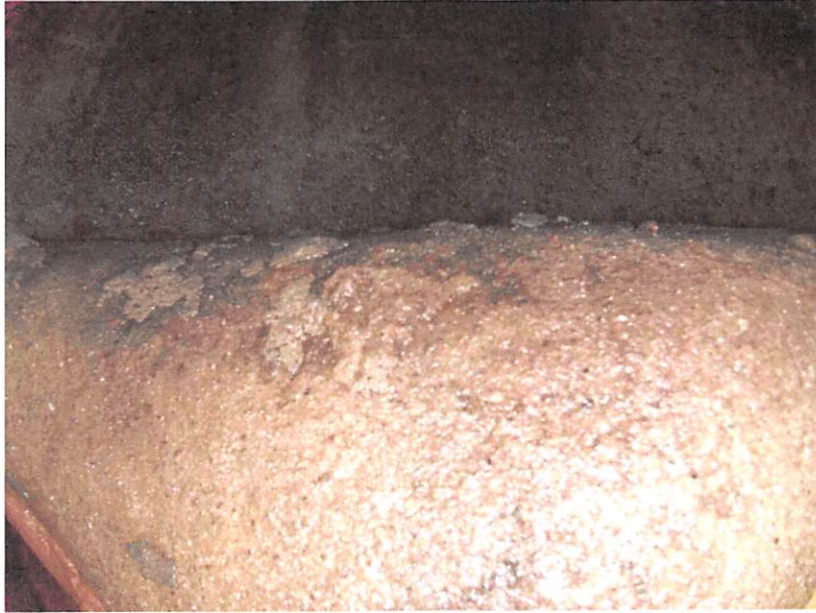
23-07_873817e9_0d4f_495f_ab7e_d928befa0923_11c85630-f555-492c-996a-d47226764506_PL12.jpg, , 8.39 Surface Roughness Increased from 12 o'clock to 12 o'clock, within 8 inch, Finish
