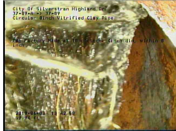
86774942-8d52-4e27-b462-b048e4fb3d4b_20190603_134534_730.jpg, 00:07:55, 59.94ft Tap Factory Made at 10 o'clock, 4inch dim, within 8 inch
