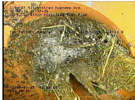
2e32f160-6892-4198-95e9-d29d8ac7168d_20190523_120332_096.jpg, 00:27:53, 432.71ft Tap Factory Made at 1 o'clock, 4inch dim, within 8 inch
