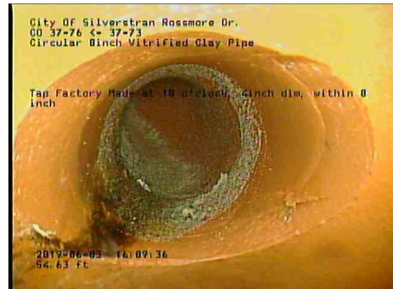
4622fffd-1a8c-4be4-89f9-92030f8038b6_20190603_161213_581.jpg, 00:03:37, 54.63ft Tap Factory Made at 10 o'clock, 4inch dim, within 8 inch
