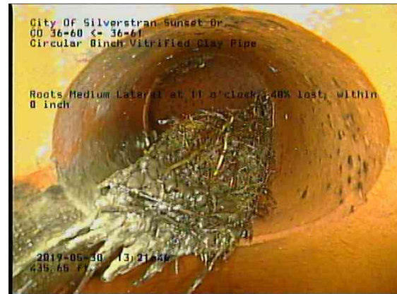
1a224b4e-8ed6-4e1b-9108-c6f99e4c0383_20190530_132421_711.jpg, 00:24:01, 435.65ft Roots Medium Lateral at 11 o'clock, 40% lost, within 8 inch
