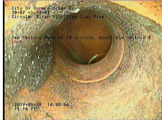
f8067e49-9b07-4874-9f19-87d52baa43a1_20190520_142326_197.jpg, 00:02:01, 11.16ft Tap Factory Made at 10 o'clock, 4inch dim, within 8 inch
