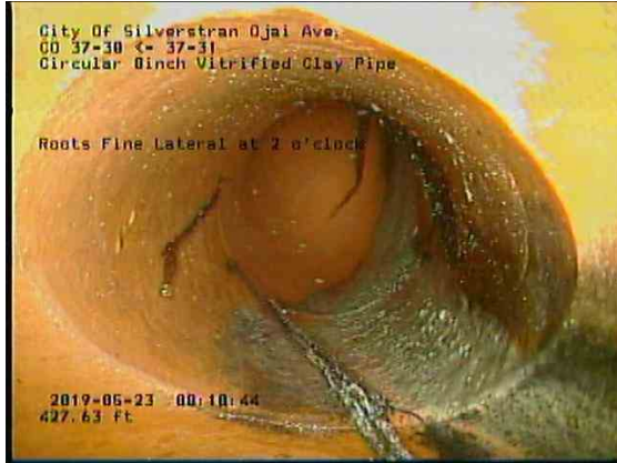
07c41698-b953-47ca-8087-e655fa303e63_20190523_081316_555.jpg, 00:27:03, 427.63ft Roots Fine Lateral at 2 o'clock
