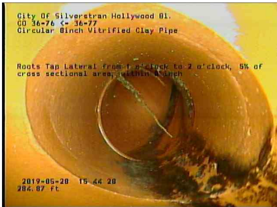
e32fa8f4-aa79-4207-9726-fa3ea743c5e8_20190528_154702_879.jpg, 00:16:09, 284.87ft Roots Tap Lateral from 1 o'clock to 2 o'clock, 5% of cross sectional area, within 8 inch
