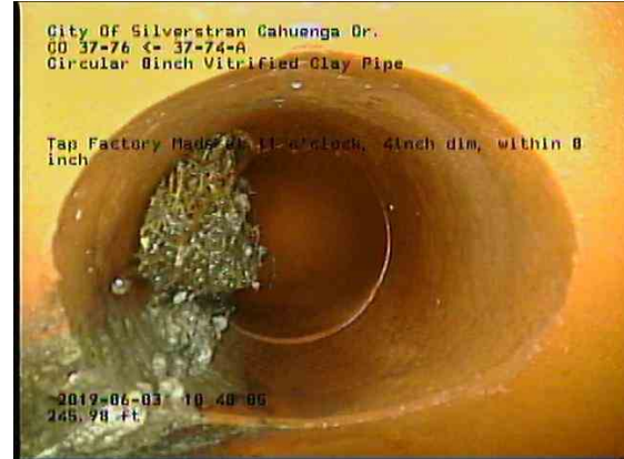
281efe10-516b-4b40-910d-555a0e418a6b_20190603_105041_781.jpg, 00:16:06, 245.98ft Tap Factory Made at 11 o'clock, 4inch dim, within 8 inch
