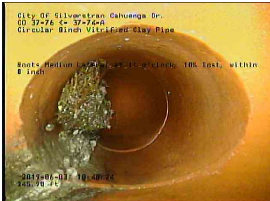
b4ba2aa7-1b5f-4464-ac34-2c2a0c009692_20190603_105100_625.jpg, 00:16:08, 245.98ft Roots Medium Lateral at 11 o'clock, 10% lost, within 8 inch
