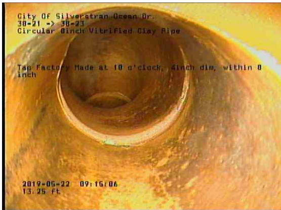
fec67a81-09ad-4c0f-9db7-f73325789723_20190522_091737_128.jpg, 00:01:15, 13.25ft Tap Factory Made at 10 o'clock, 4inch dim, within 8 inch
