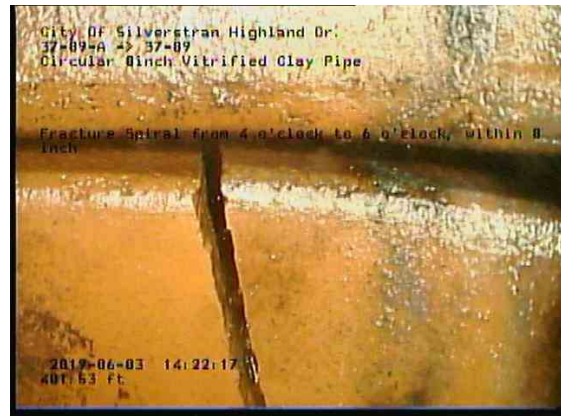
c345688a-29e1-4312-875c-0e4e2965ebea_20190603_142454_200.jpg, 00:36:02, 401.53ft Fracture Spiral from 4 o'clock to 6 o'clock, within 8 inch
