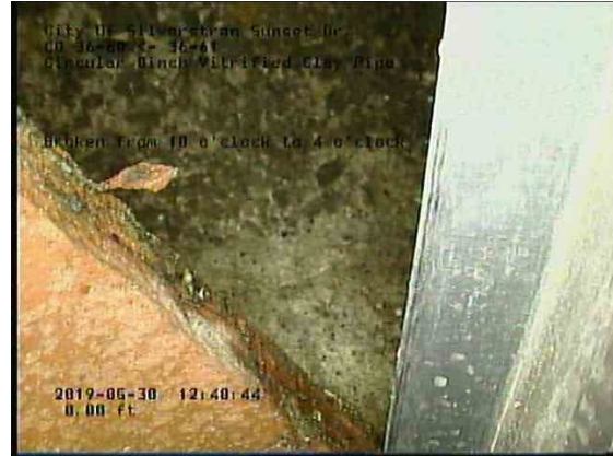
9afce06e-3576-4258-8442-d6d4f40f457a_20190530_125119_987.jpg, 00:00:35, 0.00ft Broken from 10 o'clock to 4 o'clock
