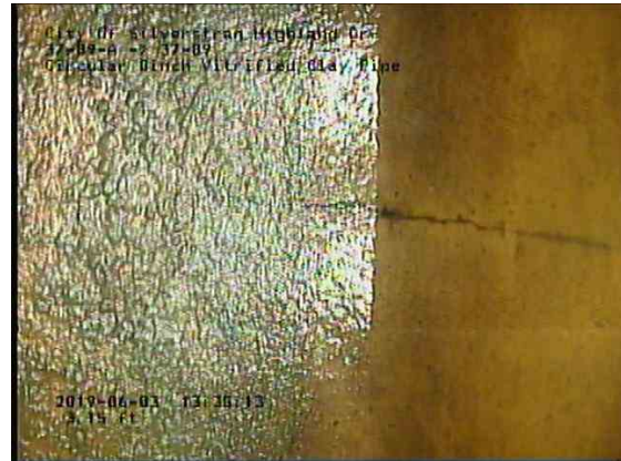
59456fa1-f0a4-4032-a008-d881fd339b08_20190603_133750_581.jpg, 00:02:41, 3.15ft Fracture Circumferential from 4 o'clock to 10 o'clock
