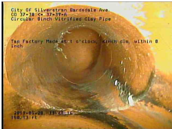
e2453816-9d51-4960-99af-d59e9e7ac166_20190528_115048_993.jpg, 00:10:16, 150.12ft Tap Factory Made at 1 o'clock, 4inch dim, within 8 inch
