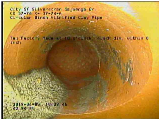
0f790c4e-7bbc-4f6b-9759-078f3831ce16_20190603_103222_277.jpg, 00:02:37, 42.94ft Tap Factory Made at 10 o'clock, 4inch dim, within 8 inch
