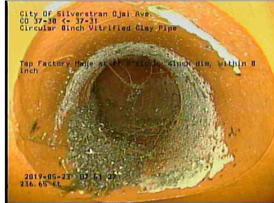
43213f2f-3379-4d99-9097-f65c676efc98_20190523_075400_132.jpg, 00:13:37, 236.65ft Tap Factory Made at 11 o'clock, 4inch dim, within 8 inch
