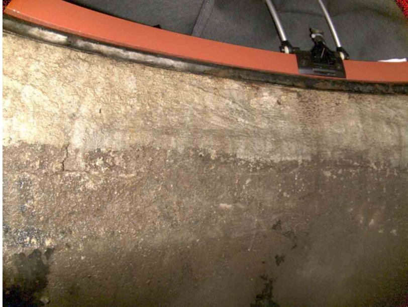
38-23_526f34cb_e675_4ea0_9cf9_0970110d8ccb_0e69838e-69cb-42bf-84b4-e508add5a327_P12.jpg, , 0.33 Crack Longitudinal at 10 o'clock, within 8 inch
