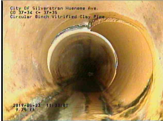
cde2528d-3ef4-4d14-99fa-e57159509e8f_20190523_113534_804.jpg, 00:04:05, 11.67ft Infiltration Gusher at 9 o'clock, within 8 inch
