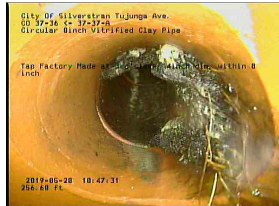
54ad9c28-6df1-4a30-a280-b1c99d190a32_20190528_105005_076.jpg, 00:15:33, 256.60ft Tap Factory Made at 3 o'clock, 4inch dim, within 8 inch
