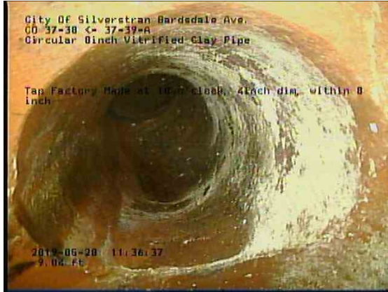
105ff841-2ca6-42e9-b051-2cfb52e459c8_20190528_113911_286.jpg, 00:01:02, 9.04ft Tap Factory Made at 10 o'clock, 4inch dim, within 8 inch
