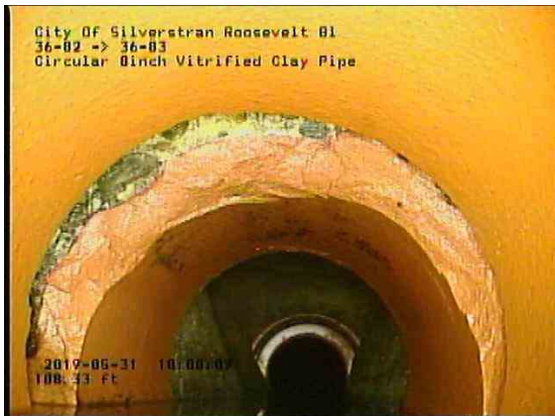
fa97e13a-8073-485d-b725-8e49419da088_20190531_101046_431.jpg, 00:08:56, 109.35ft Broken from 7 o'clock to 5 o'clock
