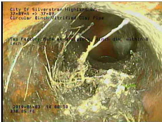
1ed8c1c9-5400-4ac6-8f94-8ac3d586aca4_20190603_140315_332.jpg, 00:22:16, 238.85ft Tap Factory Made at 2 o'clock, 4inch dim, within 8 inch
