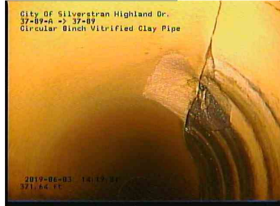
f7135f73-7691-4e17-b6bb-926a75e917fc_20190603_142228_519.jpg, 00:33:36, 372.19ft Infiltration Weeper at 2 o'clock
