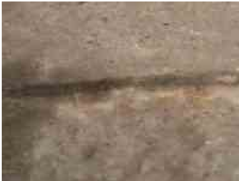
28-09_649da561_021a_4b6c_b8b5_5695380ff438_32a59c61-a6ba-4cd0-bd9a-85c83e97f5d5_P11.jpg, , 2.34 Surface Reinforcement Corroded, from 04 to -01 o'clock, within 8 inch
