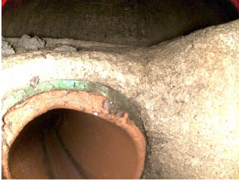
23-01_e8346f74_246f_46bb_9af3_39d1c680baea_80daa081-70dc-4ab4-86bc-08fcb2345a18_P12.jpg, , 5.68 Obstacles Construction Debris, 5% of cross sectional area from 10 o'clock to 11 o'clock
