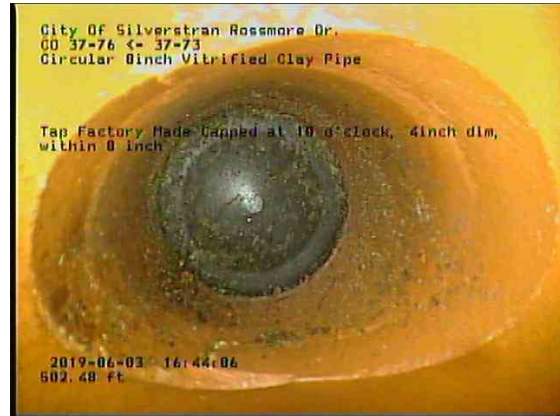
eba2059f-e377-4424-ab73-8dedb3bf34b3_20190603_164644_046.jpg, 00:31:10, 502.48ft Tap Factory Made Capped at 10 o'clock, 4inch dim, within 8 inch
