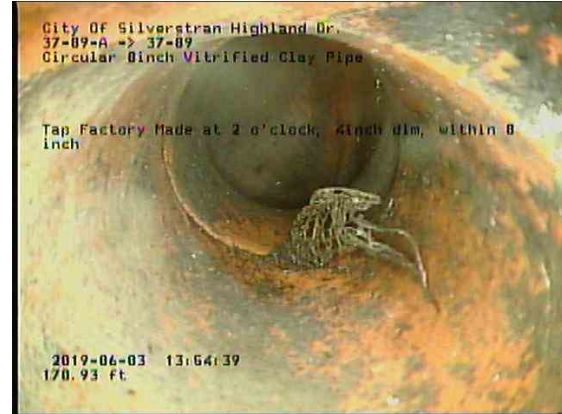
5fe319e3-0c9c-40d7-b638-3111ec100497_20190603_135716_038.jpg, 00:17:28, 170.93ft Tap Factory Made at 2 o'clock, 4inch dim, within 8 inch
