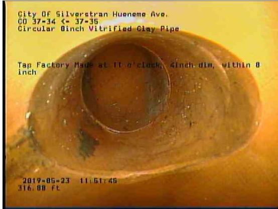
f3946b85-3c01-4649-97bb-4ab276e7f49f_20190523_115418_180.jpg, 00:20:10, 316.88ft Tap Factory Made at 11 o'clock, 4inch dim, within 8 inch
