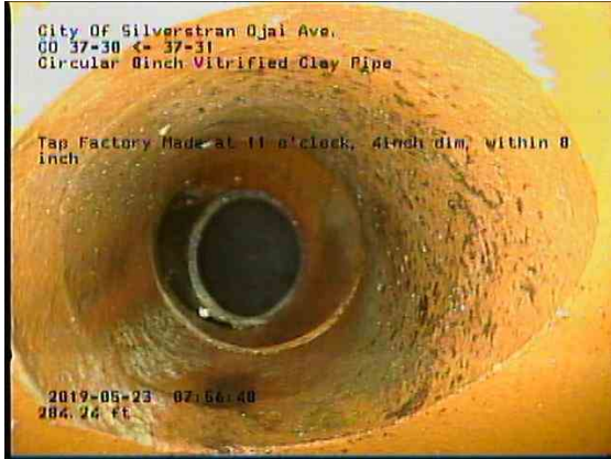
4056b91d-5903-40ea-adbb-670097fd0b3b_20190523_075920_781.jpg, 00:16:39, 284.24ft Tap Factory Made at 11 o'clock, 4inch dim, within 8 inch
