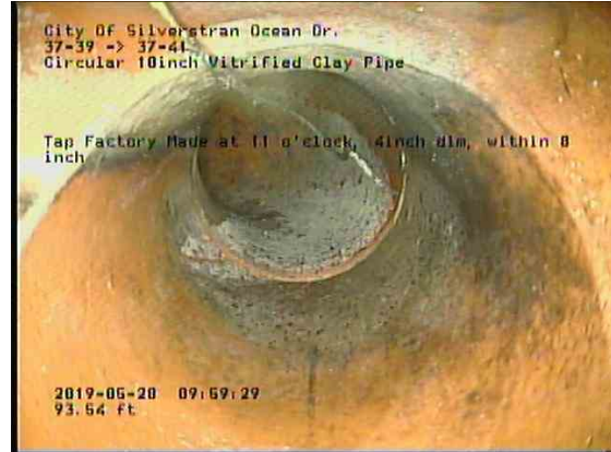
c5a5f608-9644-46f5-948f-71be30178114_20190528_100202 _607.jpg, 00:06:20, 93.54ft Tap Factory Made at 11 o'clock, 4inch dim, within 8 inch
