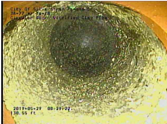
beaa3cb3-139a-4b27-9d55-1d935203b617_20190529_083156_322.jpg, 00:14:41, 130.49ft Tap Factory Made Capped at 2 o'clock, 4inch dim, within 8 inch
