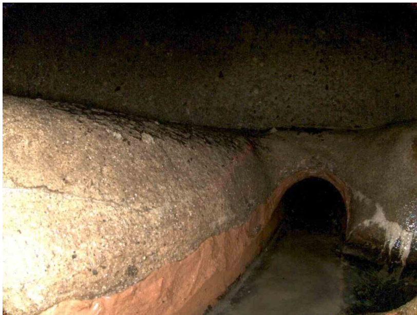
38-23_526f34cb_e675_4ea0_9cf9_0970110d8ccb_731a3224-862f-4427-a1c2-ba49ed2c6bef_P12.jpg, , 8.50 Surface Roughness Increased from 12 o'clock to 12 o'clock, within 8 inch, Finish
