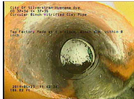
c3f306f6-f0da-4442-b38f-034eaebd1be1_20190523_114507_828.jpg, 00:12:58, 186.02ft Tap Factory Made at 1 o'clock, 4inch dim, within 8 inch
