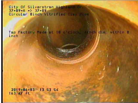
7aa086af-c9bf-4f04-99db-a5d7095799ec_20190603_135631_184.jpg, 00:16:50, 163.47ft Tap Factory Made at 10 o'clock, 4inch dim, within 8 inch
