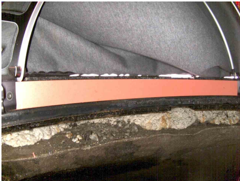
36-78_f20e677b_8ab5_4247_8921_13ab7193ed33_13c053e4-4df7-4ac6-b56f-3c16d1ccc7e3_P12.jpg, , -0.10 Surface Roughness Increased from 12 o'clock to 12 o'clock, within 8 inch
