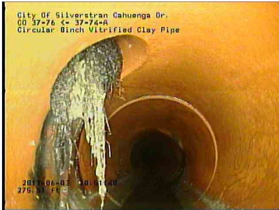
81fc2289-2339-4ae8-a6fa-879cdf9a27f5_20190603_105416_491.jpg, 00:17:53, 276.25ft Roots Ball Lateral at 10 o'clock, 90% lost, within 8 inch
