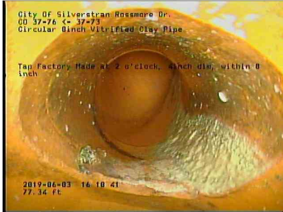
92355246-d714-485a-8609-b0846717d90e_20190603_161318_771.jpg, 00:04:35, 77.34ft Tap Factory Made at 2 o'clock, 4inch dim, within 8 inch
