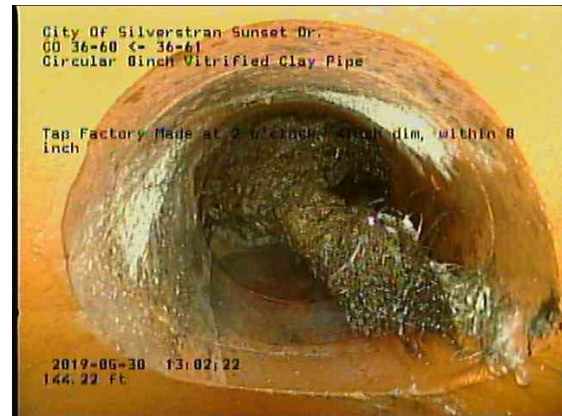
3cecd5b-8123-4ed6-9fc7-0328c5f97a70_20190530_130457_566.jpg, 00:08:43, 144.21ft Tap Factory Made at 2 o'clock, 4inch dim, within 8 inch
