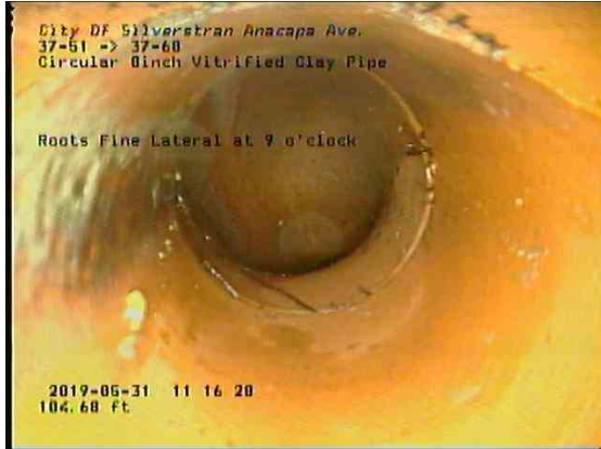
2ca49ca8-0720-43cd-beb5-b13d3a79189a_20190531_111905_450.jpg, 00:04:31, 104.68ft Roots Fine Lateral at 9 o'clock
