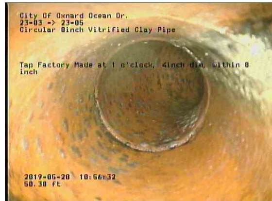
b872f605-3344-40be-8d4d-f736cdfef25b_20190520_105902_319.jpg, 00:02:44, 50.38ft Tap Factory Made at 1 o'clock, 4inch dim, within 8 inch
