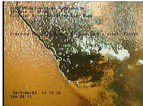
c5686161-2276-4e31-b9d2-d79af85fa2a5_20190603_142008_958.jpg, 00:32:14, 366.88ft Fracture Multiple from 3 o'clock to 6 o'clock, Finish
