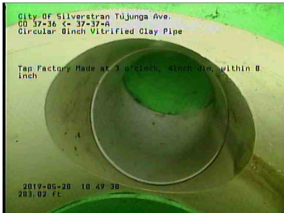
5ff92bfa-34ba-4b65-ae1-07c6a9332596_20190528_105203_774.jpg, 00:16:54, 283.02ft Tap Factory Made at 3 o'clock, 4inch dim, within 8 inch
