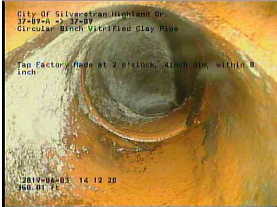
a0c05996-22ea-4d0f-b02c-46acb63a54b1_20190603_141505_240.jpg, 00:28:26, 350.01ft Tap Factory Made at 2 o'clock, 4inch dim, within 8 inch
