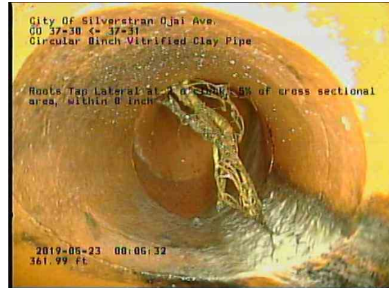
327eca71-38e1-4f42-a666-5c15df3f6b2b_20190523_080804_959.jpg, 00:22:58, 361.99ft Roots Tap Lateral at 2 o'clock, 5% of cross sectional area, within 8 inch
