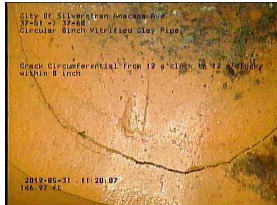
2c22ff67-d59f-4902-9dbd-11ca826950e4_20190531_112244_173.jpg, 00:07:24, 146.97ft Crack Circumferential from 12 o'clock to 12 o'clock, within 8 inch / In WYE
