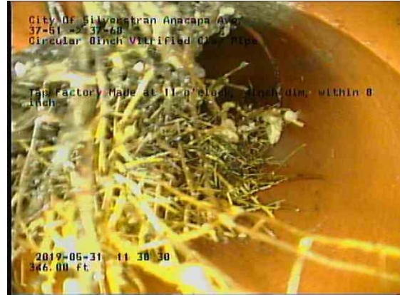
72dcc718-3b23-45b3-8b24-7321bd989157_20190531_114107_353.jpg, 00:20:38, 346.00ft Tap Factory Made at 11 o'clock, 4inch dim, within 8 inch
