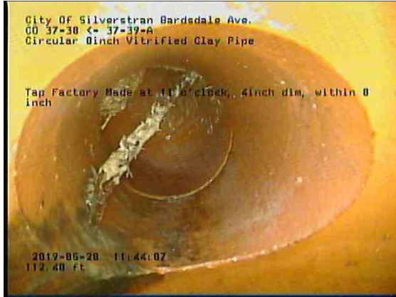
108089f2-3944-4d2a-afc3-3a38a37ca4f9_20190528_114641_122.jpg, 00:07:16, 112.40ft Tap Factory Made at 11 o'clock, 4inch dim, within 8 inch
