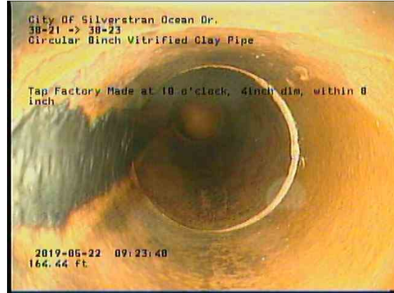
c6c706a9-f0d9-4123-81b4-fd9e4083e829_20190522_092611_759.jpg, 00:08:53, 164.44ft Tap Factory Made at 10 o'clock, 4inch dim, within 8 inch
