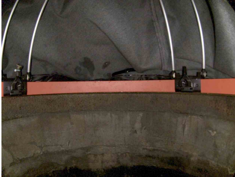
37-51_34621632_ace1_4c3b_9051_30e3d1d9a3a6_225cb988-2a8b-4a50-97ac-5af06f6feb0_P12.jpg, , -0.57 Reversal Inspection
