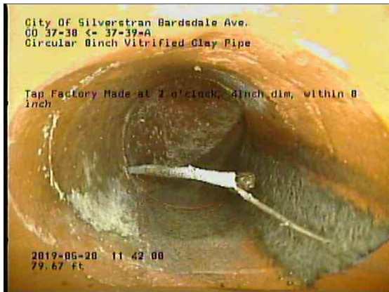
cdbf6c8c-b038-4e9a-93bc-ab95774a831d_20190528_114434_383.jpg, 00:05:30, 79.67ft Tap Factory Made at 2 o'clock, 4inch dim, within 8 inch
