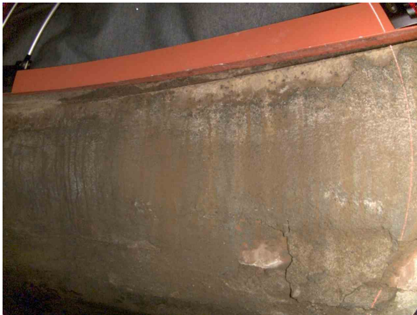
23-03_caf8412c_d397_4fc6_88c9_a9658e397a0b_326c5f2a-4e51-4bcd-ba9e-dfb18088910f_P12.jpg, , 0.04 Surface Roughness Increased from 12 o'clock to 12 o'clock, within 8 inch, Start
