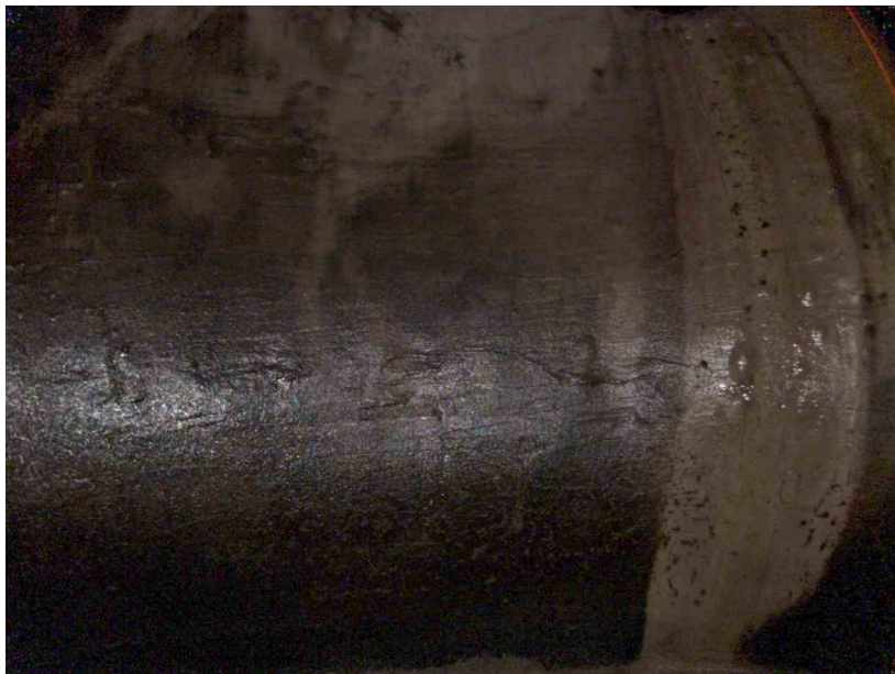
37-89_b7b73460_144a_4a36_a05d_2d26ddf59287_b1ce53f6-c38b-4399-a014-cac116379f5e_P12.jpg, , 8.11 Lining Failure Blistered at 9 o'clock, within 8 inch
