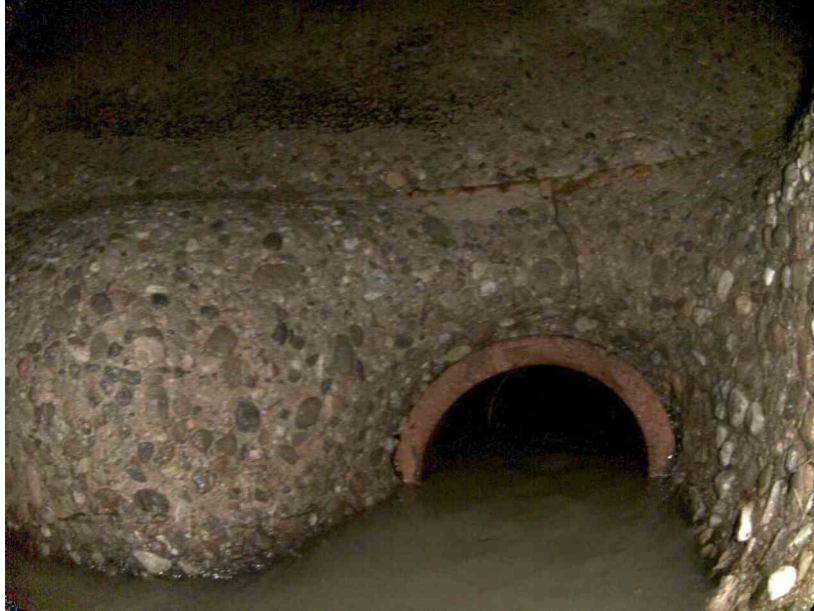
37-39_e3463806_251b_4a10_8598_66aa7b2b50ab_755413a1-c448-44fd-afd8-7411036d9010_P12.jpg, , 5.50 Surface Aggregate Visible from 12 o'clock to 12 o'clock, within 8 inch, Finish
