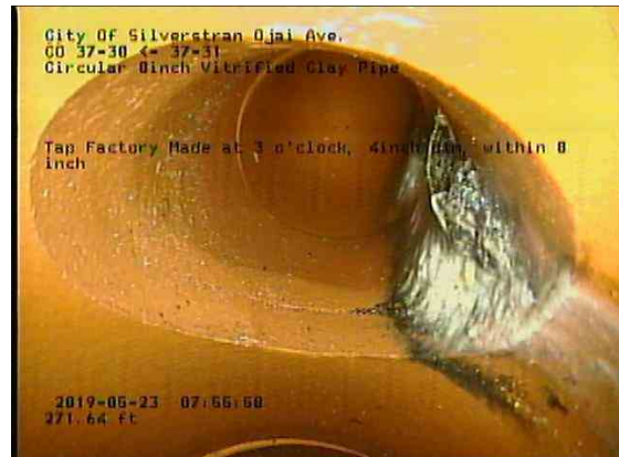
36101567-fcdd-4980-b567-776aea8743f7_20190523_075830_986.jpg, 00:15:57, 271.64ft Tap Factory Made at 3 o'clock, 4inch dim, within 8 inch
