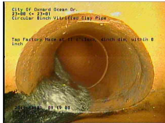
90d2d25d-8219-4fe0-9624-e08bf7695c9c_20190521_092138_008.jpg, 00:05:29, 135.17ft Tap Factory Made at 11 o'clock, 4inch dim, within 8 inch
