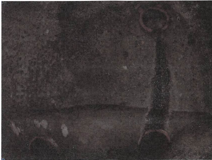
37-68_bc075bf7_3f28_485d_aaf8_7573fec9cbd6_cceabf30-0668-4f75-8b7e-afd5d7217628_P12.jpg, , 7.64 Infiltration Stain at 8 o'clock, within 8 inch
