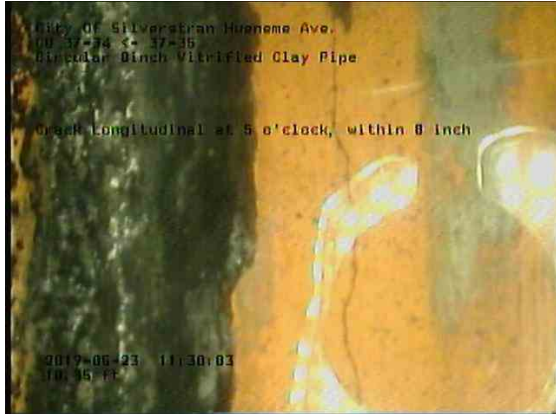
1184433c-b93c-4820-880a-402e2e7017fb_20190523_113236_564.jpg, 00:02:37, 10.35ft Crack Longitudinal at 5 o'clock, within 8 inch
