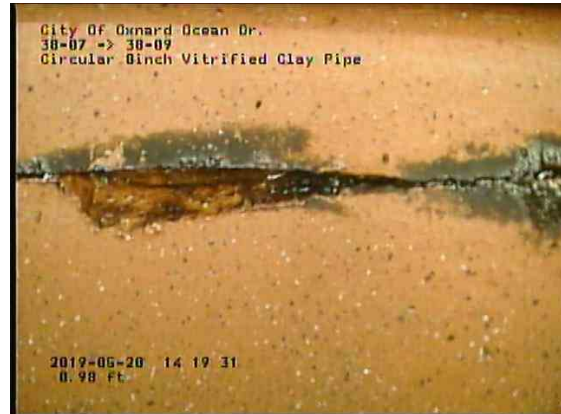
19ecd0b4-8c6e-4d0b-8cfc-cecbbac1ec7c_20190520_142201_684.jpg, 00:00:50, 0.98ft Fracture Circumferential from 12 o'clock to 12 o'clock, within 8 inch
