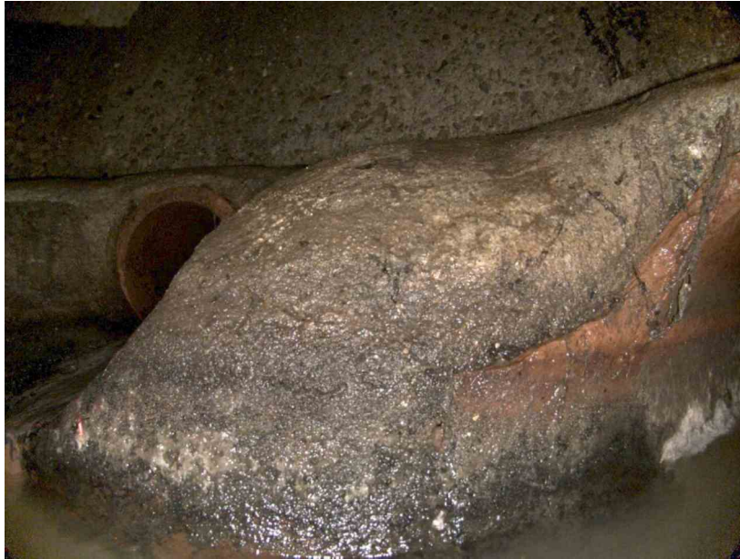
37-39_f9d93fbc_2737_41bc_8eac_424990064008_924f64bc-7839-4063-812e-13cbcd2df3f2_P12.jpg, , 4.79 Surface Roughness Increased from 12 o'clock to 12 o'clock, within 8 inch, Finish
