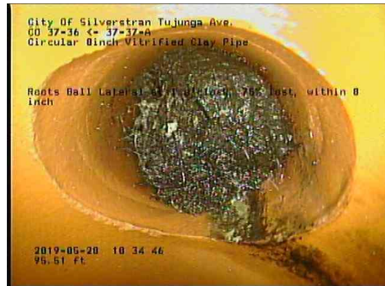
82456bb5-57ff-4ff7-9ae0-a721d61252cd_20190528_103719_326.jpg, 00:06:28, 95.51ft Roots Ball Lateral at 1 o'clock, 75% lost, within 8 inch
