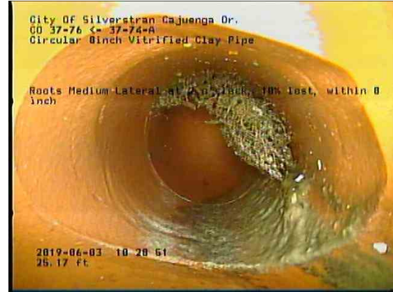
e4eb9c59-b554-450a-82f5-5b1f0e31288a_20190603_103127_685.jpg, 00:01:49, 25.17ft Roots Medium Lateral at 2 o'clock, 10% lost, within 8 inch
