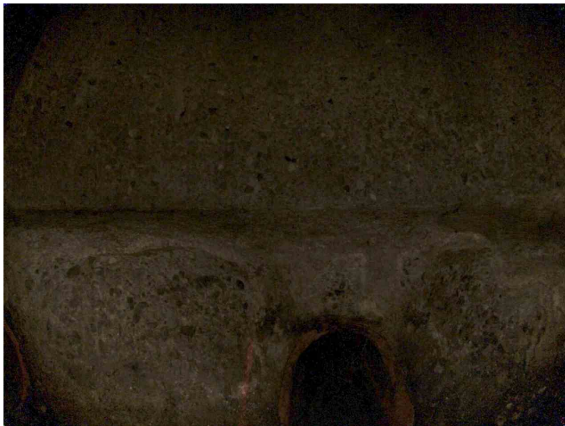
23-03_caf8412c_d397_4fc6_88c9_a9658e397a0b_77c5866e-44b5-4138-a1ec-8e62c1cd4f1e_P12.jpg, , 7.27 Surface Roughness Increased from 12 o'clock to 12 o'clock, within 8 inch, Finish
