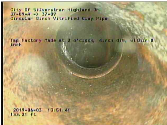
c3e2bea2f-e5ad-4cb2-bb58-8e5b6bb07edf_20190603_135418_155.jpg, 00:14:52, 133.21ft Tap Factory Made at 2 o'clock, 4inch dim, within 8 inch
