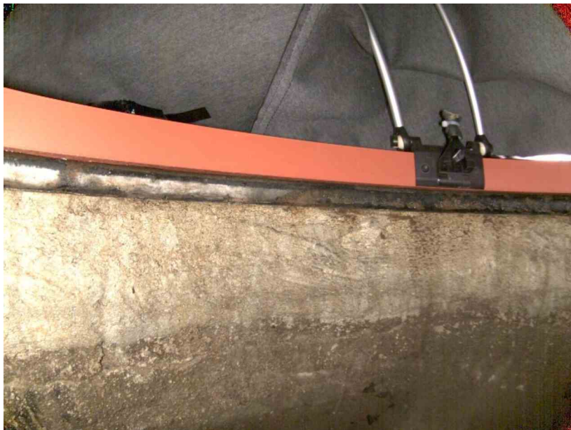
38-23_526f34cb_e675_4ea0_9cf9_0970110d8ccb_85058784-e68f-4e8a-b7b5-7a0fe87d2468_P12.jpg, , 0.02 Surface Roughness Increased from 12 o'clock to 12 o'clock, within 8 inch, Start
