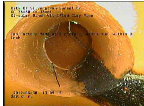
10e828e2-82b3-401b-a738-8aece52faee8_20190530_131148_995.jpg, 00:14:06, 249.40ft Tap Factory Made at 2 o'clock, 4inch dim, within 8 inch
