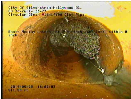
6c9f030c-b63b-405f-a203-f27e1cb90c0f_20190528_160437_460.jpg, 00:30:23, 511.50ft Roots Medium Lateral at 2 o'clock, 45% lost, within 8 inch
