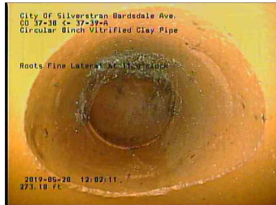
62ef9976-078e-4510-83cf-70e596401994_20190528_120445_660.jpg, 00:20:04, 273.18ft Roots Fine Lateral at 11 o'clock
