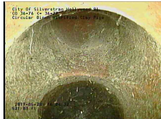
81dac533-9d54-40c0-a114-faeadc2cbd4_20190528_160706_667.jpg, 00:31:38, 521.27ft Tap Factory Made at 12 o'clock, 8inch dim, within 8 inch
