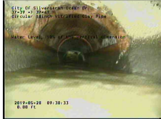
e7d00bad-ac16-446d-929e-8deb37c1cc05_20190528_094106_611.jpg, 00:00:08, 0.00ft Water Level, 10% of the vertical dimension
