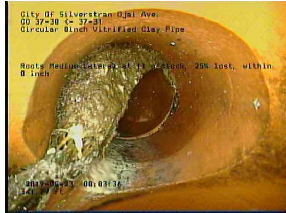
88cb7be9-42b9-4781-b6bc-6d93b3e150a4_20190523_080609_297.jpg, 00:21:31, 341.79ft Roots Medium Lateral at 11 o'clock, 25% lost, within 8 inch
