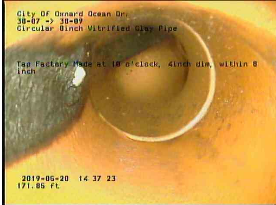
1cba3397-a263-43f3-b198-b5fae6a086ca_20190520_143953_702.jpg, 00:14:19, 171.85ft Tap Factory Made at 10 o'clock, 4inch dim, within 8 inch
