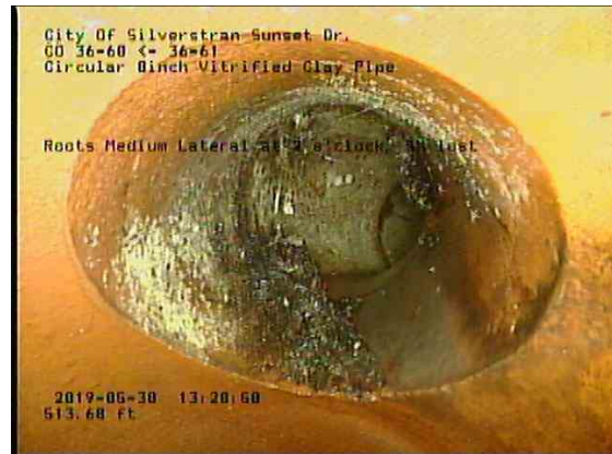
61f107ae-63dc-44c0-a5c3-9b284ca2fa3f_20190530_133125_135.jpg, 00:29:20, 513.68ft Roots Medium Lateral at 2 o'clock, 5% lost
