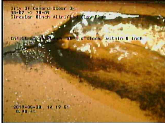
07ae68d6-e9d1-47e5-9685-bbdbfb5c49f6_20190520_142221_510.jpg, 00:01:06, 0.98ft Infiltration Runner at 3 o'clock, within 8 inch
