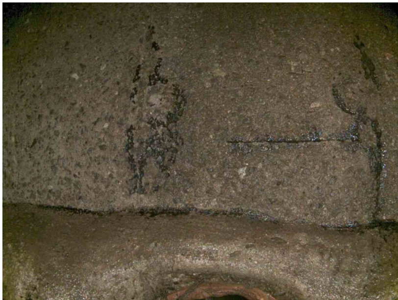
37-39_f9d93fbc_2737_41bc_8eac_424990064008_ea500f4d-0d86-4fbf-a0b9-599ee40e4332_P12.jpg, , 3.36 Surface Aggregate Visible from 12 o'clock to 12 o'clock, within 8 inch
