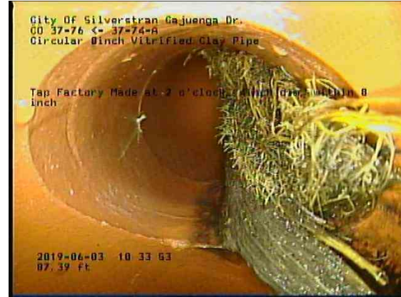
cd48e351-2f27-452f-9d63-9e3bd322b019_20190603_103629_456.jpg, 00:05:49, 87.39ft Tap Factory Made at 2 o'clock, 4inch dim, within 8 inch
