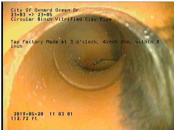
5d06406f-76d6-4ed6-8115-b2c406ad78b1_20190520_110531_124.jpg, 00:08:07, 112.72ft Tap Factory Made at 3 o'clock, 4inch dim, within 8 inch
