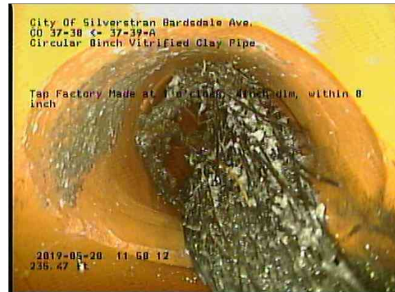
04242705-f072-4501-bc6c-3fd5184d2bb9_20190528_120046_741.jpg, 00:17:25, 235.47ft Tap Factory Made at 1 o'clock, 4inch dim, within 8 inch
