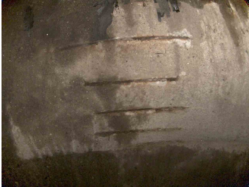
28-09_649da561_021a_4b6c_b8b5_5695380ff438_4699b76d-f272-4f57-a29f-4c5b9f8f7dc2_P12.jpg, , 2.65 Surface Reinforcement Corroded, from 04 to -01 o'clock, within 8 inch
