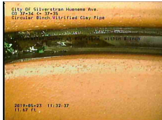
12664bd6-d339-4883-90b7-2acfe341bcfc_20190523_113510_867.jpg, 00:04:05, 11.67ft Infiltration Gusher at 9 o'clock, within 8 inch
