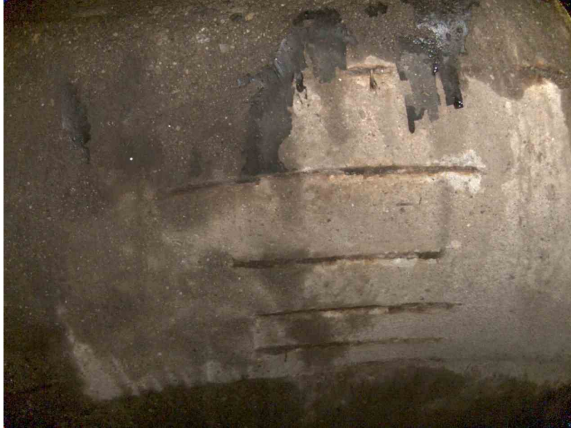
28-09_649da561_021a_4b6c_b8b5_5695380ff438_32a59c61-a6ba-4cd0-bd9a-85c83e97f5d5_P12.jpg, , 2.34 Surface Reinforcement Corroded, from 04 to -01 o'clock, within 8 inch
