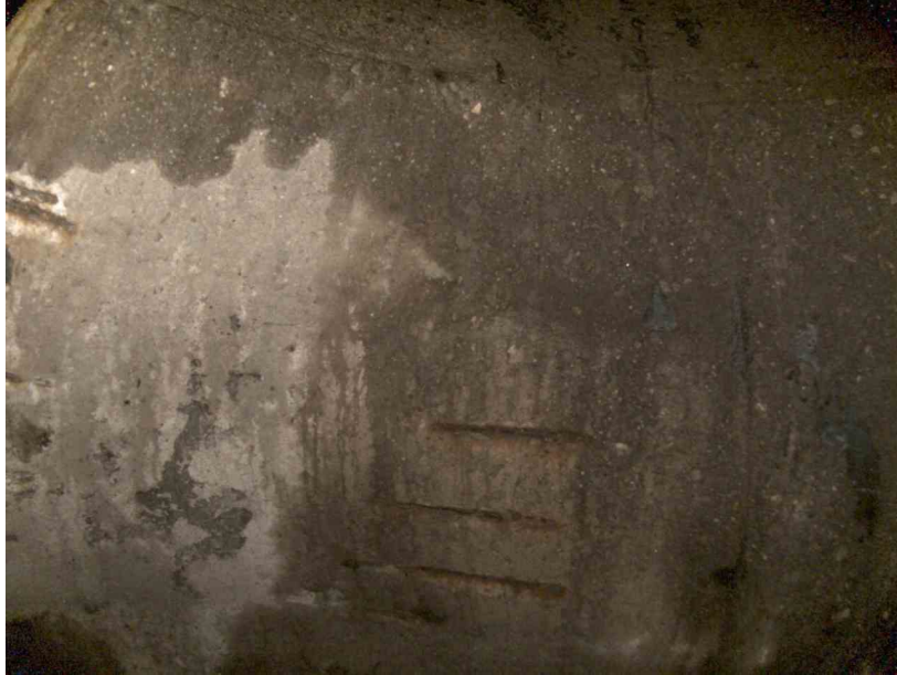
28-09_649da561_021a_4b6c_b8b5_5695380ff438_986d42a2-93a6-4e4d-99ca-49bd4ffbe2ba_P12.jpg, , 2.31 Surface Reinforcement Corroded, from 10 to -01 o'clock, within 8 inch
