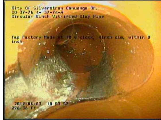
e0385131-657b-4c08-aefc-7dc0d1865d11_20190603_105633_929.jpg, 00:19:19, 296.35ft Tap Factory Made at 10 o'clock, 4inch dim, within 8 inch
