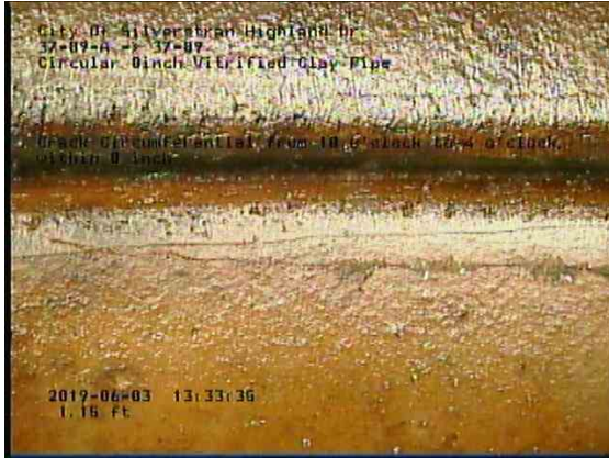
edf0fb5b-769a-41a7-aaff-f2b3f27946ea_20190603_133612_197.jpg, 00:01:43, 1.15ft Crack Circumferential from 10 o'clock to 4 o'clock, within 8 inch
