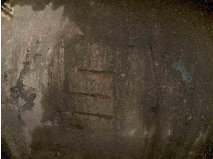
28-09_649da561_021a_4b6c_b8b5_5695380ff438_60335b05-d594-4c98-89f4-79bf729726fe_P12.jpg, , 2.66 Surface Reinforcement Corroded, from 10 to -01 o'clock, within 8 inch
