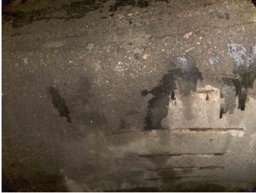
28-09_649da561_021a_4b6c_b8b5_5695380ff438_b885c202-bd32-45ca-881d-169679afd8a0_P12.jpg, , 1.96 Surface Reinforcement Corroded, from 04 to -01 o'clock, within 8 inch
