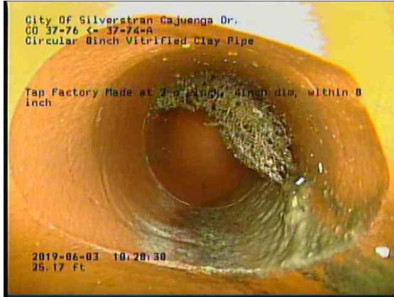
b358ac15-bcca-46ec-82bc-3ca9fcd9d9f5_20190603_103114_710.jpg, 00:01:46, 25.17ft Tap Factory Made at 2 o'clock, 4inch dim, within 8 inch
