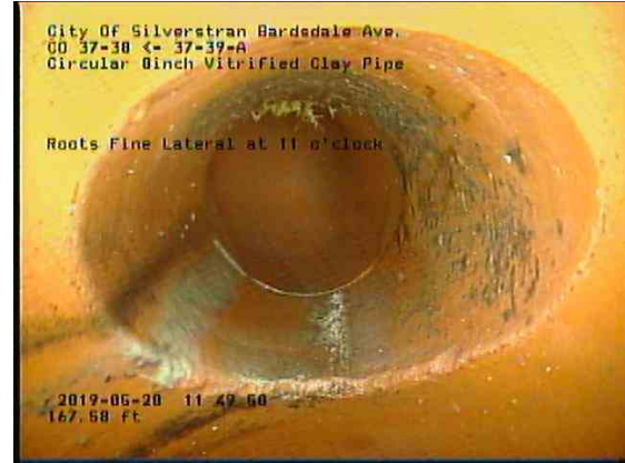
af2547a7-0f1c-4199-b9ee-8ae10e942bed_20190528_115232_503.jpg, 00:11:29, 167.58ft Roots Fine Lateral at 11 o'clock
