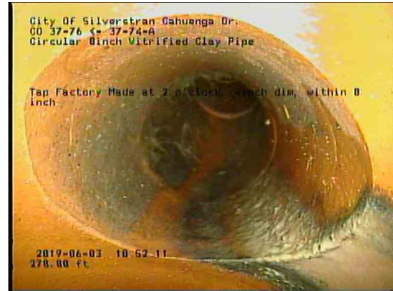
ee8c7d1a-0565-4658-9fbc-795e9b6d5469_20190603_105447_997.jpg, 00:18:24, 278.80ft Tap Factory Made at 2 o'clock, 4inch dim, within 8 inch
