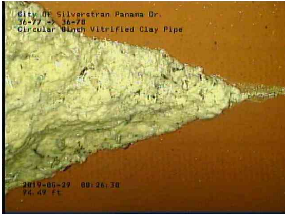
c7a79210-d0b3-4556-96ba-effe57e92479_20190529_082911_959.jpg, 00:11:50, 94.49ft Deposits Attached Encrustation, 5% of cross sectional area from 8 o'clock to 10 o'clock, within 8 inch
