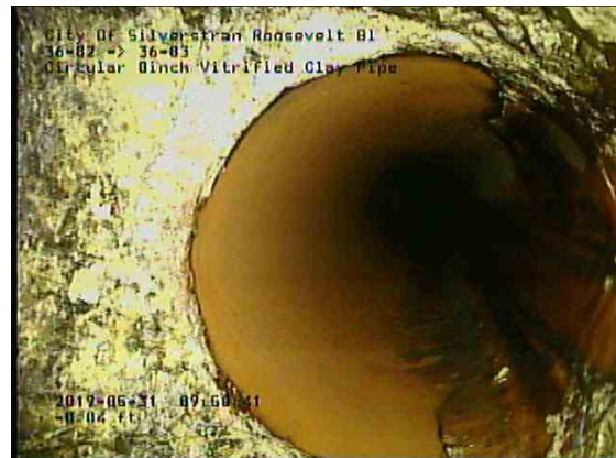
906f0a8e-8a63-4e61-af79-b1d5b69d21f0_20190531_100118_533.jpg, 00:00:50, 0.00ft Deposits Attached Encrustation, 5% of cross sectional area from 7 o'clock to 5 o'clock, within 8 inch
