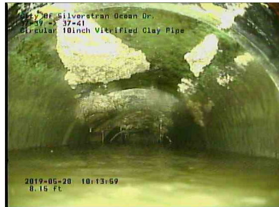
fb02755f-15c1-4357-83d7-11e3401a5e55_20190528_101632_520.jpg, 00:03:30, 7.39ft Water Level, Sag in pipe, 80% of the vertical dimension, Start
