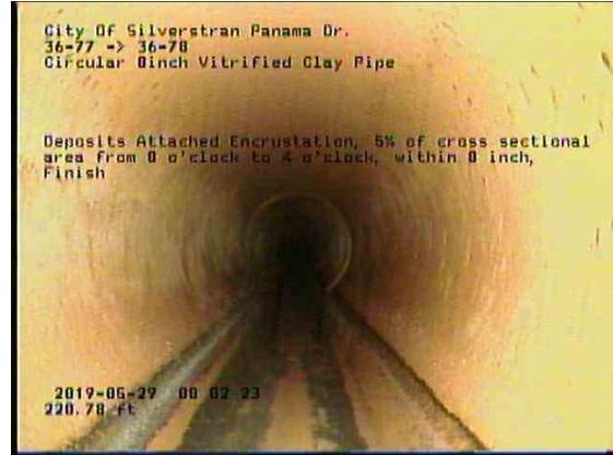
1997cd9d-df1b-455f-9dac-a87474e03574_20190529_080457_607.jpg, 00:19:19, 220.76ft Deposits Attached Encrustation, 5% of cross sectional area from 8 o'clock to 4 o'clock, within 8 inch, Finish
