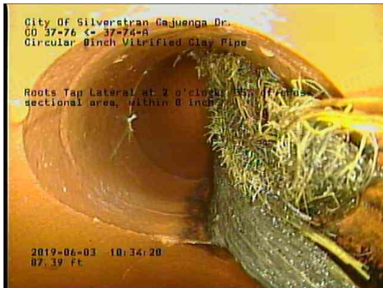
897cb046-dc93-4982-8d83-46616aa62916_20190603_103656_465.jpg, 00:05:53, 87.39ft Roots Tap Lateral at 2 o'clock, 35% of cross sectional area, within 8 inch
