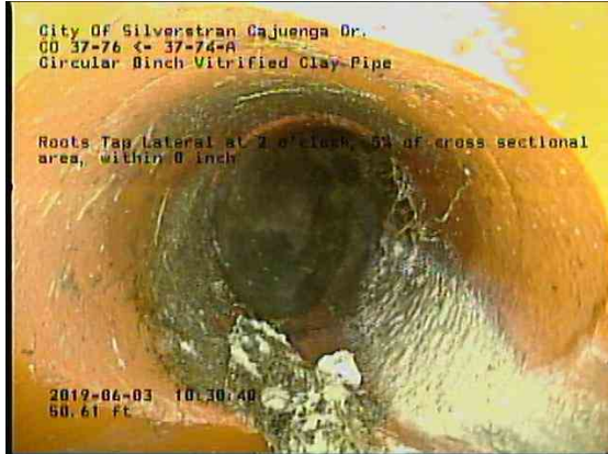
ef0dc867-8349-4191-90e4-c194659badfa_20190603_103324_807.jpg, 00:03:18, 50.61ft Roots Tap Lateral at 2 o'clock, 5% of cross sectional area, within 8 inch
