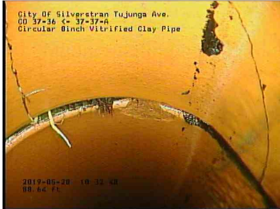
9be2a238-b5d2-4105-9618-2470546d9554_20190528_103521_938.jpg, 00:05:14, 88.66ft Fracture Longitudinal Hinge, 2 from 3 o'clock to 5 o'clock, within 8 inch
