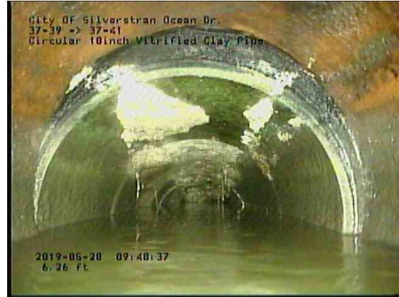
3c5be3a6-f13b-4589-9722-f87bba56286f_20190528_094310_398.jpg, 00:00:40, 7.39ft Joint Offset Large, 2Inch
