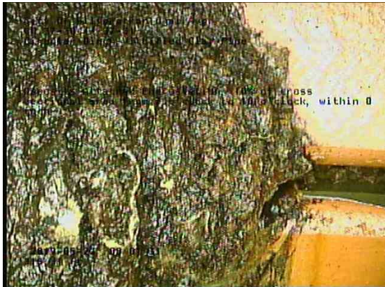
1bb14969-162a-4d38-a89d-1918eb3f2573_20190523_080403_778.jpg, 00:19:57, 315.31ft Deposits Attached Encrustation, 10% of cross sectional area from 7 o'clock to 10 o'clock, within 8 inch
