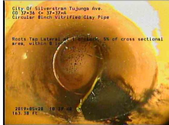
ec86239c-e105-4f02-a1b6-7bfc38d10381_20190528_104221_152.jpg, 00:09:50, 163.38ft Roots Tap Lateral at 1 o'clock, 5% of cross sectional area, within 8 inch
