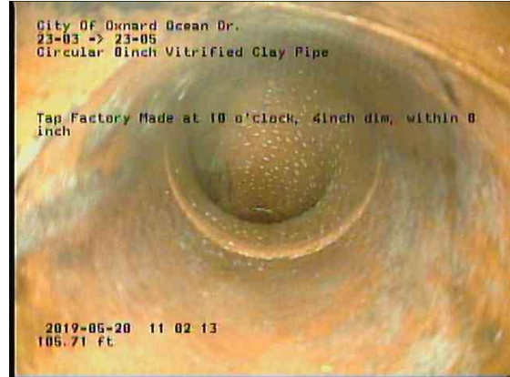
16b7fbe1-3ee7-4411-9623-ebda1aa7ffd8_20190520_110442_803.jpg, 00:07:30, 105.71ft Tap Factory Made at 10 o'clock, 4inch dim, within 8 inch
