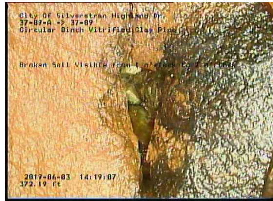
f5a9def0-c931-4199-b7a3-dfbfd53d71ca_20190603_142144_663.jpg, 00:33:29, 372.19ft Broken Soil Visible from 1 o'clock to 2 o'clock
