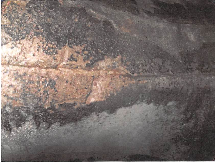
37-68_bc075bf7_3f28_485d_aaf8_7573fec9cbd6_ae7c9cc5-c9a6-4e8a-b4a1-aff349d573cc_PI2.jpg, , 1.53 Crack Longitudinal at 7 o'clock, within 8 inch
