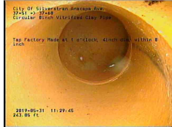
4b11f49b-30a6-4227-b989-64cec85a1339_20190531_113222_266.jpg, 00:14:17, 243.05ft Tap Factory Made at 1 o'clock, 4inch dim, within 8 inch
