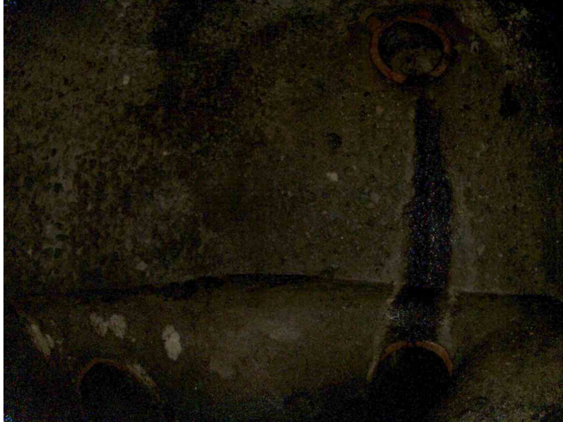
37-68_bc075bf7_3f28_485d_aaf8_7573fec9cbd6_cceabf30-0668-4f75-8b7e-afd5d7217628_PI2.jpg, , 7.64 Infiltration Stain at 8 o'clock, within 8 inch
