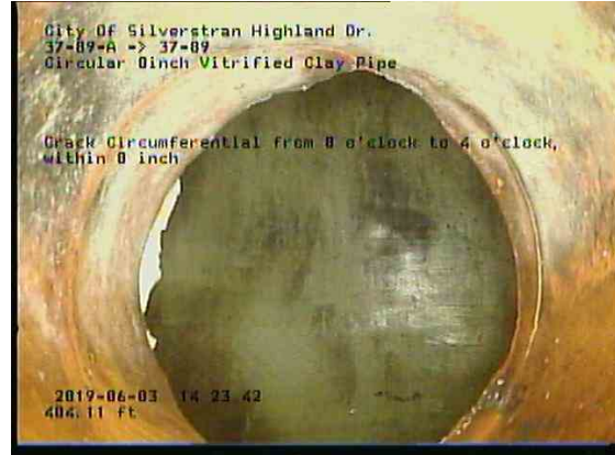
40a85798-0eb6-4633-8848-2e8488d9b2bb_20190603_142619_699.jpg, 00:36:38, 404.11ft Crack Circumferential from 8 o'clock to 4 o'clock, within 8 inch
