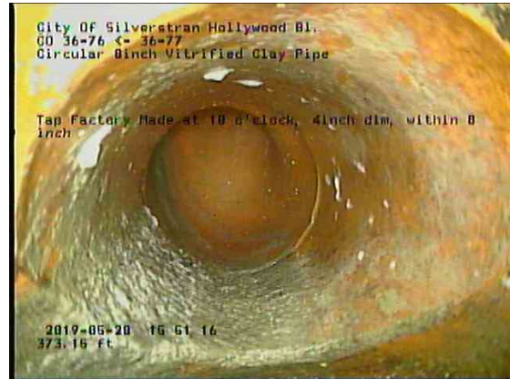
374ba6d9-05c8-4896-9ebe-ea843a6f9bf5_20190528_155350_557.jpg, 00:22:14, 373.15ft Tap Factory Made at 10 o'clock, 4inch dim, within 8 inch
