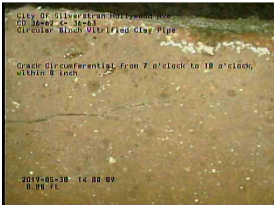
73a03eff-2e63-4612-adce-2efb35b314b4_20190530_141044_502.jpg, 00:00:57, 0.07ft Crack Circumferential from 7 o'clock to 10 o'clock, within 8 inch
