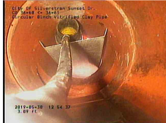
38027916-80dc-4828-ab27-92b8676eab07_20190530_125712_299.jpg, 00:01:32, 0.08ft Tap Factory Made at 6 o'clock, 8inch dim, within 8 inch
