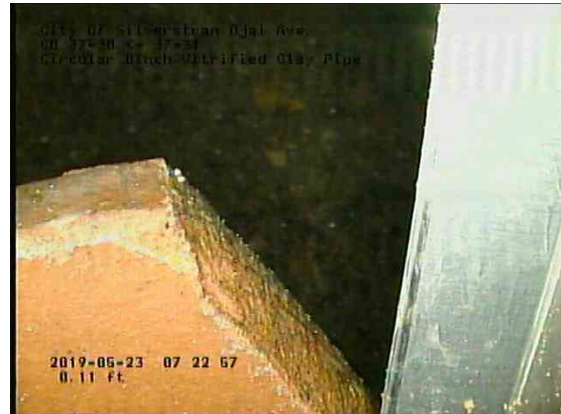
e3b4ddcc-d214-4d56-b4bc-23e1db9e1ae9_20190523_072529_604.jpg, 00:00:47, 0.11ft Broken from 11 o'clock to 4 o'clock
