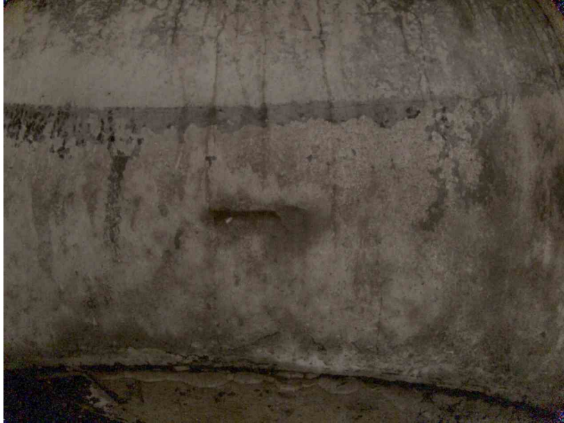
37-74-A_b7daeb13_42d1_4279_a6a1_58685002b84e_4a3c4159-085a-48c4-bf71-d41e9af6a294_P12.jpg, , 4.05 Surface Reinforcement Corroded at 9 o'clock, within 8 inch
