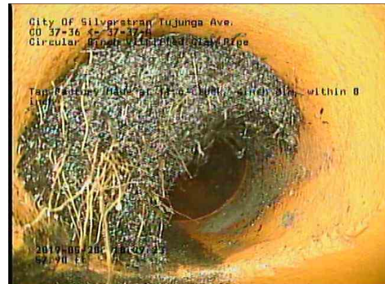
9c552e60-e346-4ca1-98ca-4fd3c9478eb6_20190528_103156_089.jpg, 00:03:01, 57.90ft Tap Factory Made at 11 o'clock, 4inch dim, within 8 inch
