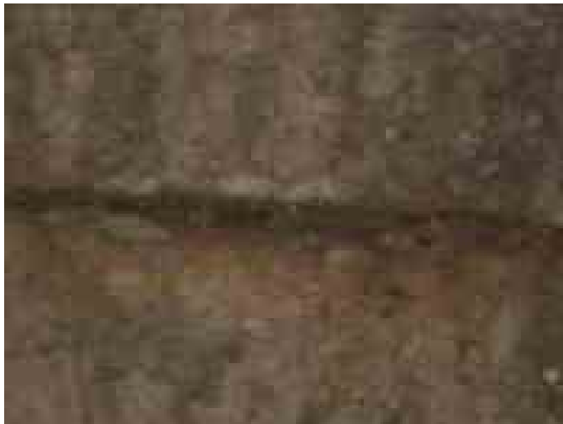
28-09_649da561_021a_4b6c_b8b5_5695380ff438_986d42a2-93a6-4e4d-99ca-49bd4ffbe2ba_P11.jpg, , 2.31 Surface Reinforcement Corroded, from 10 to -01 o'clock, within 8 inch
