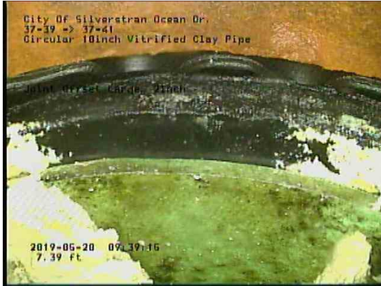
49952ff6-45e7-4139-b021-b5bdf2a08ee5_20190528_094148_817.jpg, 00:00:40, 7.39ft Joint Offset Large, 2Inch
