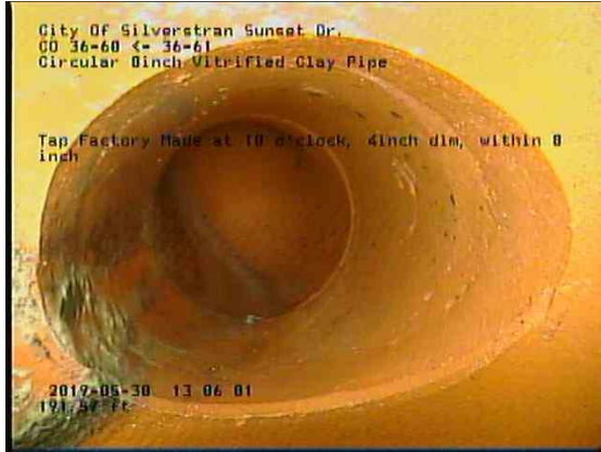
424c83ad-6daf-4e0a-a9a1-ebdc58e4a159_20190530_130836_773.jpg, 00:11:16, 191.57ft Tap Factory Made at 10 o'clock, 4inch dim, within 8 inch
