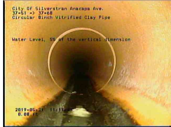
d2560a56-2bf6-4331-b681-fc3dfdfc2251_20190531_111422-629.jpg, 00:00:10, 0.00ft Water Level, 5% of the vertical dimension
