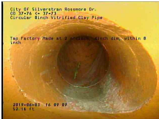
5c99c4cf-1168-4b0f-a84b-57452bfa0b4a_20190603_161146_700.jpg, 00:03:19, 52.16ft Tap Factory Made at 2 o'clock, 4inch dim, within 8 inch
