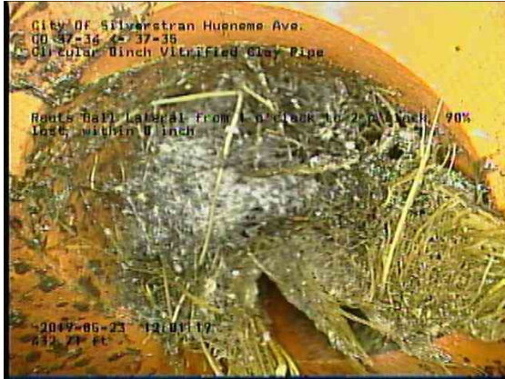
7829ffb5-79e0-46f0-8175-9fd23d2df5a7_20190523_120352_933.jpg, 00:27:58, 432.71ft Roots Ball Lateral from 1 o'clock to 2 o'clock, 90% lost, within 8 inch
