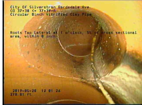
9a631e9d-057f-41ef-8ab5-2c0524cb7614_20190528_120358_288.jpg, 00:19:33, 270.80ft Roots Tap Lateral at 1 o'clock, 5% of cross sectional area, within 8 inch
