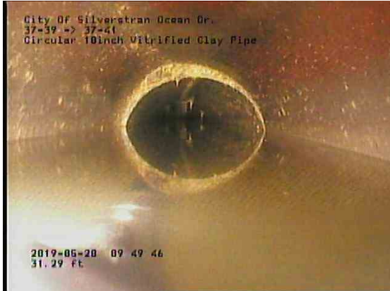
8d707d5b-fa0d-4b56-9fce-30d215b21bfe_20190528_095219_509.jpg, 00:03:34, 31.29ft Water Level, Sag in pipe, 80% of the vertical dimension, Finish
