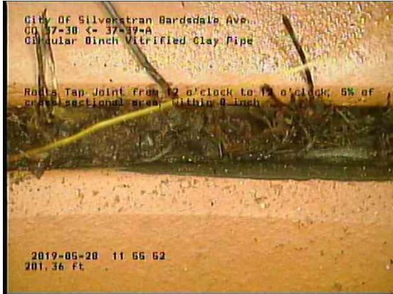
ea5472f0-b47e-4d87-9ee0-44bc60ee6adf_20190528_115826_161.jpg, 00:15:36, 201.36ft Roots Tap Joint from 12 o'clock to 12 o'clock, 5% of cross sectional area, within 8 inch
