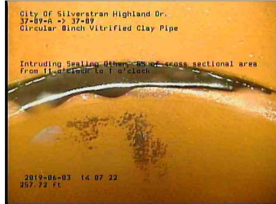
bfcddb54-d33b-415d-b7c6-55f892169652_20190603_140958_854.jpg, 00:23:43, 257.72ft Intruding Sealing Other, 5% of cross sectional area from 11 o'clock to 1 o'clock
