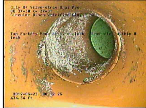
ebc1e46c-c373-44ab-9752-41f00f660847_20190523_081457_625.jpg, 00:27:55, 434.34ft Tap Factory Made at 12 o'clock, 8inch dim, within 8 inch
