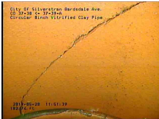
5fbb2c2d-f566-4395-b540-ec897655229e_20190528_115413_154.jpg, 00:12:50, 182.74ft Fracture Longitudinal Hinge, 3 from 3 o'clock to 7 o'clock, within 8 inch
