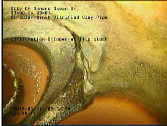
0c9758fa-0261-48fe-9281-c03aff41f3ab_20190521_093648_692.jpg, 00:18:13, 334.98ft Infiltration Dripper at 11 o'clock
