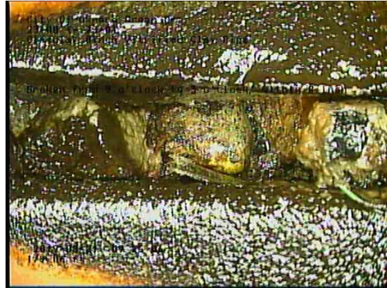
2bb4ce1d-f8e8-4d86-ae69-70fd15f010bb_20190521_092736_594.jpg, 00:10:08, 179.06ft Broken from 9 o'clock to 3 o'clock, within 8 inch
