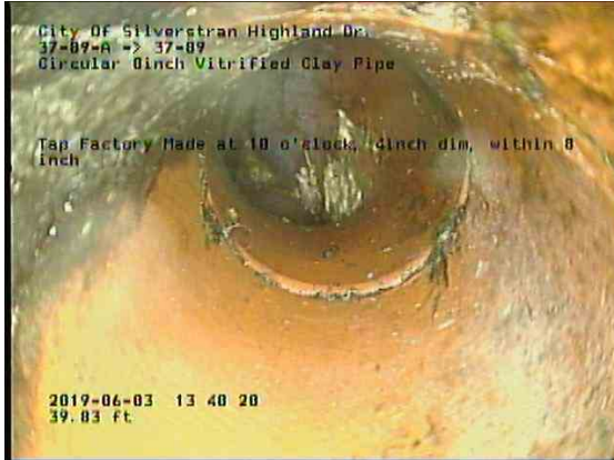
e58685e2-4258-4bdb-a720-a1d155ec0659_20190603_134257_017.jpg, 00:05:55, 39.83ft Tap Factory Made at 10 o'clock, 4inch dim, within 8 inch
