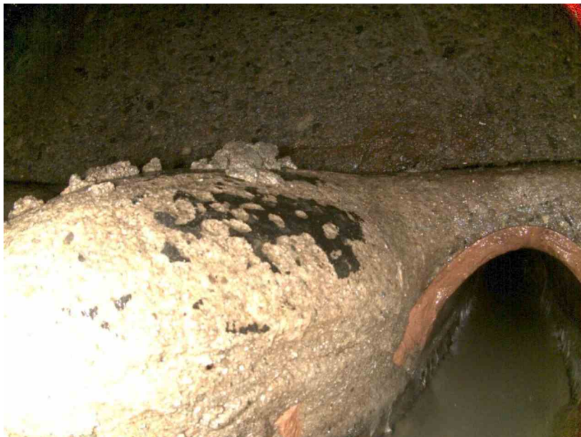
37-31_3a06f078_e941_4f01_ba58_04484b70b803_f16b28f4-f080-4b92-9262-280a38d67558_P12.jpg, , 8.16 Deposits Settled Compacted, 5% of cross sectional area at 10 o'clock, within 8 inch
