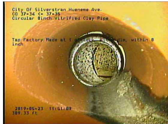
a27ed541-81a0-48a3-8bd2-5a04ab1163b2_20190523_11534_2_276.jpg, 00:19:42, 309.33ft Tap Factory Made at 1 o'clock, 4inch dim, within 8 inch
