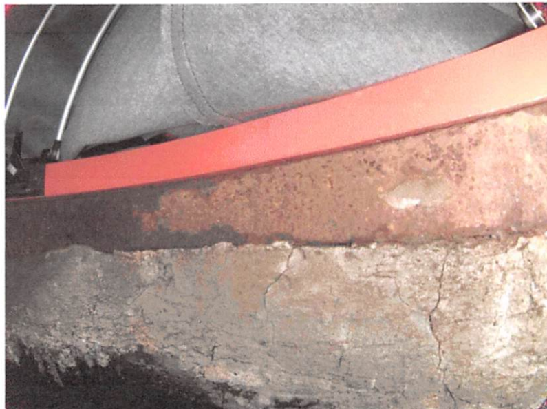
37-71_81c5c894_a2fd_4ca1_827e_284ab3133a40_07e7144f-d97b-4e5e-9e78-3df7b1b64efd_P12.jpg, , 0.20 Crack Longitudinal at 6 o'clock, within 8 inch
