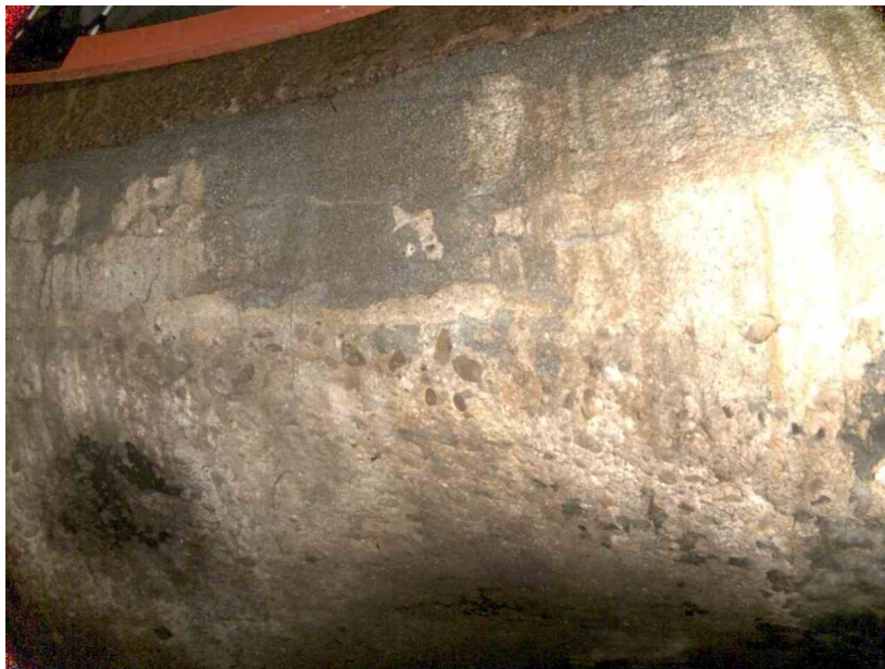
37-39_e3463806_251b_4a10_8598_66aa7b2b50ab_b61346a6-5cef-4041-8875-f7294a920564_P12.jpg, , 0.55 Surface Aggregate Visible from 12 o'clock to 12 o'clock, within 8 inch, Start
