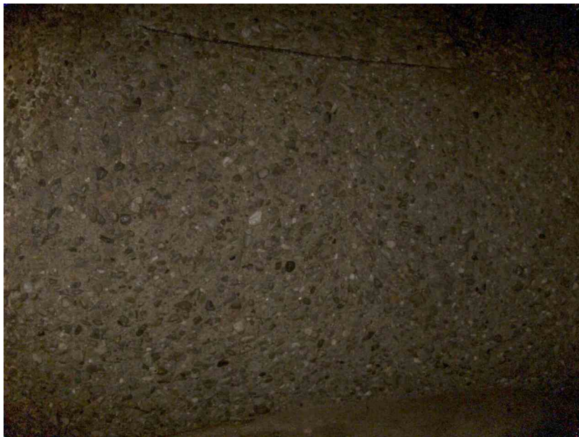
37-35_f6e7d8ee_4d76_46d5_86b4_5a5b78e4e34f_4fc0d4c6-111f-4509-8133-d17bd359c045_P12.jpg, , 7.57 Surface Aggregate Visible from 12 o'clock to 12 o'clock, within 8 inch
