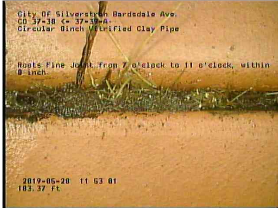
a3a9fb14-3f67-4fcf-b37c-be30c2bc9298_20190528_115534_124.jpg, 00:13:29, 183.37ft Roots Fine Joint from 7 o'clock to 11 o'clock, within 8 inch
