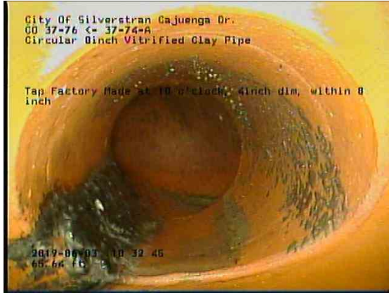
bf6ae7dc-816b-45fb-b69f-dda4aad3970c_20190603_103521_199.jpg, 00:04:49, 65.64ft Tap Factory Made at 10 o'clock, 4inch dim, within 8 inch
