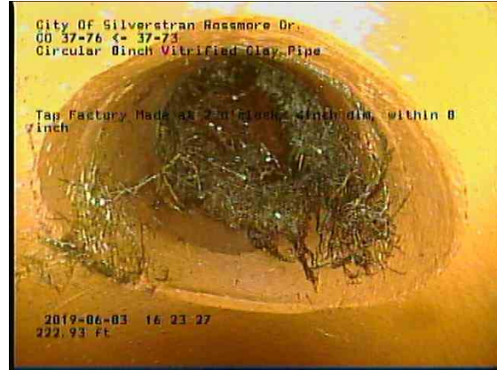
f966e9e2-ebba-47c4-9ef5-61336b9747dd_20190603_162604_559.jpg, 00:14:33, 222.93ft Tap Factory Made at 2 o'clock, 4inch dim, within 8 inch
