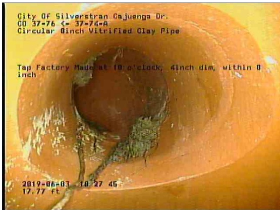
04981713-4c5d-4146-aafe-a17eabe72176_20190603_103021_217.jpg, 00:01:12, 17.77ft Tap Factory Made at 10 o'clock, 4inch dim, within 8 inch
