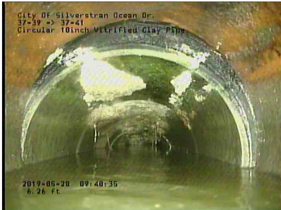
1bbe94cf-b143-43a1-8c70-e954676c53d7_20190528_094308_776.jpg, 00:00:47, 7.39ft Material Change, Polyvinyl chloride / 10"
