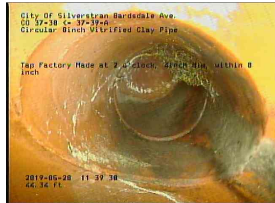
9b47a59e-54b9-439f-a96d-ca8f7e419be3_20190528_114204_519.jpg, 00:03:22, 44.34ft Tap Factory Made at 2 o'clock, 4inch dim, within 8 inch
