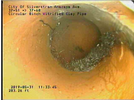
4588dfb1-cff6-433b-8e96-cae2402cf3ee_20190531_113621_880.jpg, 00:16:44, 283.30ft Tap Factory Made at 2 o'clock, 4inch dim, within 8 inch
