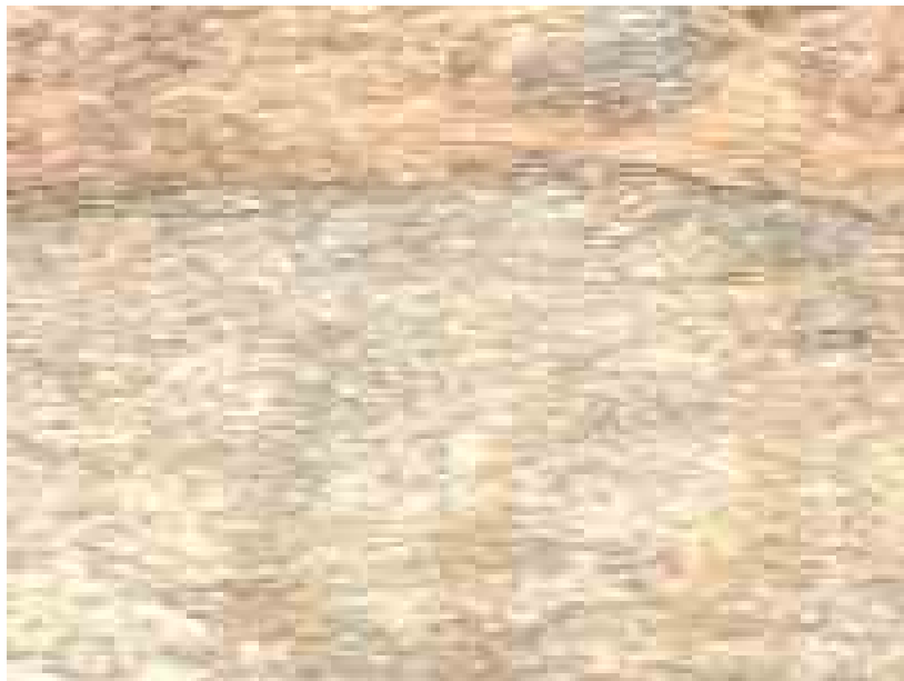
28-09_649da561_021a_4b6c_b8b5_5695380ff438_47b6dd48-897f-4927-b742-b77f48d8bb36_P11.jpg, , 0.03 Surface Roughness Increased, from 06 to -01 o'clock, within 8 inch, S01
