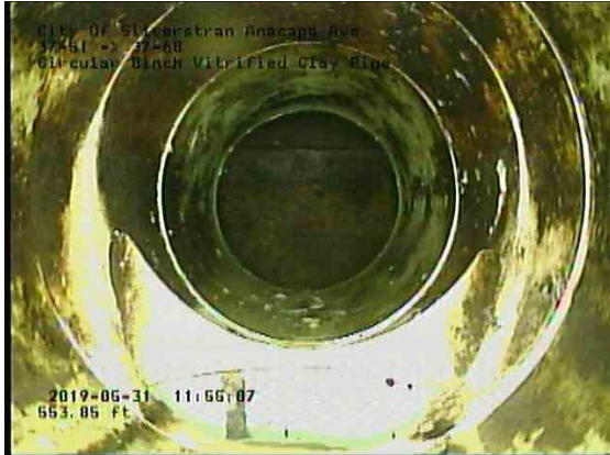
43191c15-e3ae-4259-bbdc-8fbef0137700_20190531_115744_211.jpg, 00:33:12, 554.43ft Tap Factory Made at 6 o'clock, 8inch dim, within 8 inch
