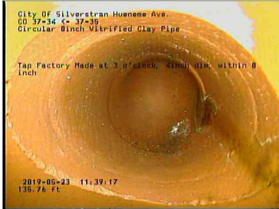
1e30851d-f53d-44e0-b837-0063eb7732fc_20190523_114150_178.jpg, 00:10:12, 135.76ft Tap Factory Made at 3 o'clock, 4inch dim, within 8 inch
