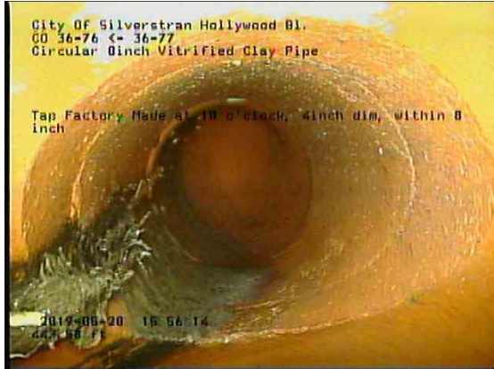
c31a10dd-315d-4f44-ac37-6b8434e1ebbc_20190528_155849_112.jpg, 00:26:18, 443.58ft Tap Factory Made at 10 o'clock, 4inch dim, within 8 inch
