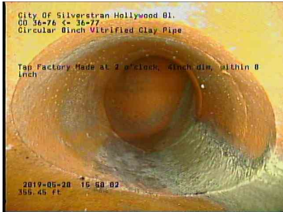
e35fb37f-9b8c-44f4-b2f5-107e5cef1bc7_20190528_155236_336.jpg, 00:21:08, 355.45ft Tap Factory Made at 2 o'clock, 4inch dim, within 8 inch
