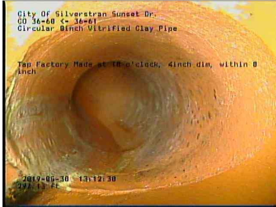
68e1f18c-450b-4c7a-b61e-9c211de127dd_20190530_131505_899.jpg, 00:16:36, 297.13ft Tap Factory Made at 10 o'clock, 4inch dim, within 8 inch
