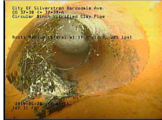
399cf8a7-3aab-4839-8713-60f2b48d8d94_20190528_114949_807.jpg, 00:09:23, 147.31ft Roots Medium Lateral at 11 o'clock, 20% lost
