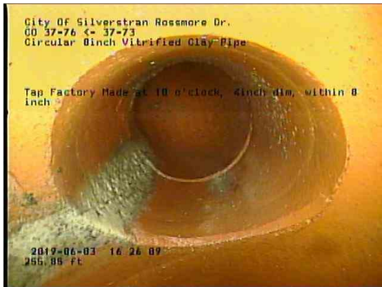
ec90d1c3-c99d-46d4-a973-bb67a6088908_20190603_162846_472.jpg, 00:16:29, 255.85ft Tap Factory Made at 10 o'clock, 4inch dim, within 8 inch
