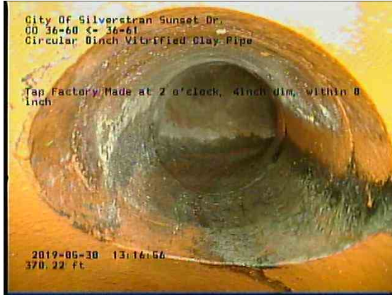
ef7bf8e6-520d-41a5-9dc7-8ce33b9fd540_20190530_131931_632.jpg, 00:20:29, 370.22ft Tap Factory Made at 2 o'clock, 4inch dim, within 8 inch
