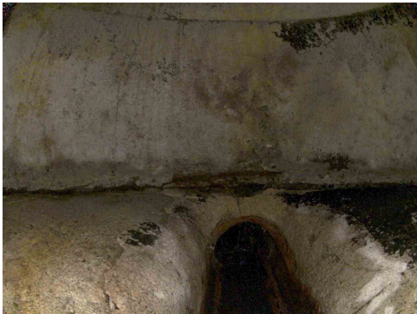
37-74-A_b7daeb13_42d1_4279_a6a1_58685002b84e_827eab20-93ee-45e4-9a82-80eed1922f70_P12.jpg, , 5.17 Surface Reinforcement Corroded at 6 o'clock, within 8 inch
