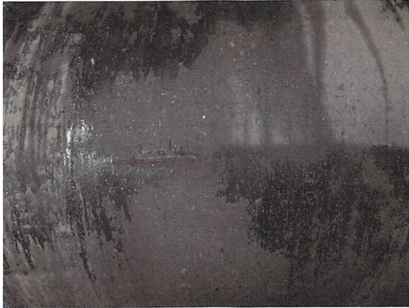
23-07_873817e9_0d4f_495f_ab7e_d928befa0923_7a8a0fdb-be91-4c87-8784-7edc0fca4c73_PI2.jpg, , 3.43 Surface Reinforcement Corroded at 1 o'clock, within 8 inch
