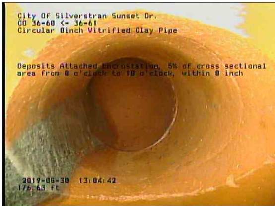
e57b2e32-95ac-4296-a464-931c75b63427_20190530_130717_807.jpg, 00:10:12, 176.63ft Deposits Attached Encrustation, 5% of cross sectional area from 8 o'clock to 10 o'clock, within 8 inch / IN WYE
