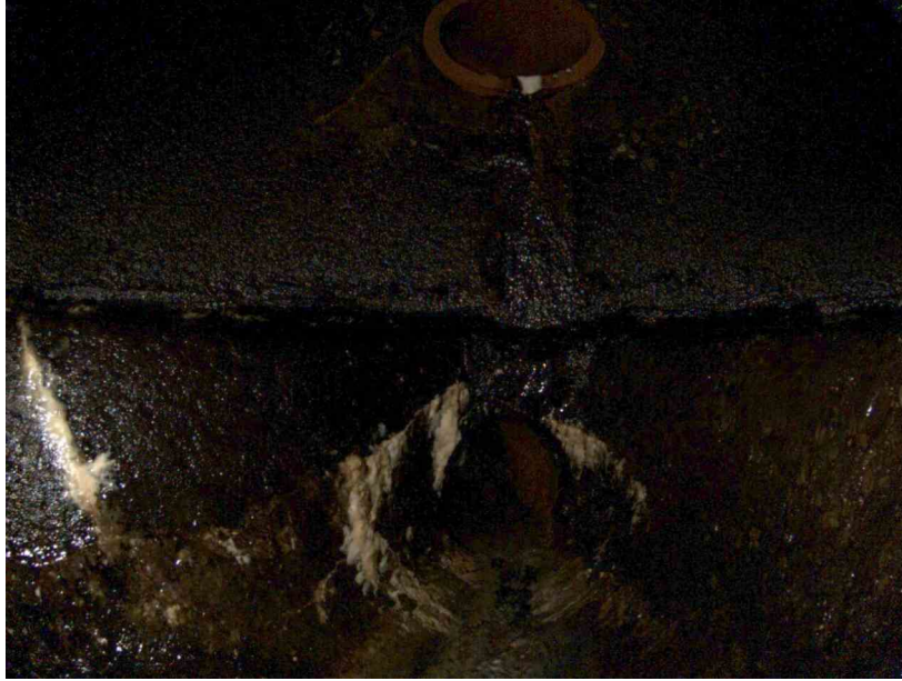
36-82_d8b17f0a_c20d_4a90_8fc5_f6b02c187456_924f9ada-9db4-4a2f-ac56-1a1e7f0c0f41_P12.jpg, , 8.03 Deposits Attached Grease, 5% of cross sectional area at 9 o'clock, within 8 inch
