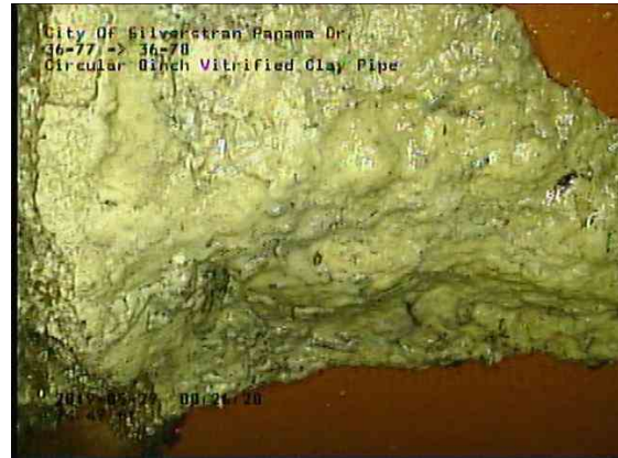
0b97f9bc-ffe8-40b8-b7e2-995c0a838d11_20190529_082902_907.jpg, 00:11:50, 94.49ft Deposits Attached Encrustation, 5% of cross sectional area from 8 o'clock to 10 o'clock, within 8 inch
