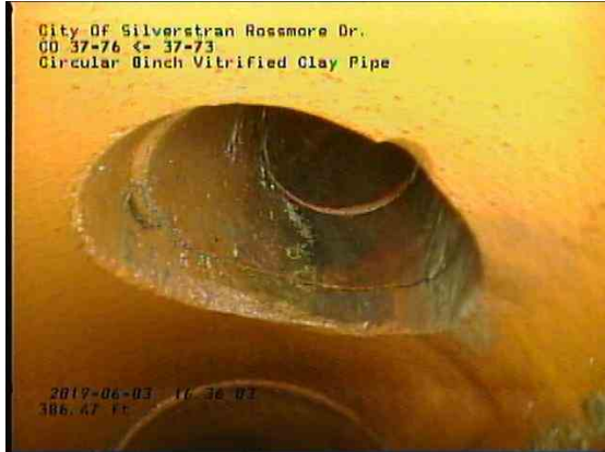
36a6c289-10c6-4e9f-afa8-91c082bb9e29_20190603_163840_613.jpg, 00:24:35, 386.68ft Fracture Circumferential from 3 o'clock to 4 o'clock, within 8 inch / IN WYE
