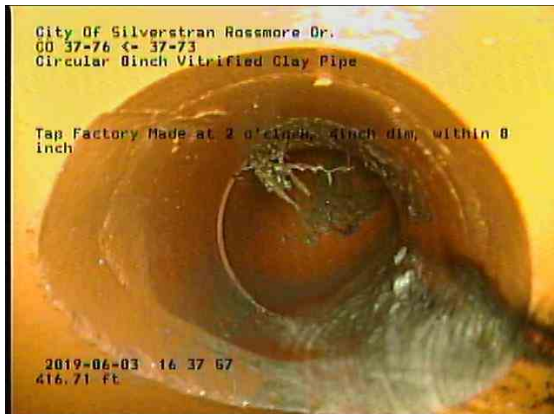
52d464fc-3dc6-4c15-a523-10a15f9b6661_20190603_164034_129.jpg, 00:26:24, 416.70ft Tap Factory Made at 2 o'clock, 4inch dim, within 8 inch
