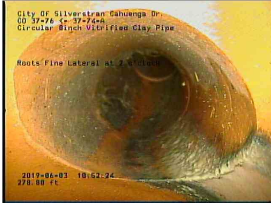
b38d1636-328f-4305-998d-e90c3b03cadf_20190603_105500_556.jpg, 00:18:27, 278.80ft Roots Fine Lateral at 2 o'clock
