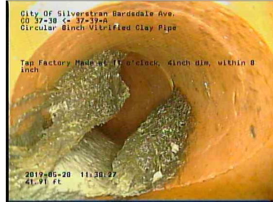
bab6791c-4651-4d3f-9592-7b2a82338ef3_20190528_114101_183.jpg, 00:02:44, 41.91ft Tap Factory Made at 11 o'clock, 4inch dim, within 8 inch
