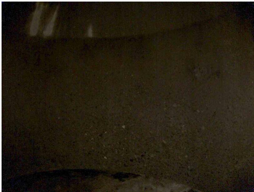
23-01_e8346f74_246f_46bb_9af3_39d1c680baea_69d3fab2-ef4b-479f-ade1-404eff70cf0c_P12.jpg, , 3.81 Surface Aggregate Visible from 4 o'clock to 7 o'clock, within 8 inch
