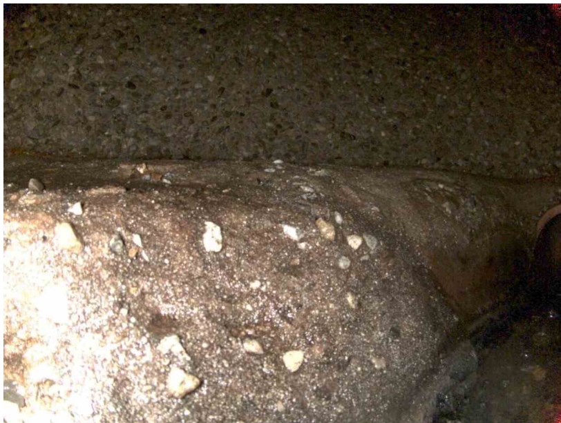
37-35_f6e7d8ee_4d76_46d5_86b4_5a5b78e4e34f_fb80f9fa-2a13-42aa-ac5b-944e72e13cb2_P12.jpg, , 9.69 Surface Aggregate Projecting at 10 o'clock, within 8 inch
