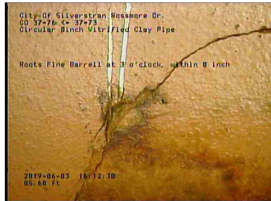
89620bc1-8bb7-4aa5-bcf8-23be6de01501_20190603_161507_533.jpg, 00:05:52, 85.68ft Roots Fine Barrell at 3 o'clock, within 8 inch
