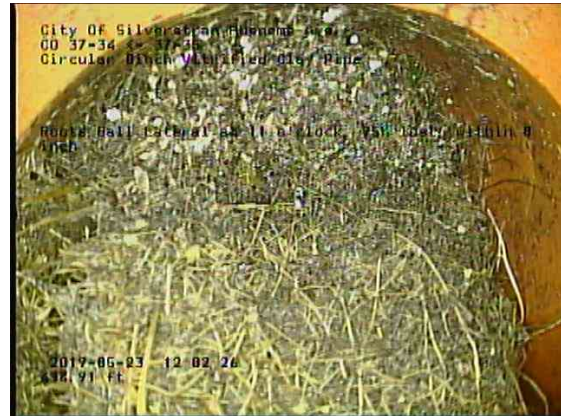
a36b0e93-865d-420a-8612-17099a6fc5b7_20190523_120459_774.jpg, 00:28:46, 434.91ft Roots Ball Lateral at 11 o'clock, 95% lost, within 8 inch
