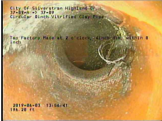
09e0ba0a-b8da-427c-9cdf-9fb34391e2b6_20190603_135917_901.jpg, 00:19:07, 196.20ft Tap Factory Made at 2 o'clock, 4inch dim, within 8 inch
