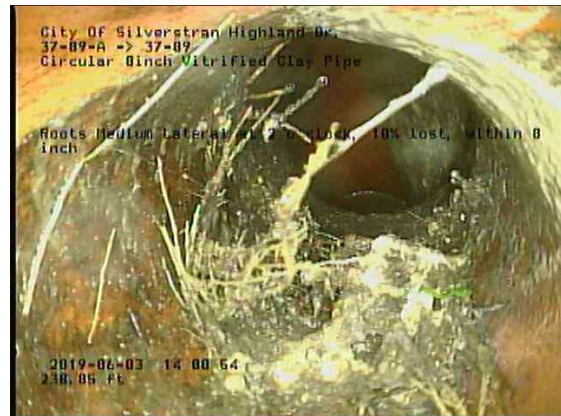
6259d6f3-37e6-467d-9819-cfeaff7831e9_20190603_140331_476.jpg, 00:22:18, 238.85ft Roots Medium Lateral at 2 o'clock, 10% lost, within 8 inch
