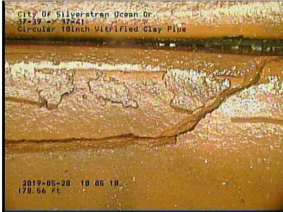
104e0d02-31bd-45f2-b78d-2558f8294249_20190528_100743_811.jpg, 00:10:54, 178.56ft Fracture Circumferential from 7 o'clock to 2 o'clock, within 8 inch
