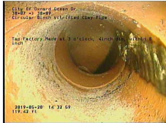
24b8cea6-aa09-4e2e-b0a5-d54fda156682_20190520_143529_593.jpg, 00:10:44, 119.42ft Tap Factory Made at 3 o'clock, 4inch dim, within 8 inch
