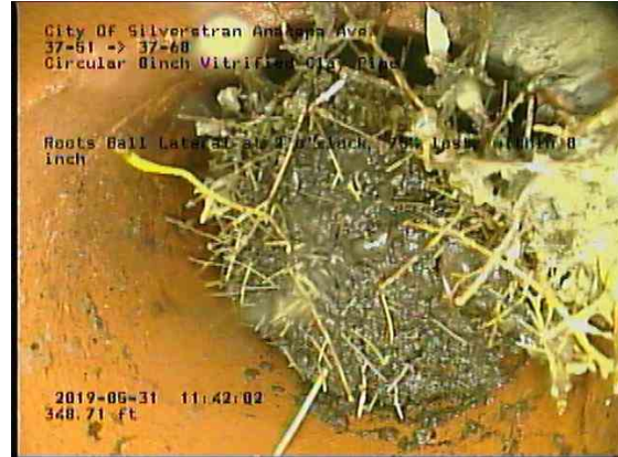
1bdb64c-4119-40c2-ad1c-6a0cc9f2d531_20190531_114438_398.jpg, 00:21:45, 348.71ft Roots Ball Lateral at 2 o'clock, 75% lost, within 8 inch
