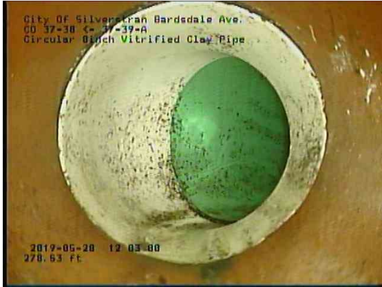
32feaf8-47df-4948-a2bf-19e7e478a03b_20190528_120534_290.jpg, 00:20:25, 278.92ft Material Change, Polyvinyl chloride / 8"
