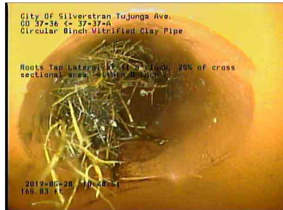
84292b92-7f95-4627-aeef-7b6b02bc3339_20190528_104324_330.jpg, 00:10:19, 165.83ft Roots Tap Lateral at 11 o'clock, 25% of cross sectional area, within 8 inch
