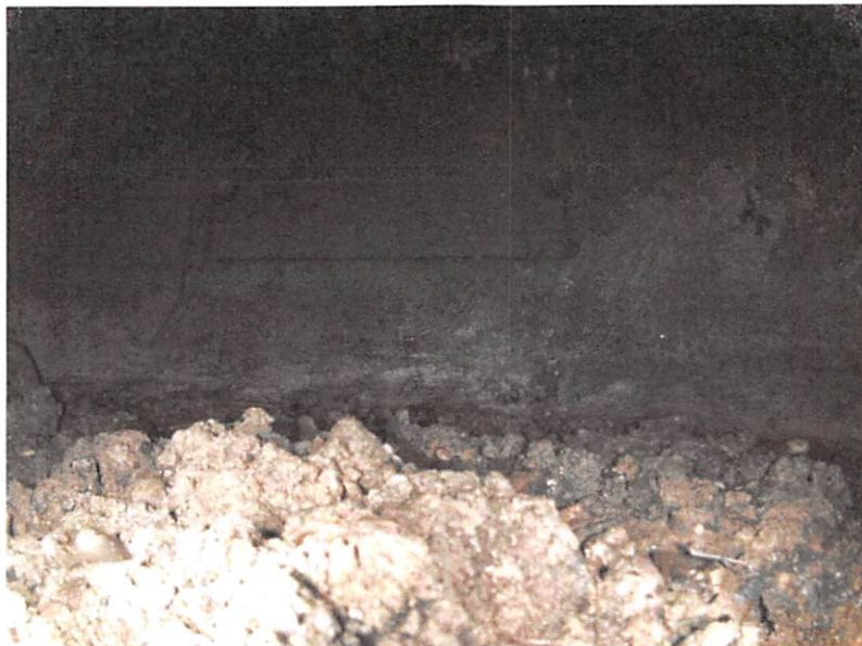
37-71_81c5c894_a2fd_4ca1_827e_284ab3133a40_43f0aef-34a1-4221-94f8-d52b50a16773_P12.jpg, , 7.82 Deposits Settled Compacted, 10% of cross sectional area from 12 o'clock to 5 o'clock, within 8 inch
