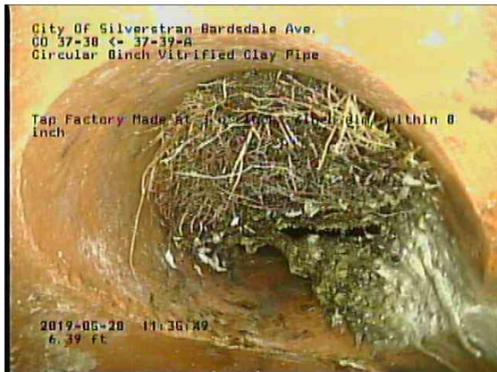
0c5f5e40-6f3d-40d1-a3f4-e6770482b3fa_20190528_113823_213.jpg, 00:00:36, 6.39ft Tap Factory Made at 3 o'clock, 4inch dim, within 8 inch
