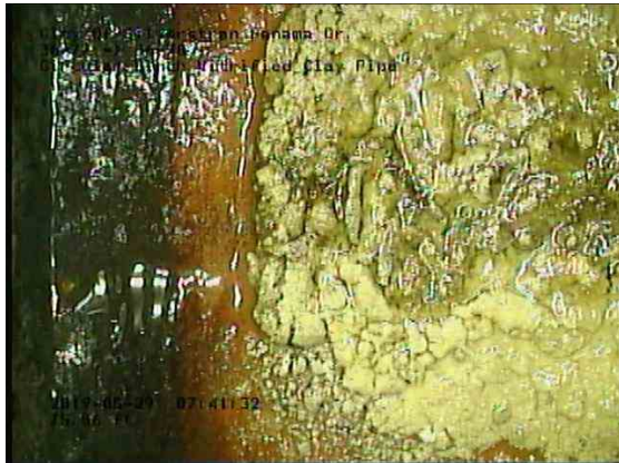
4cdf7aa3-03cc-466b-9f3e-5b9a2bbc8c2c_20190529_074405_960.jpg, 00:05:33, 75.56ft Infiltration Weeper from 7 o'clock to 5 o'clock, within 8 inch
