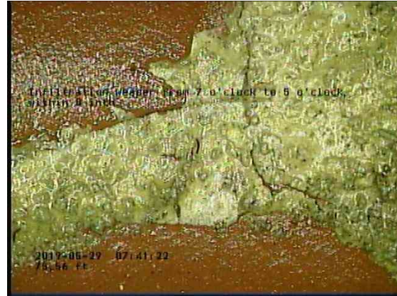
61a23f2c-324e-49f6-bdc4-736ec66fe6b6_20190529_074356_323.jpg, 00:05:33, 75.56ft Infiltration Weeper from 7 o'clock to 5 o'clock, within 8 inch
