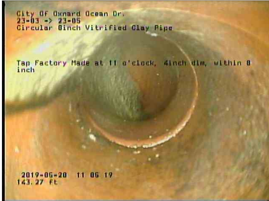
882ee781-8d25-467f-affa-6b82868e8d6f_20190520_110749_449.jpg, 00:10:10, 143.27ft Tap Factory Made at 11 o'clock, 4inch dim, within 8 inch
