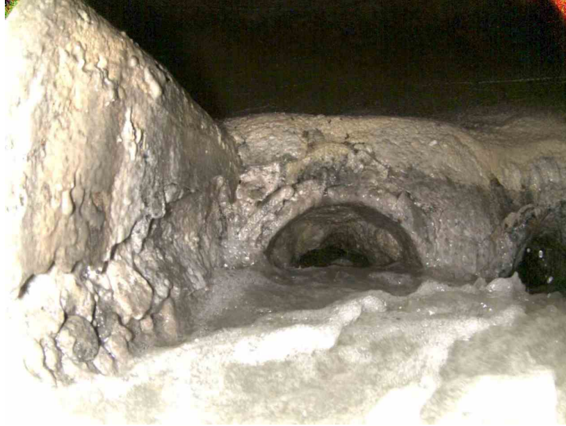
37-89_b7b73460_144a_4a36_a05d_2d26ddf59287_84ddab16-6324-489c-9c4c-349cbfa86c2d_P12.jpg, , 10.27 Lining Failure Delaminating at 3 o'clock, within 8 inch
