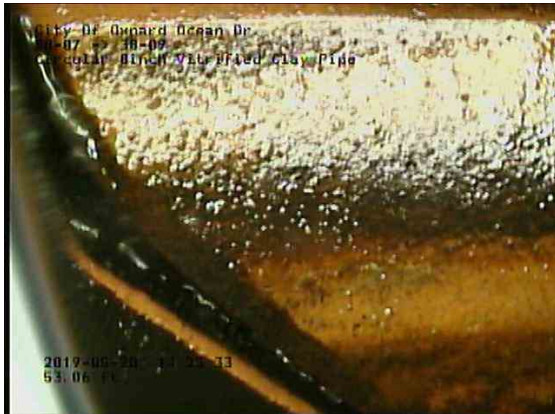
ba022e4c-6802-416f-ae30-1d9b4fa2b8d7_20190520_142803_380.jpg, 00:05:13, 52.86ft Broken from 11 o'clock to 3 o'clock, within 8 inch
