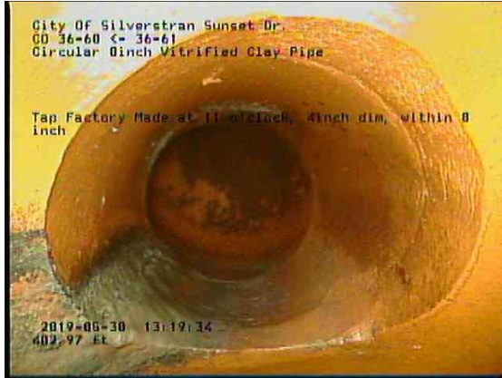
c432aa54-44c9-4112-9ca5-3a0c750a414d_20190530_132209_592.jpg, 00:22:29, 402.97ft Tap Factory Made at 11 o'clock, 4inch dim, within 8 inch
