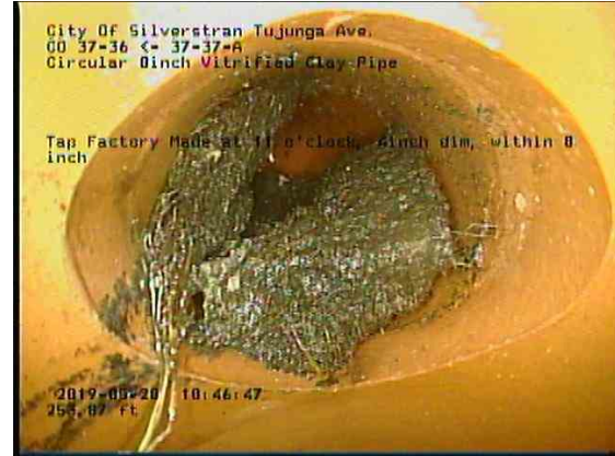
70465f0e-27f2-428d-a63b-6fd5a3f6aef6_20190528_104920_351.jpg, 00:15:07, 253.87ft Tap Factory Made at 11 o'clock, 4inch dim, within 8 inch
