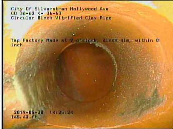
1ee4c2ae-9760-4b61-8060-10117052a714_20190530_142759_449.jpg, 00:11:15, 145.42ft Tap Factory Made at 9 o'clock, 4inch dim, within 8 inch
