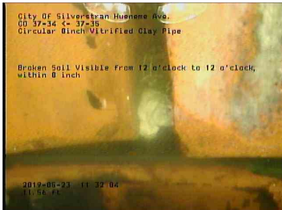
0d01e920-d0ea-44b2-8c45-753be36cb31f_20190523_113437_115.jpg, 00:03:41, 11.56ft Broken Soil Visible from 12 o'clock to 12 o'clock, within 8 inch
