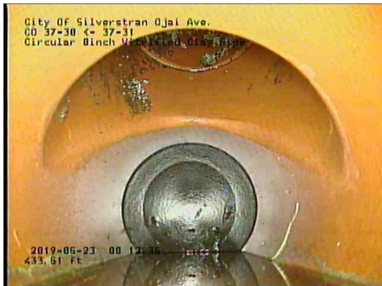
dc7344d8-8494-43d1-a906-9809744e9820_20190523_081507_663.jpg, 00:27:55, 434.34ft Tap Factory Made at 12 o'clock, 8inch dim, within 8 inch
