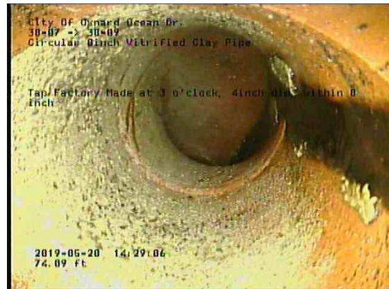
2c05cf76-8692-4207-beb3-526bd19c44b8_20190520_143136_339.jpg, 00:07:27, 74.09ft Tap Factory Made at 3 o'clock, 4inch dim, within 8 inch
