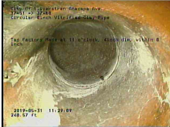
4d67c098-f890-4ec1-abd1-bb7cd8dbf5aa_20190531_113144_477.jpg, 00:13:49, 240.57ft Tap Factory Made at 11 o'clock, 4inch dim, within 8 inch
