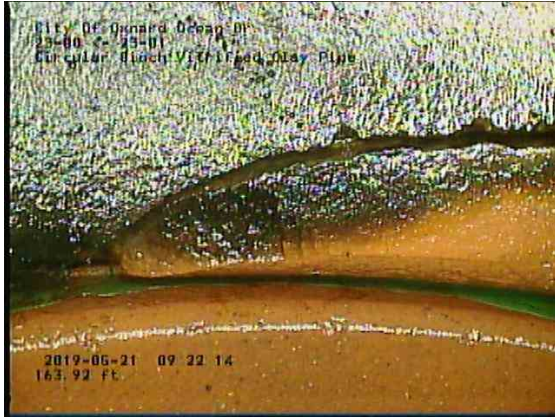
634d749e-f4a1-4147-9a3d-ceb9b47de711_20190521_092444_049.jpg, 00:07:48, 163.92ft Fracture Circumferential from 11 o'clock to 5 o'clock
