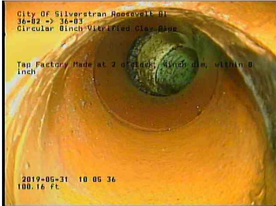
3cb780ba-5bee-4804-bcda-863503fe2368_20190531_100812_903.jpg, 00:07:22, 100.16ft Tap Factory Made at 2 o'clock, 4inch dim, within 8 inch
