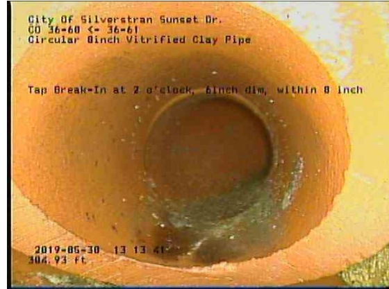
89a43f2e-f5be-4acd-a56b-c9d7a56ffa18_20190530_131616_176.jpg, 00:17:10, 304.92ft Tap Break-In at 2 o'clock, 6inch dim, within 8 inch
