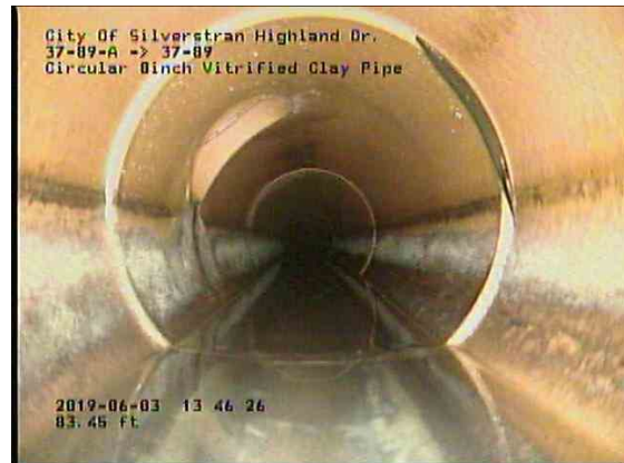
d8b9d150-4b31-4110-89c9-dfcc9fb613f4_20190603_134903_305.jpg, 00:10:07, 84.41ft Intruding Sealing Other, 5% of cross sectional area from 1 o'clock to 3 o'clock
