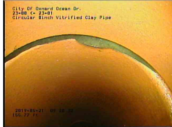
d980ef56-b9f3-4dc6-b2a2-8241ed6a36c0_20190521_092302_089.jpg, 00:06:29, 156.35ft Intruding Sealing Other, 5% of cross sectional area from 1 o'clock to 3 o'clock
