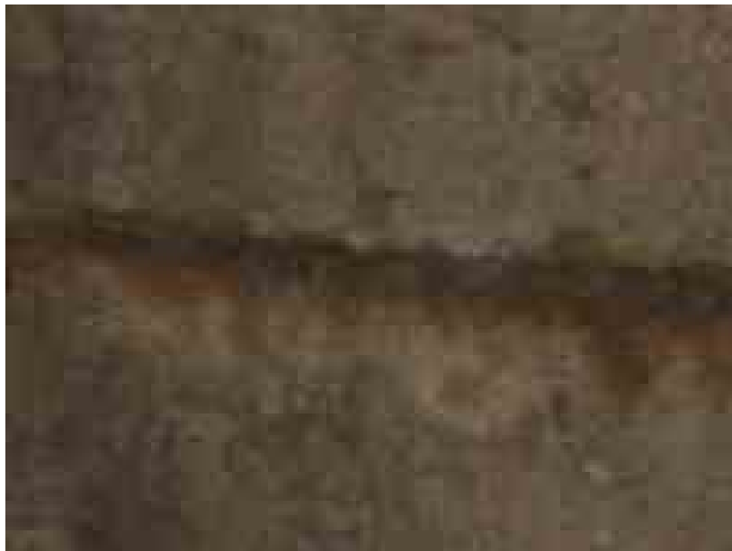
28-09_649da561_021a_4b6c_b8b5_5695380ff438_45944e11-9aa9-4c5e-8023-ea428999f8aa_P11.jpg, , 2.98 Surface Reinforcement Corroded, from 10 to -01 o'clock, within 8 inch
