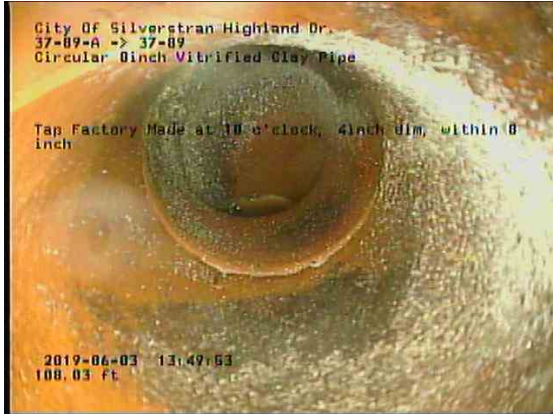
4b9310d7-16ae-48ef-b7d4-c1d7d6d12700_20190603_135230_283.jpg, 00:13:19, 108.03ft Tap Factory Made at 10 o'clock, 4inch dim, within 8 inch
