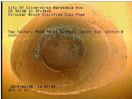
6e03a123-7879-454a-b88d-cffba252d0e8_20190528_120432_889.jpg, 00:20:01, 273.17ft Tap Factory Made at 11 o'clock, 4inch dim, within 8 inch
