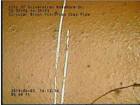
330f17cb-87f0-40ea-8235-c9a4900485c0_20190603_161511_200.jpg, 00:05:52, 85.68ft Roots Fine Barrell at 3 o'clock, within 8 inch
