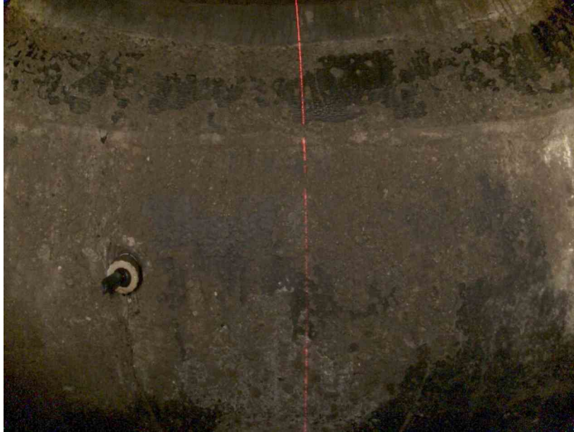
37-35_f6e7d8ee_4d76_46d5_86b4_5a5b78e4e34f_696fd2d6-6fb4-46b7-ab1f-98a80bae0cfd_P12.jpg, , 1.46 Obstacles Inuding Thru Wall, 5% of cross sectional area at 6 o'clock
