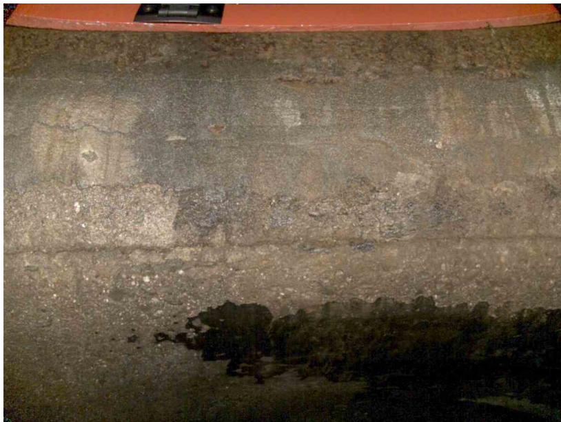
37-39_f9d93fbc_2737_41bc_8eac_424990064008_f393c6e6-6eff-49c5-9bb6-b3b7fc70a67f_P12.jpg, , 0.47 Surface Roughness Increased from 12 o'clock to 12 o'clock, within 8 inch, Start
