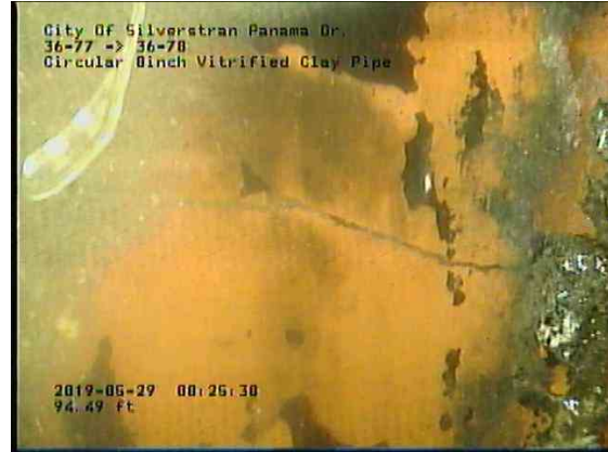
5ed87e68-3de8-41a8-92f4-9dd68939ecd5_20190529_082812_620.jpg, 00:11:37, 94.49ft Fracture Multiple from 2 o'clock to 10 o'clock, within 8 inch
