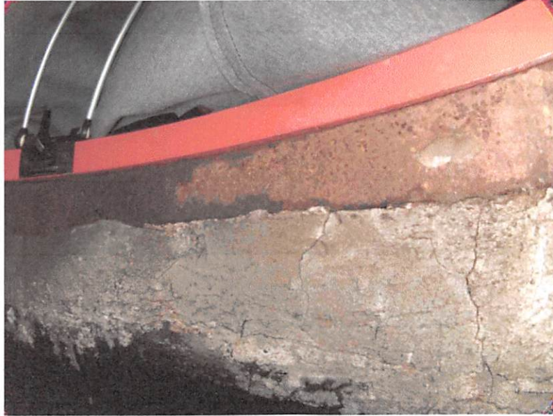
37-71_81c5c894_a2fd_4ca1_827e_284ab3133a40_6dfab672-5437-488e-b413-6ace9a40e13c_P12.jpg, , 0.28 Crack Longitudinal at 7 o'clock, within 8 inch
