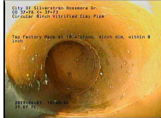
19bf312f-ebad-4236-9b11-4c13e384472c_20190603_161043_458.jpg, 00:02:22, 29.67ft Tap Factory Made at 10 o'clock, 4inch dim, within 8 inch
