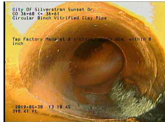
352f10b8-f068-4de8-a2c1-b90e60954155_20190530_132120_328.jpg, 00:21:48, 390.41ft Tap Factory Made at 2 o'clock, 4inch dim, within 8 inch
