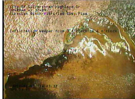
896d2223-6a1b-448b-ae70-0b7c4b920d3c_20190603_141613_953.jpg, 00:29:25, 362.75ft Infiltration Weeper from 3 o'clock to 4 o'clock
