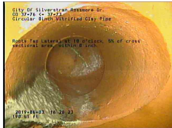
0b5e973d-6883-4861-aa0a-505685837ec7_20190603_162301_063.jpg, 00:12:16, 190.51ft Roots Tap Lateral at 10 o'clock, 5% of cross sectional area, within 8 inch
