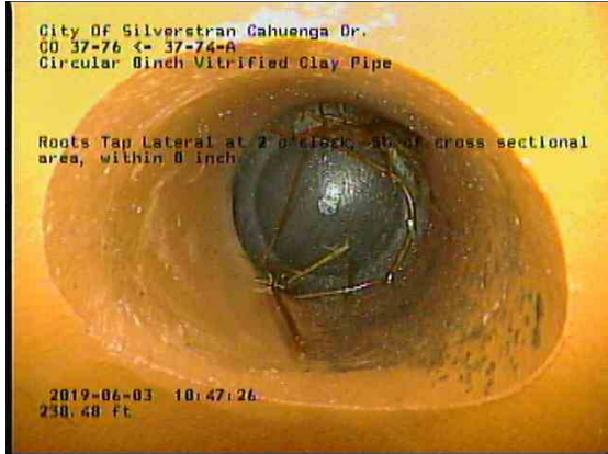
cb366758-9a99-4112-aba2-a3040b02d116_20190603_105002_862.jpg, 00:15:36, 238.48ft Roots Tap Lateral at 2 o'clock, 5% of cross sectional area, within 8 inch
