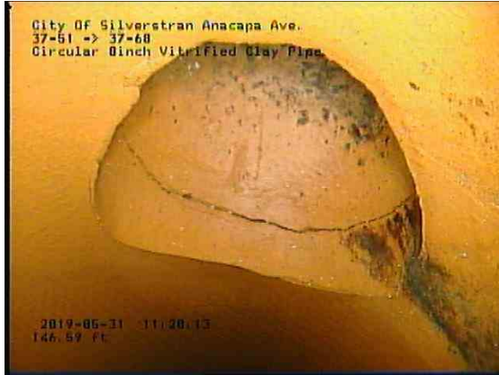
4c7017c8-6192-40b2-9179-d39396bacc99_20190531_112250_641.jpg, 00:07:24, 146.97ft Crack Circumferential from 12 o'clock to 12 o'clock, within 8 inch / In WYE
