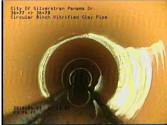
4665dd3d-e685-448a-9a31-03c746b90b6a_20190529_074441_311.jpg, 00:04:52, 74.91ft Deposits Attached Encrustation, 5% of cross sectional area at 2 o'clock, within 8 inch
