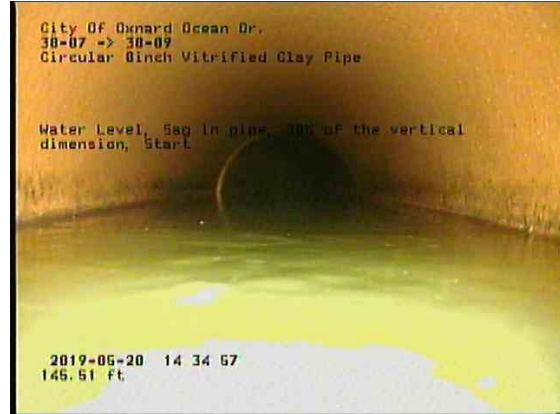
1165d41a-0333-4249-b410-8fcd84b312f5_20190520_143727_118.jpg, 00:12:21, 145.51ft Water Level, Sag in pipe, 30% of the vertical dimension, Start
