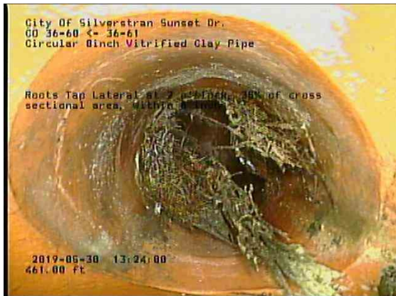
d65b8640-213e-42e9-b830-ac8a71c9d507_20190530_132635_755.jpg, 00:25:26, 460.99ft Roots Tap Lateral at 2 o'clock, 35% of cross sectional area, within 8 inch
