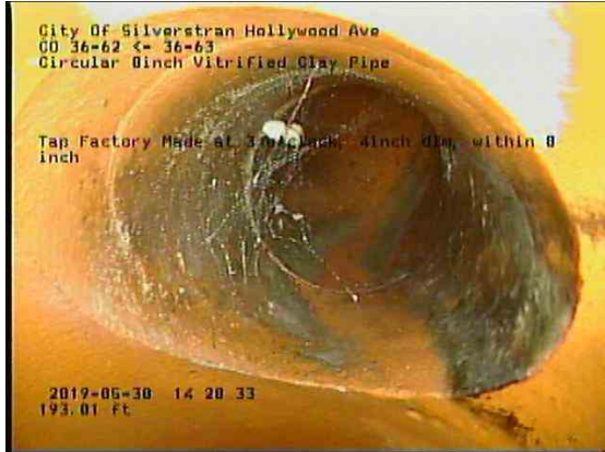
02c626d6-1a4c-4120-a74c-d833bc2756a3_20190530_143108_689.jpg, 00:13:54, 193.00ft Tap Factory Made at 3 o'clock, 4inch dim, within 8 inch
