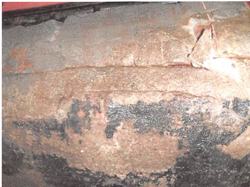
23-07_873817e9_0d4f_495f_ab7e_d928befa0923_6258d4fc-67de-42ed-a17c-88fb8a8373f8_PI2.jpg, , 0.49 Crack Circumferential from 12 o'clock to 12 o'clock, within 8 inch
