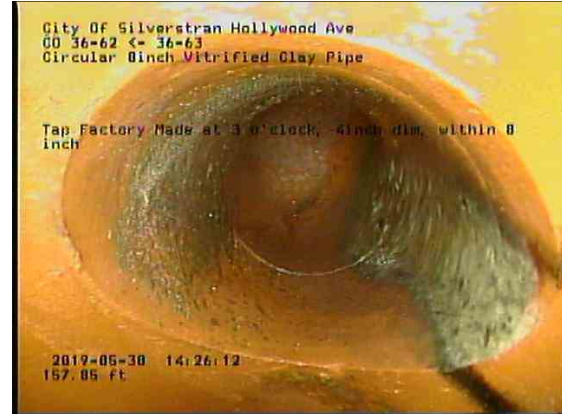
2aa00e97-f7ba-4cd2-8a7f-e41df4f4a765_20190530_142848_004.jpg, 00:11:57, 157.85ft Tap Factory Made at 3 o'clock, 4inch dim, within 8 inch
