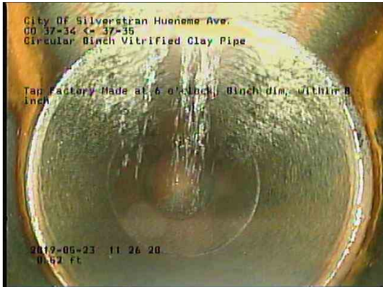
0d303b1c-7bb0-468b-ba69-2cd41a30b866_20190523_112853_785.jpg, 00:00:56, 0.52ft Tap Factory Made at 6 o'clock, 8inch dim, within 8 inch
