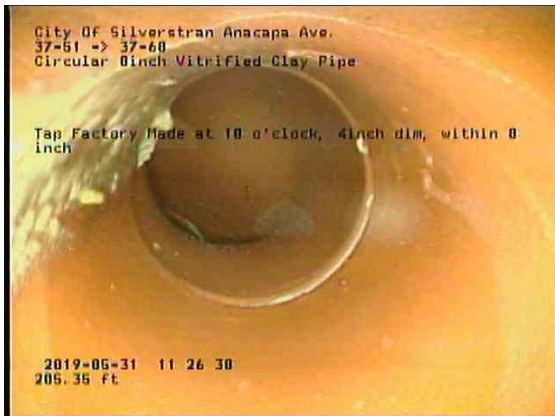
405c5b4c-e50d-44de-aa8a-60af7b1df44c_20190531_112915_506.jpg, 00:11:36, 205.35ft Tap Factory Made at 10 o'clock, 4inch dim, within 8 inch
