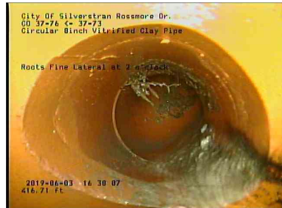
c481ad72-c24e-4470-8e91-c7cec95ec617_20190603_16404_4_129.jpg, 00:26:27, 416.71ft Roots Fine Lateral at 2 o'clock
