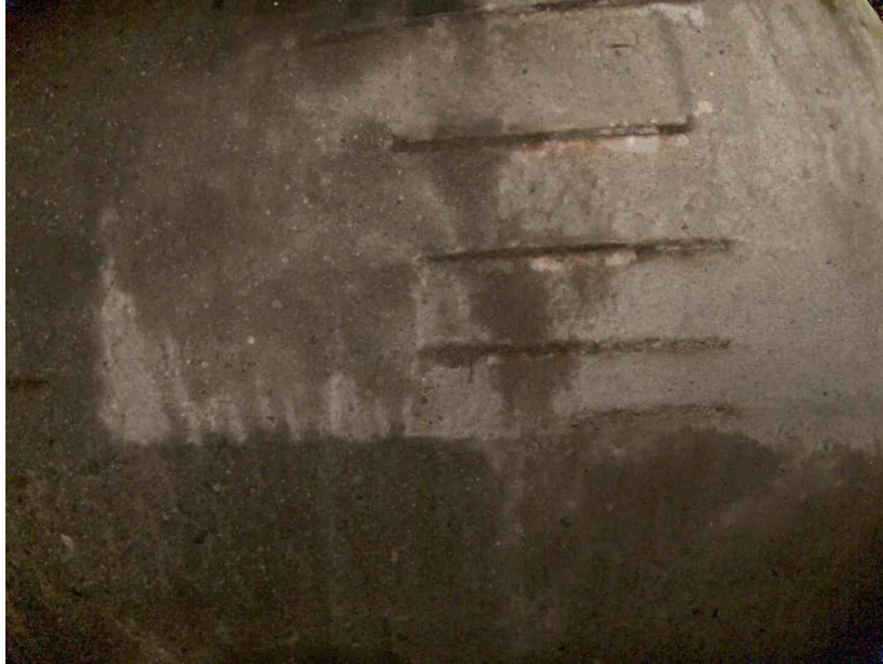
28-09_649da561_021a_4b6c_b8b5_5695380ff438_bbc57b83-8037-4a5b-8b09-f94d6c96ff7a_P12.jpg, , 3.01 Surface Reinforcement Corroded, from 04 to -01 o'clock, within 8 inch
