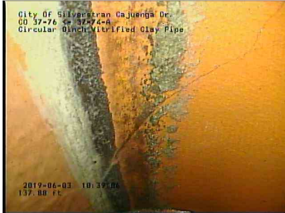
073784f6-6699-421a-a784-460ed8973ac9_20190603_104142_069.jpg, 00:09:33, 137.88ft Crack Spiral from 6 o'clock to 11 o'clock, within 8 inch
