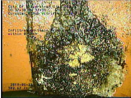
b0ca37ea-b18a-432c-bef0-22dd48451740_20190523_080219_896.jpg, 00:18:35, 302.67ft Infiltration Stain from 4 o'clock to 5 o'clock, within 8 inch
