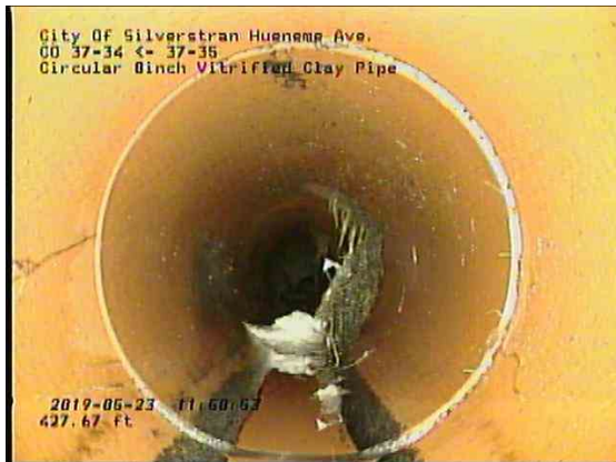
f827b99f-57c6-4ea9-ad3a-2477adec4a65_20190523_120126_680.jpg, 00:26:16, 428.65ft Roots Fine Joint from 7 o'clock to 5 o'clock, within 8 inch
