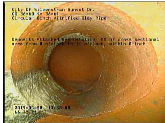
1ba4d1aa-a92a-4d47-bb71-2510bf3b0234_20190530_130043_945.jpg, 00:04:54, 66.33ft Deposits Attached Encrustation, 5% of cross sectional area from 8 o'clock to 11 o'clock, within 8 inch / IN WYE
