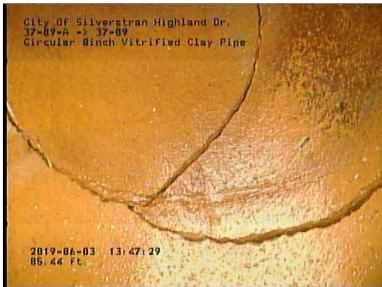
7eb37d75-d6f1-41fd-8885-8507d4219ef3_20190603_135006_683.jpg, 00:10:56, 85.58ft Fracture Multiple from 12 o'clock to 12 o'clock, within 8 inch / IN WYE
