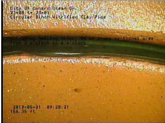
c2b5bf38-c8d5-4e14-98b7-31a41093fde7_20190521_092251_614.jpg, 00:06:29, 156.35ft Intruding Sealing Other, 5% of cross sectional area from 1 o'clock to 3 o'clock
