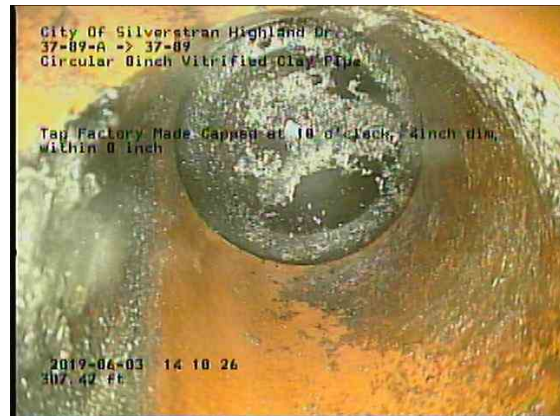
555f5110-bdf7-48fe-8f85-b3e077d1cf60_20190603_141303_681.jpg, 00:26:32, 307.42ft Tap Factory Made Capped at 10 o'clock, 4inch dim, within 8 inch
