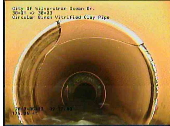
2d6522c3-87ec-45d4-89ea-bc6ff8015d59_20190522_092931_478.jpg, 00:11:15, 176.27ft Fracture Multiple from 7 o'clock to 2 o'clock, within 8 inch
