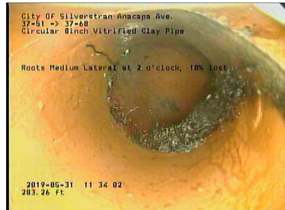
7b4c0d57-5792-4b98-8b35-ce304d3eaa26_20190531_113639_707.jpg, 00:17:10, 283.26ft Roots Medium Lateral at 2 o'clock, 10% lost
