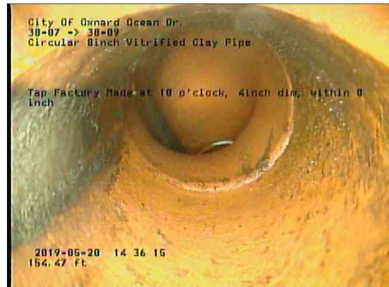
691a3ce2-aa85-41ec-836e-ee402ad76596_20190520_143845_032.jpg, 00:13:23, 154.47ft Tap Factory Made at 10 o'clock, 4inch dim, within 8 inch
