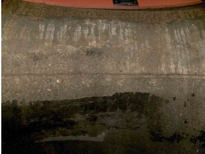
37-39_f9d93fbc_2737_41bc_8eac_424990064008_7cfdb3ba-bc5f-4c17-b98b-5c27e4a9cb64_P12.jpg, , 0.53 Crack Circumferential from 12 o'clock to 12 o'clock, within 8 inch
