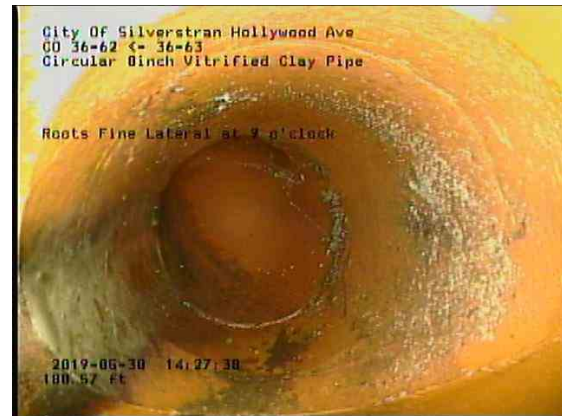
436a8188-fc01-4fe4-b1fc-84d71b7ad2f6_20190530_143013_246.jpg, 00:13:05, 180.57ft Roots Fine Lateral at 9 o'clock
