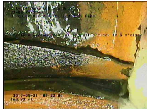
8ce988b6-bc94-4e45-a756-bad07eabe668_20190521_092434_086.jpg, 00:07:48, 163.92ft Fracture Circumferential from 11 o'clock to 5 o'clock
