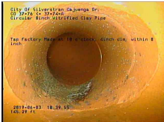
866d1549-f58e-4a8d-bebd-f0c8a4a96987_20190603_104231_177.jpg, 00:10:23, 145.29ft Tap Factory Made at 10 o'clock, 4inch dim, within 8 inch
