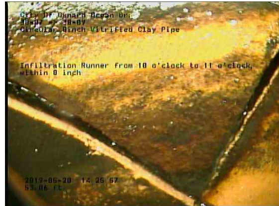
9813adaf-1aad-4115-922e-f835f64123a5_20190520_142827_620.jpg, 00:05:46, 53.06ft Infiltration Runner from 10 o'clock to 11 o'clock, within 8 inch
