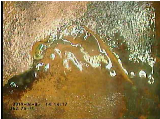
88e62e8e-b940-4b43-8a7c-406a9da3a5e8_20190603_141653_712.jpg, 00:29:48, 362.75ft Fracture Multiple from 3 o'clock to 6 o'clock, Start
