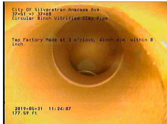
4049ba8a-0ce5-445c-accd-3ecb7dd88335_20190531_112644_672.jpg, 00:09:28, 177.59ft Tap Factory Made at 3 o'clock, 4inch dim, within 8 inch
