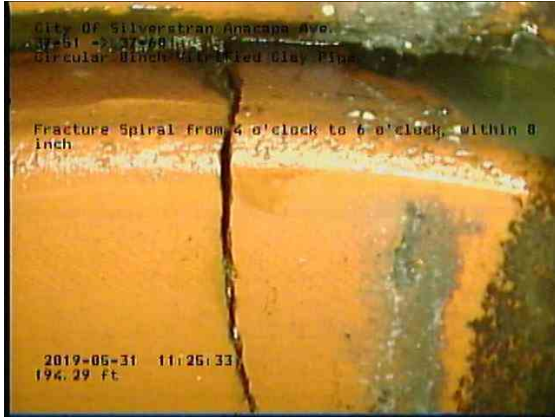
7c04d3fa-33c2-476b-9d1a-d8b42afa7b41_20190531_112809_921.jpg, 00:10:38, 194.29ft Fracture Spiral from 4 o'clock to 6 o'clock, within 8 inch
