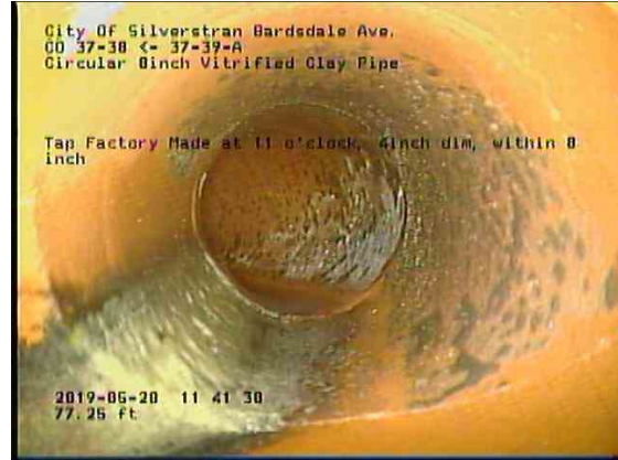
94c6c42f-a8c3-4a7f-aed6-3bb05be224e8_20190528_114404_153.jpg, 00:05:07, 77.25ft Tap Factory Made at 11 o'clock, 4inch dim, within 8 inch
