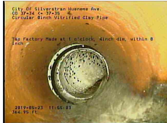
8db6c3e2-2e72-41e7-95d3-08128a8714f8_20190523_115736_463.jpg, 00:23:01, 364.95ft Tap Factory Made at 1 o'clock, 4inch dim, within 8 inch
