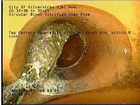
a7971dfb-5684-4199-85f1-42a51bcb7418_20190523_080541_620.jpg, 00:21:28, 341.79ft Tap Factory Made at 11 o'clock, 4inch dim, within 8 inch
