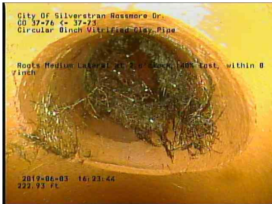
c0a48f71-c261-49dc-8106-a376ccf85ff5_20190603_162621_363.jpg, 00:14:36, 222.93ft Roots Medium Lateral at 2 o'clock, 40% lost, within 8 inch
