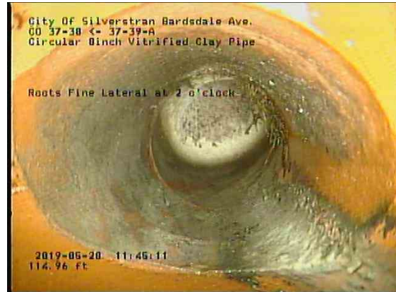
7e17f81f-5db2-47df-abd2-c40691c101d5_20190528_114745_181.jpg, 00:07:42, 114.96ft Roots Fine Lateral at 2 o'clock
