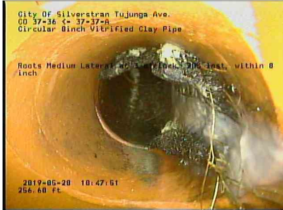
1a1ed1ac-dfe5-4eb1-8727-39ddb803df83_20190528_105024_772.jpg, 00:15:36, 256.60ft Roots Medium Lateral at 3 o'clock, 20% lost, within 8 inch
