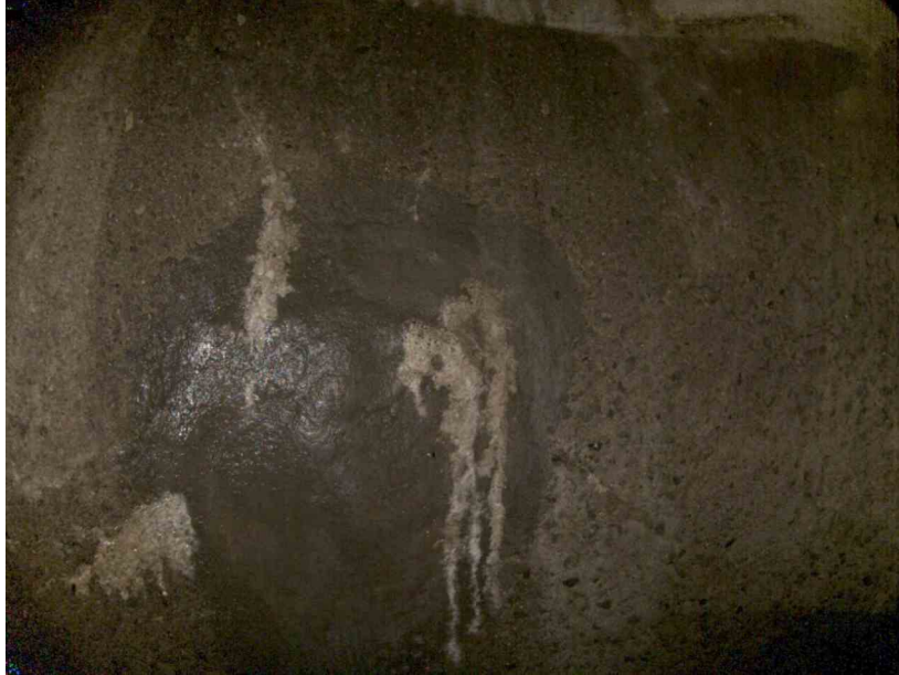
28-09_649da561_021a_4b6c_b8b5_5695380ff438_12f4e905-5732-41ca-8680-3f1580b7b9a8_P12.jpg, , 5.09 Infiltration Stain, from 03 to -01 o'clock, within 8 inch
