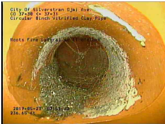
e7913879-e7c3-4ae0-b7bf-e382a7868220_20190523_075415_149.jpg, 00:13:44, 236.65ft Roots Fine Lateral at 11 o'clock
