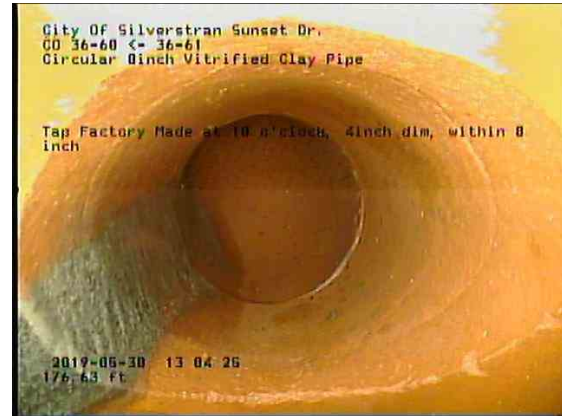
9de485de-7b64-44a6-bf9f-c5f4ded6db73_20190530_130700_481.jpg, 00:10:10, 176.63ft Tap Factory Made at 10 o'clock, 4inch dim, within 8 inch
