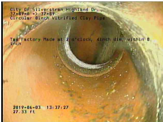
79ff7883-703d-45e1-9113-e7ac4e12b0d1_20190603_134004_562.jpg, 00:04:51, 27.33ft Tap Factory Made at 2 o'clock, 4inch dim, within 8 inch
