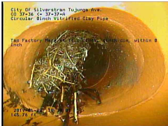
227c3710-37ad-4fc8-b2ee-7f81a107b7f9_20190528_104034_816.jpg, 00:08:54, 145.76ft Tap Factory Made at 11 o'clock, 4inch dim, within 8 inch
