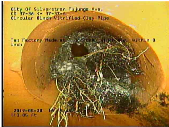
00c22381-a3cc-4dd3-be0f-041aa5dc904d_20190528_103819_503.jpg, 00:07:19, 113.05ft Tap Factory Made at 1 o'clock, 4inch dim, within 8 inch
