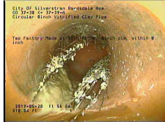
0d2b5184-3e23-4944-9899-27549ebf6259_20190528_115930_389.jpg, 00:16:31, 218.04ft Tap Factory Made at 11 o'clock, 4inch dim, within 8 inch
