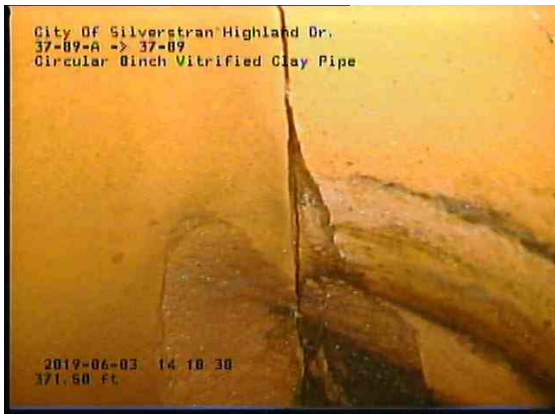
55064868-05dc-4540-819f-005cd62811fa_20190603_142114_902.jpg, 00:33:04, 371.50ft Fracture Longitudinal at 1 o'clock, within 8 inch
