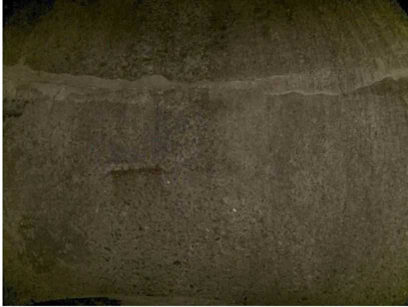
37-89-A_b79949af_46fc_4028_94b0_26ae49ec5641_899e83b9-6c9a-4762-8ffe-2ac3267b634f_P12.jpg, , 7.45 Surface Reinforcement Corroded at 11 o'clock, within 8 inch
