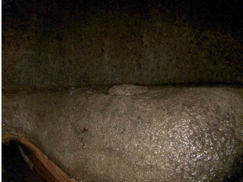
23-05_07f89197_7dd0_4207_a0d5_4ab641627b63_ad9305d6-3ff0-49fe-b190-6f0c8c426190_P12.jpg, , 6.92 Obstacles Construction Debris, 5% of cross sectional area at 3 o'clock
