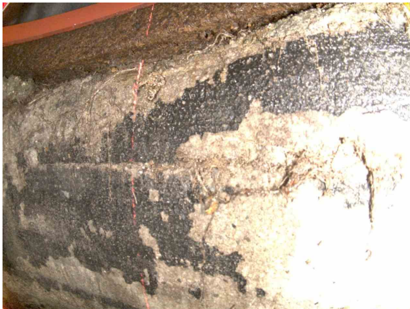
37-89-A_b79949af_46fc_4028_94b0_26ae49ec5641_7b46ce55-72ba-4220-988e-558e8da0b1e2_P12.jpg, , 0.41 Surface Roughness Increased from 12 o'clock to 12 o'clock, within 8 inch, Start
