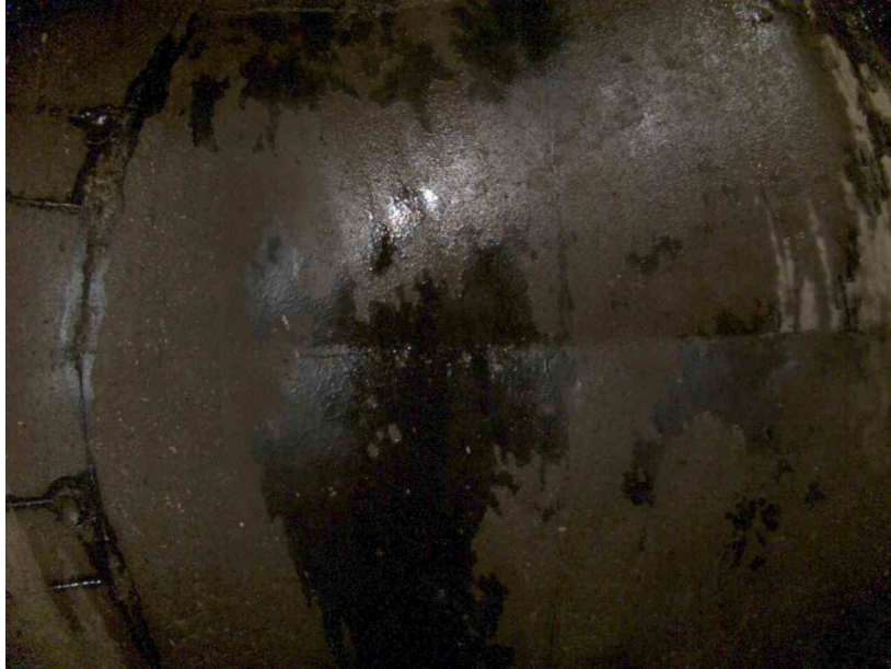
36-78_f20e677b_8ab5_4247_8921_13ab7193ed33_631e5cc8-7fab-493f-9853-2d4277167e13_P12.jpg, , 1.78 Infiltration Stain at 3 o'clock, within 8 inch
