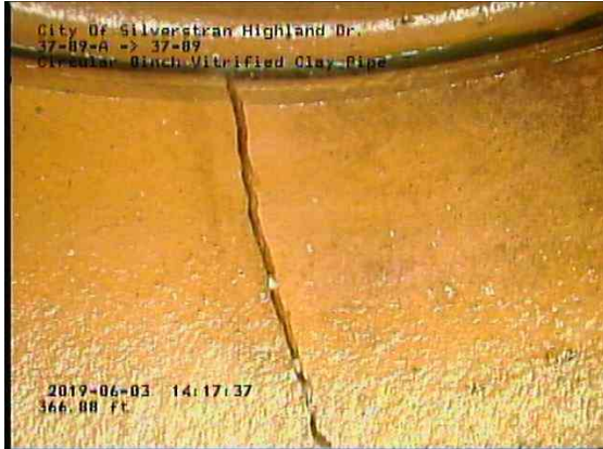
d667f1b9-e8c6-46b0-b434-f6e9173c03cf_20190603_142014_166.jpg, 00:32:14, 366.88ft Fracture Multiple from 3 o'clock to 6 o'clock, Finish
