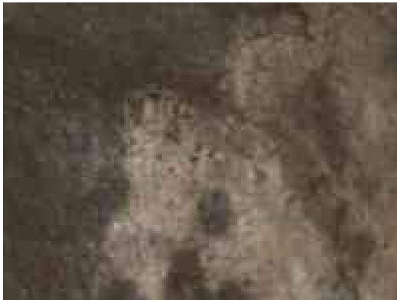
28-09_649da561_021a_4b6c_b8b5_5695380ff438_12f4e905-5732-41ca-8680-3f1580b7b9a8_P11.jpg, , 5.09 Infiltration Stain, from 03 to -01 o'clock, within 8 inch
