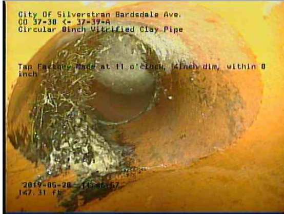
f72bbe40-4144-4c66-9d21-8703b4adf7ad_20190528_114930_950.jpg, 00:09:20, 147.31ft Tap Factory Made at 11 o'clock, 4inch dim, within 8 inch
