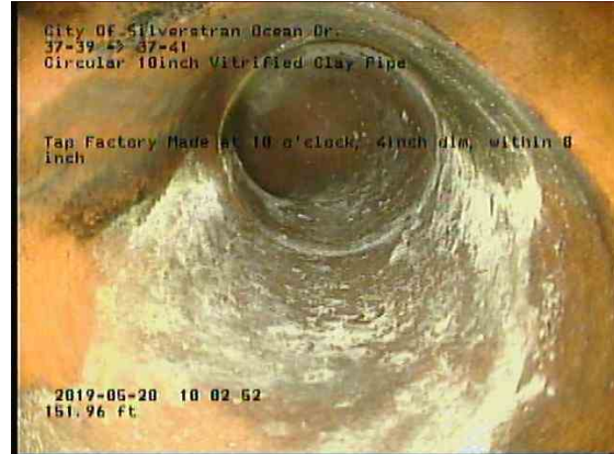
515b3794-7303-4ca6-9eda-0d73f80655a5_20190528_100525_438.jpg, 00:09:07, 151.96ft Tap Factory Made at 10 o'clock, 4inch dim, within 8 inch
