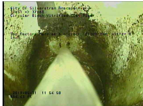
28fc8e88-4286-4667-ae9b-d86c2eeff883_20190531_115727_300.jpg, 00:33:12, 554.43ft Tap Factory Made at 6 o'clock, 8inch dim, within 8 inch
