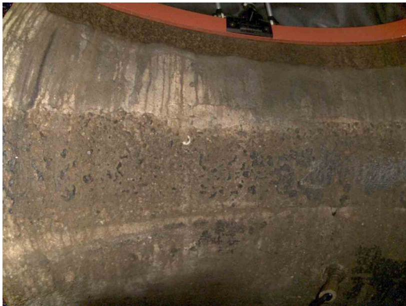
37-35_f6e7d8ee_4d76_46d5_86b4_5a5b78e4e34f_eb079222-a340-4917-a881-a8747db53a69_P12.jpg, , 0.57 Surface Roughness Increased from 12 o'clock to 12 o'clock, within 8 inch, Start
