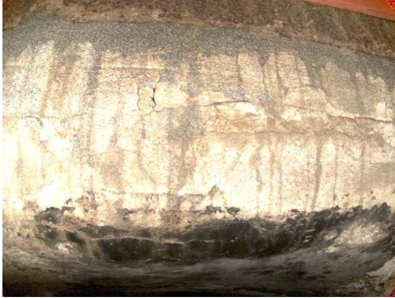
37-39_e3463806_251b_4a10_8598_66aa7b2b50ab_aff92091-f8d5-4490-8d98-ffc28d14534b_P12.jpg, , 0.32 Fracture Circumferential from 12 o'clock to 12 o'clock, within 8 inch
