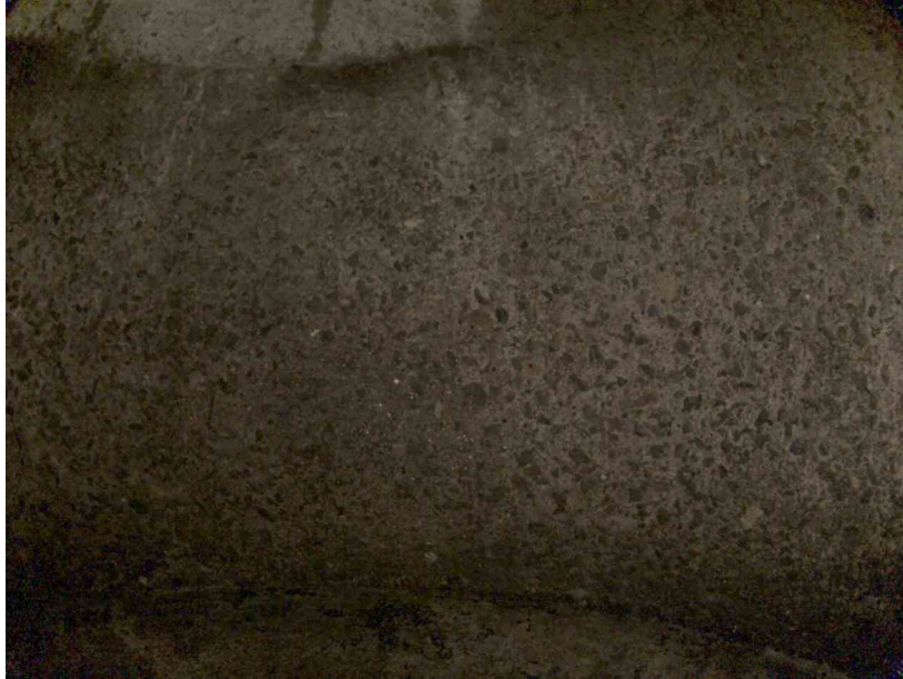
36-61_cd22f785_8cc2_4e9f_ab8d_76fe60c0a5c6_06214432-8949-45fe-b852-6aa60ad19ea5_P12.jpg, , 4.69 Surface Aggregate Visible from 4 o'clock to 9 o'clock, within 8 inch
