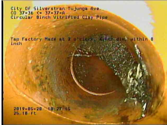
6434f00a-7985-47f4-8500-04e00e7bc849_20190528_102948_595.jpg, 00:01:33, 25.10ft Tap Factory Made at 2 o'clock, 4inch dim, within 8 inch
