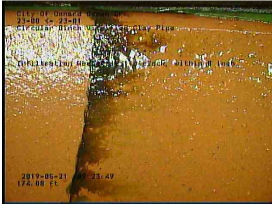
1089121c-01e9-437b-a436-8abcba45f94_20190521_092619_423.jpg, 00:09:00, 174.08ft Infiltration Weeper at 1 o'clock, within 8 inch
