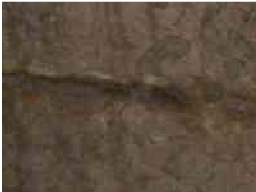
28-09_649da561_021a_4b6c_b8b5_5695380ff438_60335b05-d594-4c98-89f4-79bf729726fe_P11.jpg, , 2.66 Surface Reinforcement Corroded, from 10 to -01 o'clock, within 8 inch
