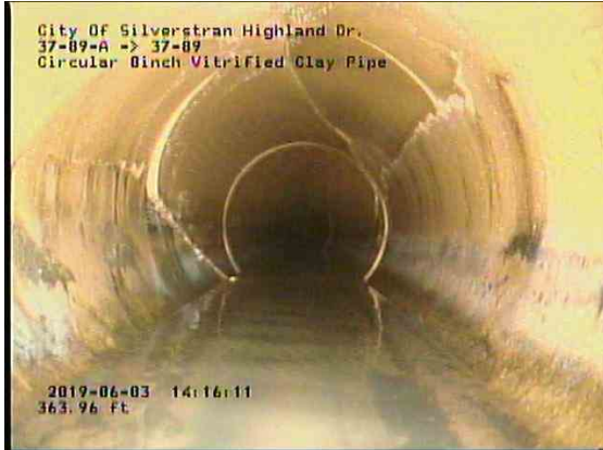
6317c7a3-f0a3-4379-9cdb-94632dc38248_20190603_141848_208.jpg, 00:31:08, 363.96ft Fracture Multiple from 12 o'clock to 12 o'clock
