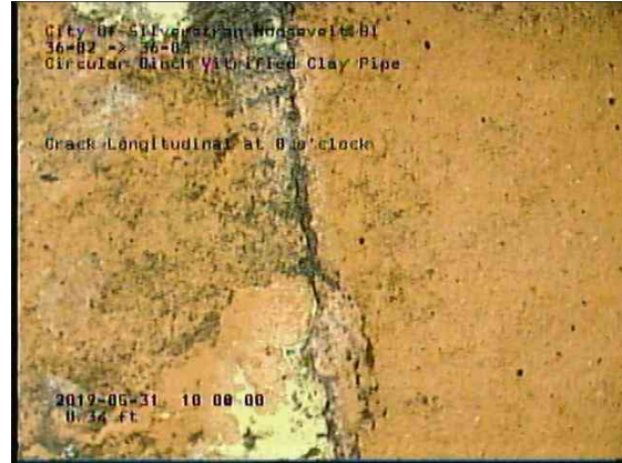
67a54bcb-ae28-4a81-a1ad-10f58d7818a4_20190531_100237_030.jpg, 00:02:10, 0.34ft Crack Longitudinal at 8 o'clock
