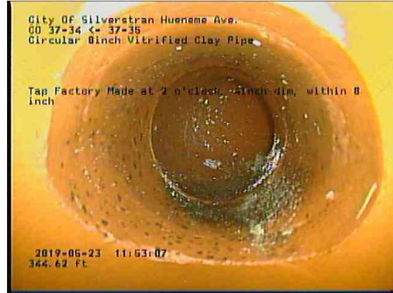
bb8ab630-a199-46e3-9507-3a4655e55d58_20190523_115540_178.jpg, 00:21:23, 344.62ft Tap Factory Made at 2 o'clock, 4inch dim, within 8 inch
