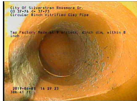
8077d3c7-39e6-44e2-b5e8-98c967a49ede_20190603_16320_0_460.jpg, 00:19:11, 306.41ft Tap Factory Made at 9 o'clock, 4inch dim, within 8 inch
