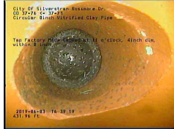
fada6ef2-fa12-4bdf-b211-521083121cc2_20190603_164156_148.jpg, 00:27:23, 431.96ft Tap Factory Made Gapped at 11 o'clock, 4inch dim, within 8 inch
