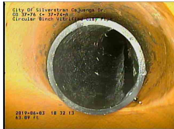
d8943bd3-6856-4fa7-92e9-15689a50ff1c_20190603_103449_852.jpg, 00:04:14, 62.81ft Tap Factory Made Intruding at 2 o'clock, 4inch dim, 1inch intrusion, within 8 inch
