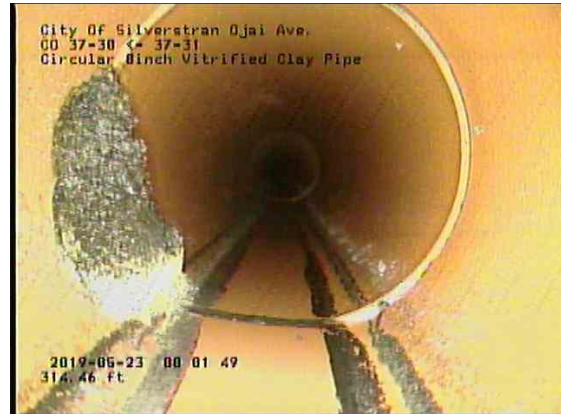
aade38a9-1d8b-429e-abf2-fac66017f932_20190523_080421_710.jpg, 00:19:57, 315.31ft Deposits Attached Encrustation, 10% of cross sectional area from 7 o'clock to 10 o'clock, within 8 inch
