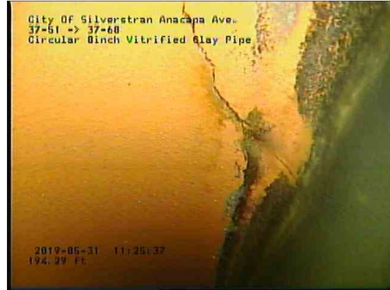
87f06df7-80ba-4055-a3b2-6477e1e44bb7_20190531_112814_292.jpg, 00:10:38, 194.29ft Fracture Spiral from 4 o'clock to 6 o'clock, within 8 inch
