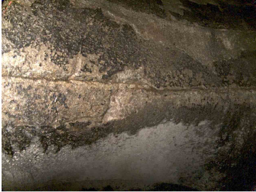
37-68_bc075bf7_3f28_485d_aaf8_7573fec9cbd6_ae7c9cc5-c9a6-4e8a-b4a1-aff349d573cc_P12.jpg, , 1.53 Crack Longitudinal at 7 o'clock, within 8 inch
