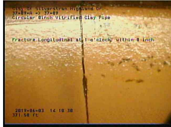
9b4ab3db-0486-4b93-a97b-39dd439dc8b3_20190603_142107_662.jpg, 00:33:04, 371.50ft Fracture Longitudinal at 1 o'clock, within 8 inch
