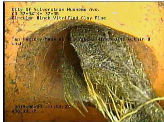
7349739b-7d4a-4465-b77e-64a56cdd28fc_20190523_120156_221.jpg, 00:26:52, 430.22ft Tap Factory Made at 1 o'clock, 4inch dim, within 8 inch
