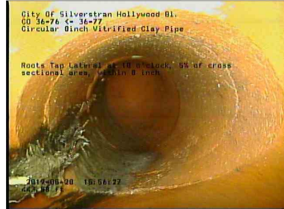
c1b62526-2c3e-4a8e-9163-c5b22d037d9f_20190528_155901_725.jpg, 00:26:20, 443.58ft Roots Tap Lateral at 10 o'clock, 5% of cross sectional area, within 8 inch
