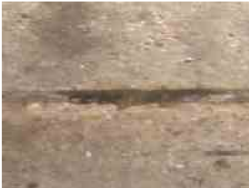
28-09_649da561_021a_4b6c_b8b5_5695380ff438_b885c202-bd32-45ca-881d-169679afd8a0_P11.jpg, , 1.96 Surface Reinforcement Corroded, from 04 to -01 o'clock, within 8 inch
