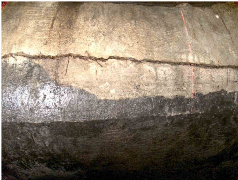
37-39-A_545e9b99_6729_4fa7_8d17_f1c1b7c45969_4a412c8f-4bc0-47dc-afd3-4bde88606715_P12.jpg, , 0.83 Fracture Circumferential from 12 o'clock to 12 o'clock, within 8 inch
