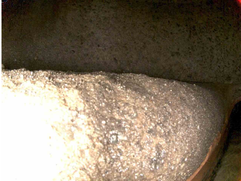
28-09_649da561_021a_4b6c_b8b5_5695380ff438_46b2a042-f0c1-4b8d-81b9-c02dd1b32027_P12.jpg, , 9.25 Surface Roughness Increased, from 03 to -01 o'clock, within 8 inch, F01
