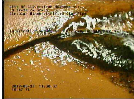
a75875b2-0b7e-4147-b681-2ae0c220a959_20190523_113310_504.jpg, 00:02:58, 10.67ft Infiltration Gusher at 3 o'clock, within 8 inch
