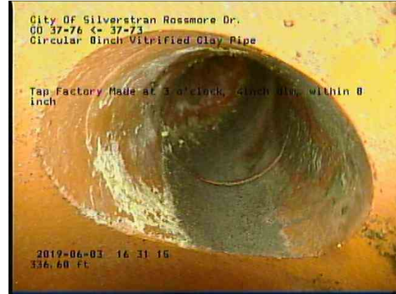
969bb0b6-8d0f-4216-a0b2-1500664cd222_20190603_163352_129.jpg, 00:20:49, 336.60ft Tap Factory Made at 3 o'clock, 4inch dim, within 8 inch
