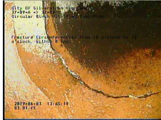
cdce7c1a-d787-4c02-9196-6b9f0130ed73_20190603_134756_575.jpg, 00:09:44, 83.01ft Fracture Circumferential from 12 o'clock to 12 o'clock, within 8 inch / IN WYE
