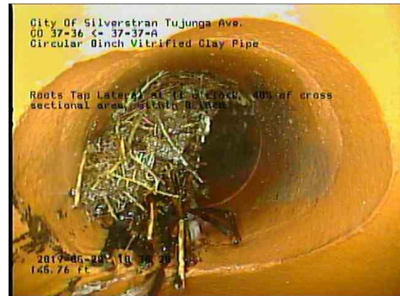
46cd208d-ca34-45ee-beaf-de15ecf82fa8_20190528_104101_398.jpg, 00:08:57, 145.76ft Roots Tap Lateral at 11 o'clock, 40% of cross sectional area, within 8 inch
