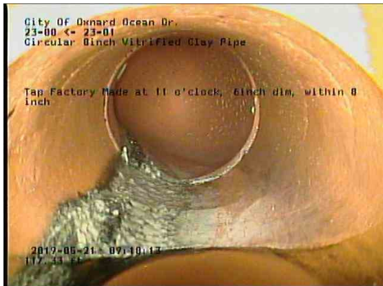
e4040fec-df2c-49a4-bc7a-1ec55dd3b199_20190521_092042_930.jpg, 00:04:40, 117.33ft Tap Factory Made at 11 o'clock, 8inch dim, within 8 inch
