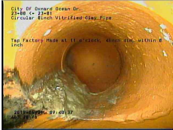
22c4c2a9-7ad4-4584-a246-7ece61f1421d_20190521_094307_860.jpg, 00:24:07, 463.28ft Tap Factory Made at 11 o'clock, 4inch dim, within 8 inch
