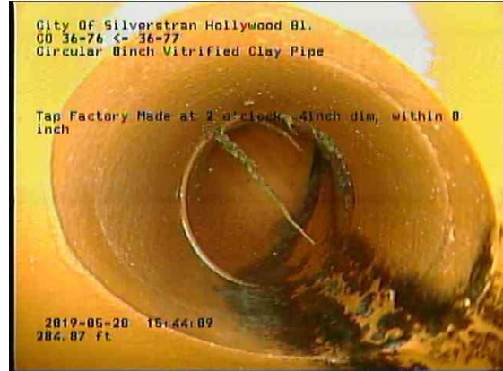
5856e717-f881-4ff5-bc50-d1c6fbe9e8f0_20190528_154643_71.jpg, 00:16:05, 284.87ft Tap Factory Made at 2 o'clock, 4inch dim, within 8 inch
