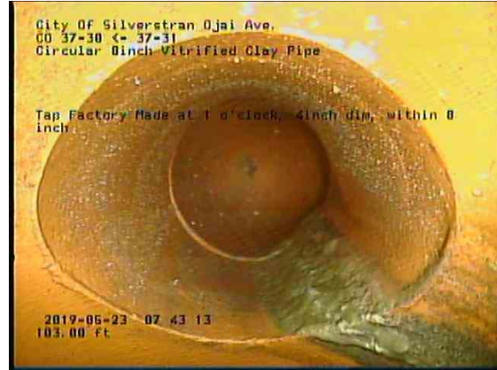
20226ff-e0f0-4721-9320-f510f0cd05d7_20190523_074545_664.jpg, 00:06:38, 103.00ft Tap Factory Made at 1 o'clock, 4inch dim, within 8 inch
