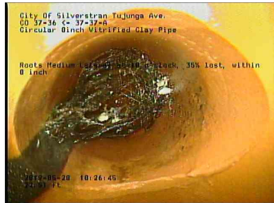
150e1c3d-fa8f-439e-8929-ab8b5f708665_20190528_102918_345.jpg, 00:01:12, 22.51ft Roots Medium Lateral at 10 o'clock, 35% lost, within 8 inch
