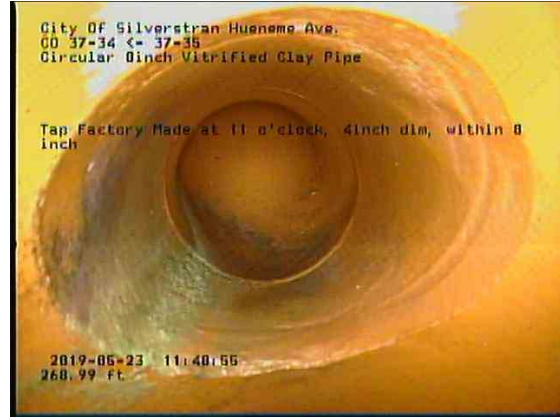
e41b79a6-f05b-43db-a787-3409d276be7c_20190523_115128_978.jpg, 00:17:47, 268.99ft Tap Factory Made at 11 o'clock, 4inch dim, within 8 inch
