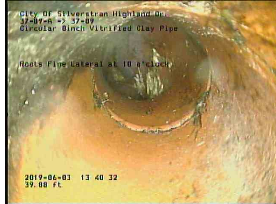
c56dec65-e9b1-40e8-9b5d-e918f06d136c_20190603_134308_754.jpg, 00:05:57, 39.85ft Roots Fine Lateral at 10 o'clock
