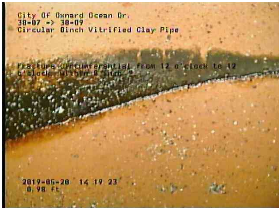
7b424d15-16e0-4dad-a7d2-83f66133d5b9_20190520_142153_017.jpg, 00:00:50, 0.98ft Fracture Circumferential from 12 o'clock to 12 o'clock, within 8 inch
