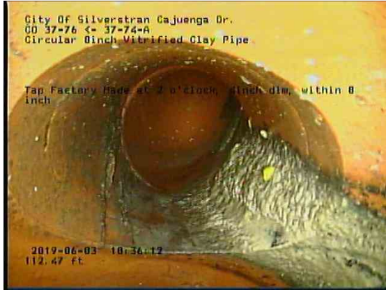
af9cf710-93dc-4259-b13b-99c0356a902b_20190603_103848_560.jpg, 00:07:27, 112.47ft Tap Factory Made at 2 o'clock, 4inch dim, within 8 inch
