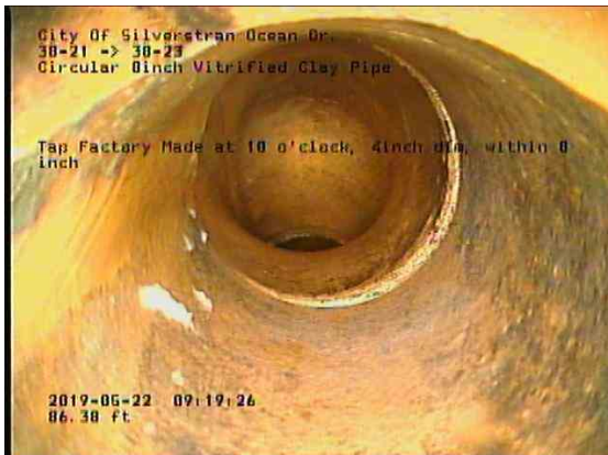
4524ba70-9092-41d6-857d-9f6810dde421_20190522_092157_129.jpg, 00:05:04, 86.38ft Tap Factory Made at 10 o'clock, 4inch dim, within 8 inch
