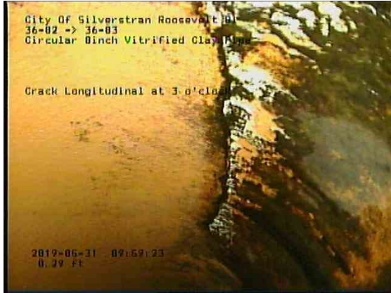
d1aec621-6e2d-4199-ba37-05269a0cd597_20190531_100200_309.jpg, 00:01:42, 0.29ft Crack Longitudinal at 3 o'clock
