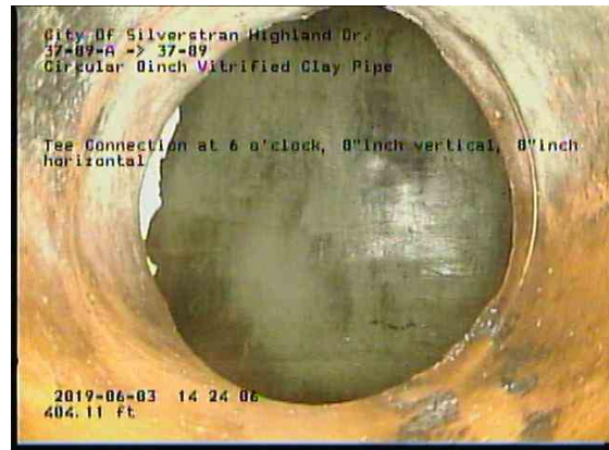
e4f6c3fb-f390-42ca-bd59-7411a5a89d15_20190603_142643_276.jpg, 00:36:47, 404.11ft Tee Connection at 6 o'clock, 8"inch vertical, 8"inch horizontal / DROP
