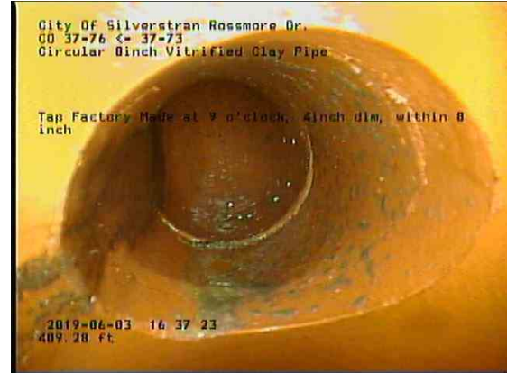
d780113e-9ee1-477e-9ac7-5b6ba3cd91a5_20190603_16400_0_370.jpg, 00:25:57, 409.28ft Tap Factory Made at 9 o'clock, 4inch dim, within 8 inch
