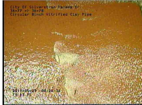
4320f3cb-dbb7-4d81-9841-23bfd7bc4caf_20190529_082308_825.jpg, 00:08:37, 79.63ft Infiltration Stain from 2 o'clock to 3 o'clock, within 8 inch
