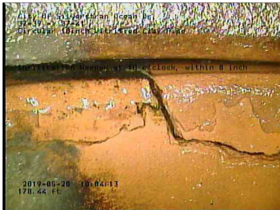
4b374689-ef56-482a-bf3f-000ceb249ea0_20190528_100646_722.jpg, 00:10:16, 178.44ft Infiltration Weeper at 10 o'clock, within 8 inch
