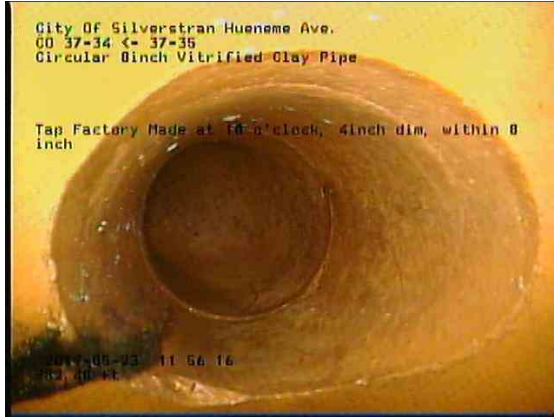
ae695281-3a20-4217-95be-8fb32e416a29_20190523_115849_014.jpg, 00:24:03, 382.40ft Tap Factory Made at 10 o'clock, 4inch dim, within 8 inch
