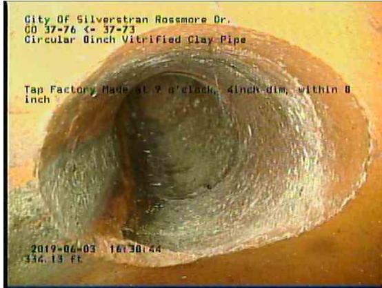
5e7b6973-5e5f-41d0-b9c7-2c34502f86bb_20190603_163321_503.jpg, 00:20:25, 334.13ft Tap Factory Made at 9 o'clock, 4inch dim, within 8 inch
