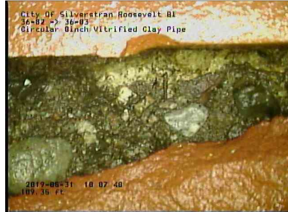
3b223a3f-84a2-4741-9c4f-2ab95f58b030_20190531_101025_650.jpg, 00:08:56, 109.35ft Broken from 7 o'clock to 5 o'clock
