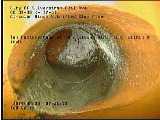
fb0b797a-1335-4275-8407-ea137d25030d_20190523_07485_5_409.jpg, 00:09:21, 160.86ft Tap Factory Made at 10 o'clock, 4inch dim, within 8 inch
