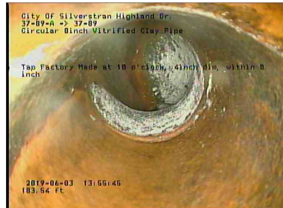
c901f3cd-c378-4290-aff3-fa2ab3ce0c37_20190603_135821_702.jpg, 00:18:18, 183.54ft Tap Factory Made at 10 o'clock, 4inch dim, within 8 inch
