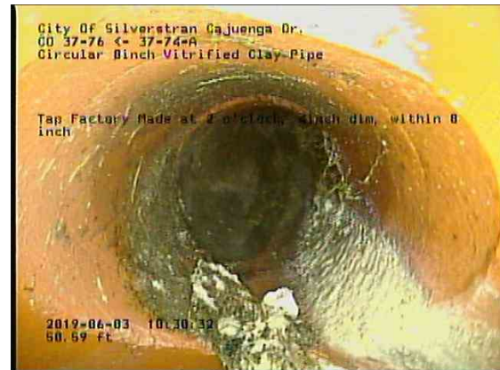
9c0e9dd0-1021-4d9d-90a5-b33e33b5cdfc_20190603_103308_227.jpg, 00:03:15, 50.58ft Tap Factory Made at 2 o'clock, 4inch dim, within 8 inch
