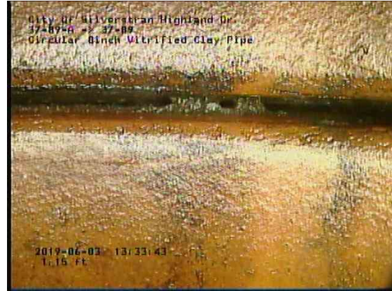
a85e7591-a2c5-4ec8-a54f-c4f37cb39169_20190603_133619_671.jpg, 00:01:43, 1.15ft Crack Circumferential from 10 o'clock to 4 o'clock, within 8 inch
