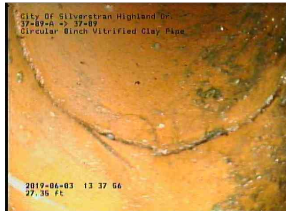
dd52113a-f0c0-4e3a-8142-b334e872fb46_20190603_134033_304.jpg, 00:04:53, 27.35ft Fracture Circumferential from 12 o'clock to 12 o'clock, within 8 inch / IN WYE
