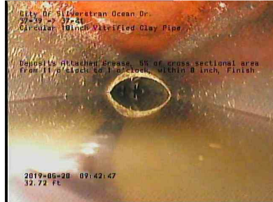
2ee2d9d3-a998-4754-80fe-9f4de364d08a_20190528_094520_855.jpg, 00:03:25, 32.72ft Deposits Attached Grease, 5% of cross sectional area from 11 o'clock to 1 o'clock, within 8 inch, Finish
