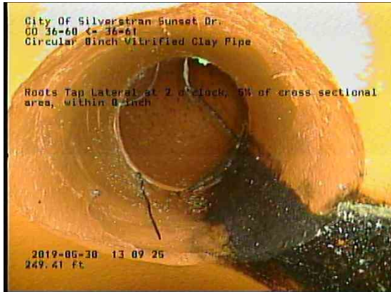
bf925c9a-aa15-4d41-9f43-3e415566cfa4_20190530_131200_923.jpg, 00:14:09, 249.41ft Roots Tap Lateral at 2 o'clock, 5% of cross sectional area, within 8 inch
