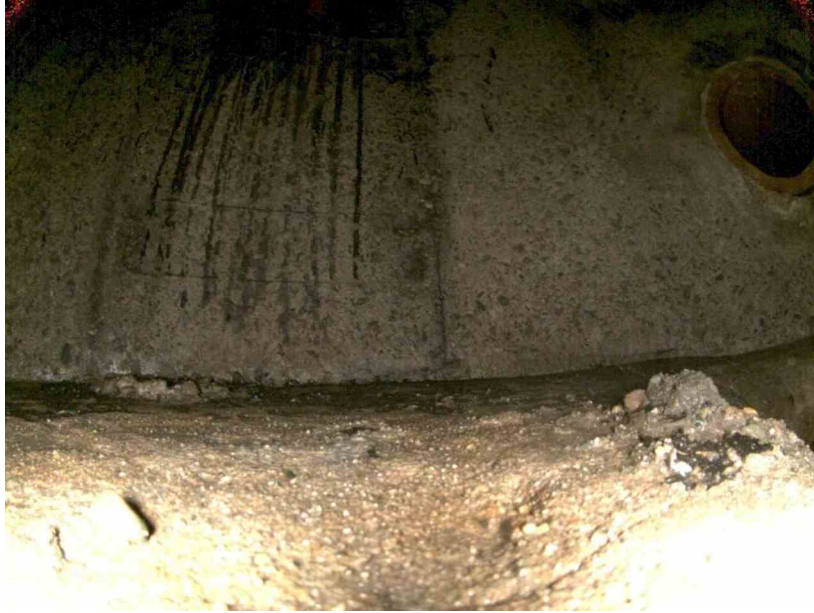
37-51_34621632_ace1_4c3b_9051_30e3d1d9a3a6_d15850d1-7919-4898-87c9-4ce2826f6222_P12.jpg, , 6.19 Deposits Settled Compacted, 5% of cross sectional area at 2 o'clock, within 8 inch
