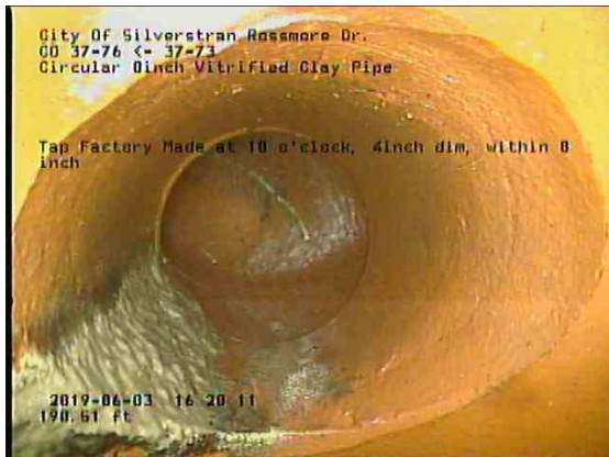
9731e98d-8d47-4f49-ba71-24adf3386b3d_20190603_162248_571.jpg, 00:12:13, 190.50ft Tap Factory Made at 10 o'clock, 4inch dim, within 8 inch
