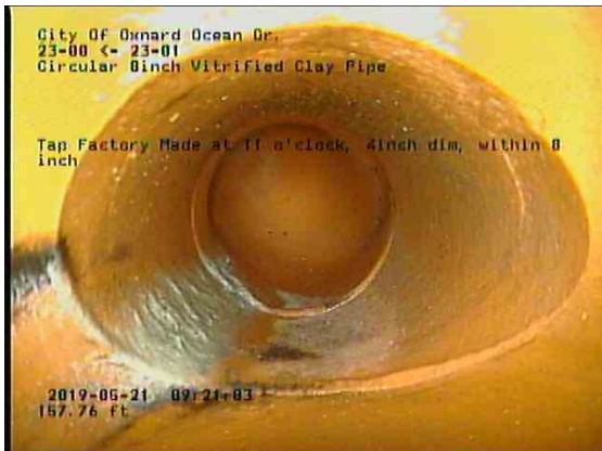
8400e27f-701f-4f90-a2a5-9c0c797ac391_20190521_092333_335.jpg, 00:07:05, 157.76ft Tap Factory Made at 11 o'clock, 4inch dim, within 8 inch
