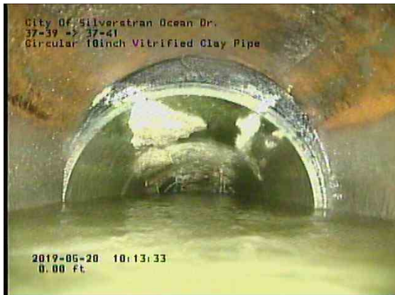
7cb4f904-99a8-4977-be9a-fd16cefdee22_20190528_101606_700.jpg, 00:03:30, 7.39ft Water Level, Sag in pipe, 80% of the vertical dimension, Start
