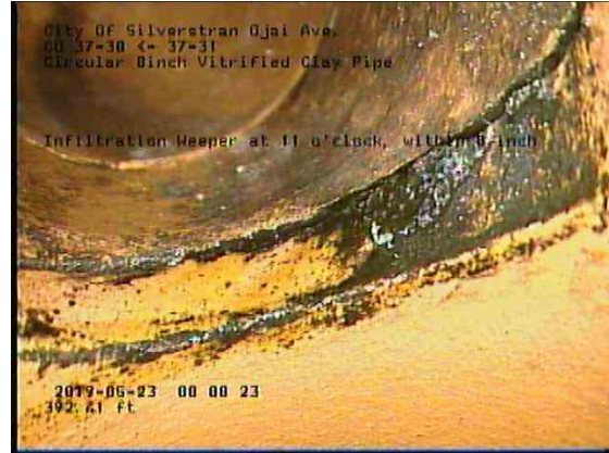
23cbcb3a-979d-45fa-bf95-59a814dfe25c_20190523_081055_538.jpg, 00:25:11, 392.41ft Infiltration Weeper at 11 o'clock, within 8 inch / IN WYE
