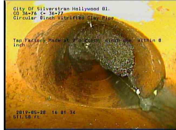
63e71fc8-0110-4741-909d-13f943fd31b2_20190528_160408_944.jpg, 00:30:21, 511.50ft Tap Factory Made at 2 o'clock, 4inch dim, within 8 inch
