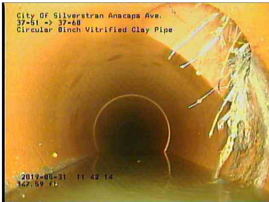
299bc29e-c79a-402e-8ba2-e16d5b0eb10a_20190531_114451_555.jpg, 00:21:45, 348.71ft Roots Ball Lateral at 2 o'clock, 75% lost, within 8 inch
