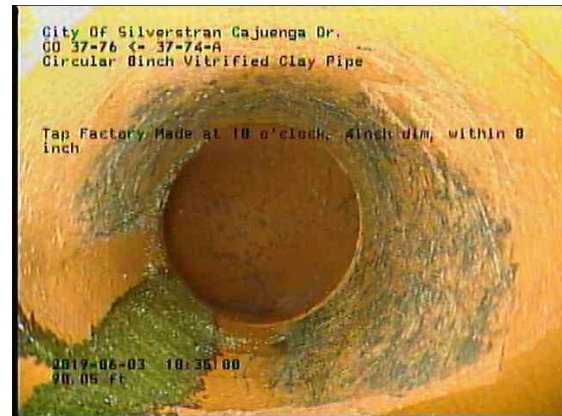
1783ae07-84d0-4f0c-9322-5e546dffbd47_20190603_103736_351.jpg, 00:06:23, 90.05ft Tap Factory Made at 10 o'clock, 4inch dim, within 8 inch
