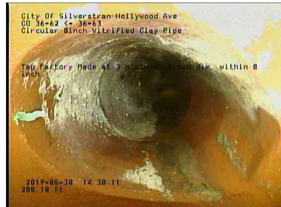
f90d2f57-9363-4119-bb9b-00e5a9b6aeb0_20190530_143246_421.jpg, 00:15:01, 208.18ft Tap Factory Made at 3 o'clock, 4inch dim, within 8 inch
