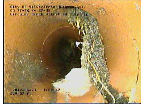
7cd76eec-8235-401e-868b-6775c5736d59_20190523_12022_2_946.jpg, 00:26:55, 430.22ft Roots Ball Lateral at 1 o'clock, 65% lost, within 8 inch
