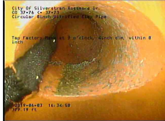
b2b8ec43-b45c-41d7-a5f8-4bfff6ad618_20190603_163727_599.jpg, 00:23:52, 379.19ft Tap Factory Made at 9 o'clock, 4inch dim, within 8 inch
