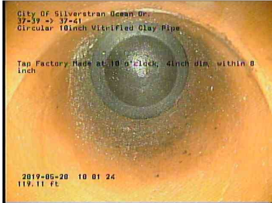
84981bbd-fc2c-4114-b72d-b5def5291514_20190528_100357_663.jpg, 00:07:46, 119.11ft Tap Factory Made at 10 o'clock, 4inch dim, within 8 inch
