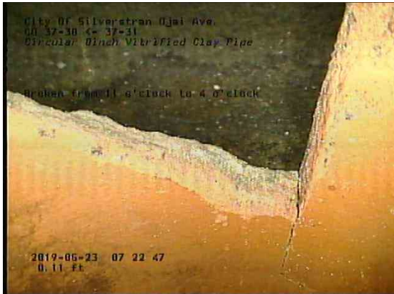
b8b02119-77e8-4eb8-ae8b-b9bf0fc53d41_20190523_072520_430.jpg, 00:00:47, 0.11ft Broken from 11 o'clock to 4 o'clock
