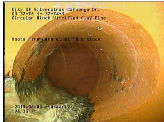
55a03279-92f1-4f4b-bdfc-fbff174b5ee3_20190603_104648_149.jpg, 00:13:21, 196.35ft Roots Fine Lateral at 10 o'clock
