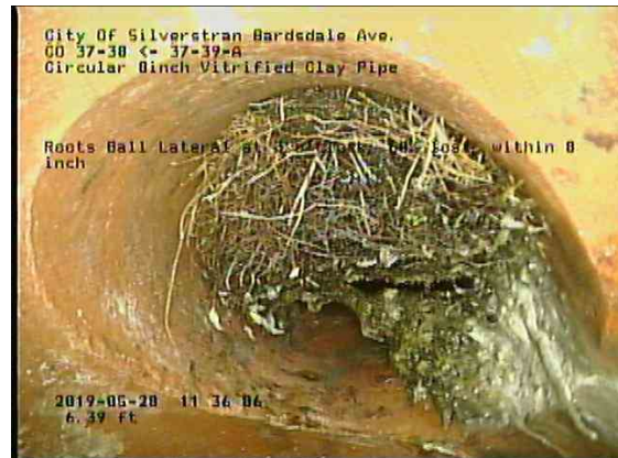
cf6d5b63-573e-47d1-bac6-ad94d0217abe_20190528_113840_076.jpg, 00:00:38, 6.39ft Roots Ball Lateral at 3 o'clock, 60% lost, within 8 inch
