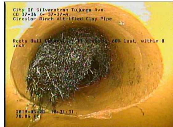
dd394de8-2880-4815-a93b-d8e57e5e5eb6_20190528_10340_614.jpg, 00:04:26, 78.05ft Roots Ball Lateral at 11 o'clock, 60% lost, within 8 inch
