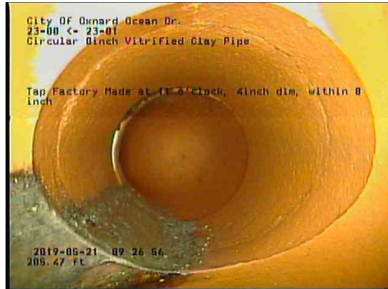
2b7cf24c-6bb7-43b9-b084-bce5a7592178_20190521_092926_031.jpg, 00:11:40, 205.47ft Tap Factory Made at 11 o'clock, 4inch dim, within 8 inch
