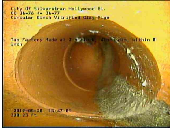
3662e0d4-600e-494d-8e43-72e0c1ddc8cb_20190528_154935_258.jpg, 00:18:24, 320.23ft Tap Factory Made at 2 o'clock, 4inch dim, within 8 inch
