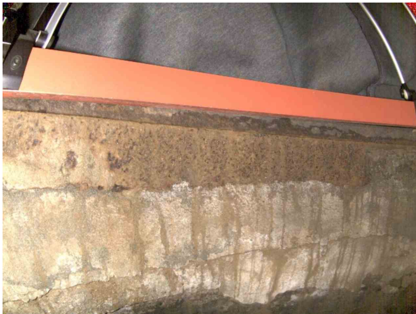
38-21_d8133f19_15ad_4f3f_8ad3_1a1fbd3e9bcc_dbb02aab-ad39-4ede-a058-eb7f5cf2afe2_P12.jpg, , 0.09 Surface Roughness Increased from 12 o'clock to 12 o'clock, within 8 inch, Start
