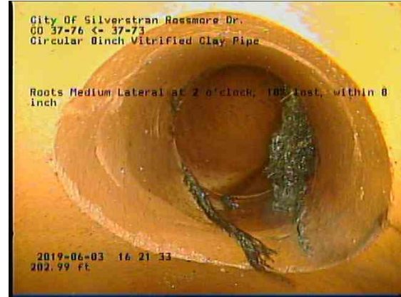
4279d3b2-3530-4101-a3ec-08d218e677a5_20190603_162410_926.jpg, 00:13:03, 202.99ft Roots Medium Lateral at 2 o'clock, 10% lost, within 8 inch
