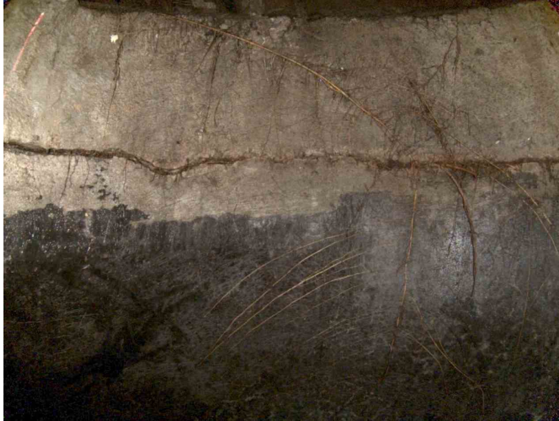
37-39-A_545e9b99_6729_4fa7_8d17_f1c1b7c45969_eafdd2e2-26fb-49c3-870f-206620ecf4eb_P12.jpg, , 0.82 Roots Fine Joint from 8 o'clock to 12 o'clock, within 8 inch
