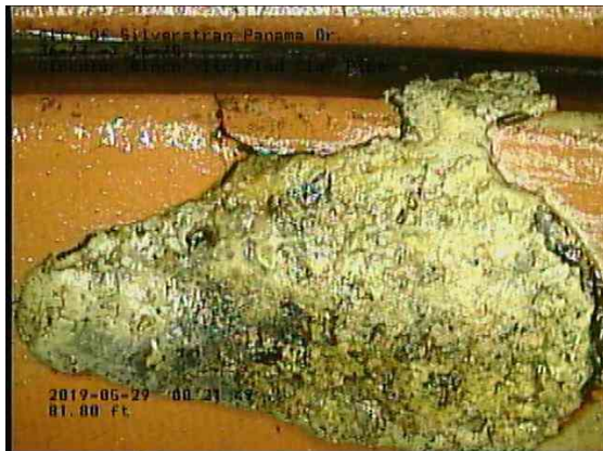
5d48d87d-0f31-4f37-909b-cbd75ccc1489_20190529_082423_444.jpg, 00:09:35, 81.80ft Deposits Attached Encrustation, 5% of cross sectional area from 3 o'clock to 4 o'clock, within 8 inch
