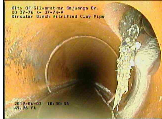
8bb730ee-7fac-4dcc-91c2-427a8a707be6_20190603_103332_317.jpg, 00:03:18, 50.61ft Roots Tap Lateral at 2 o'clock, 5% of cross sectional area, within 8 inch
