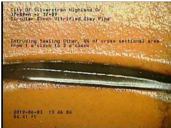
3e24f40d-b9e4-4b2a-874a-ecce73c469e1_20190603_134841_463.jpg, 00:10:07, 84.41ft Intruding Sealing Other, 5% of cross sectional area from 1 o'clock to 3 o'clock
