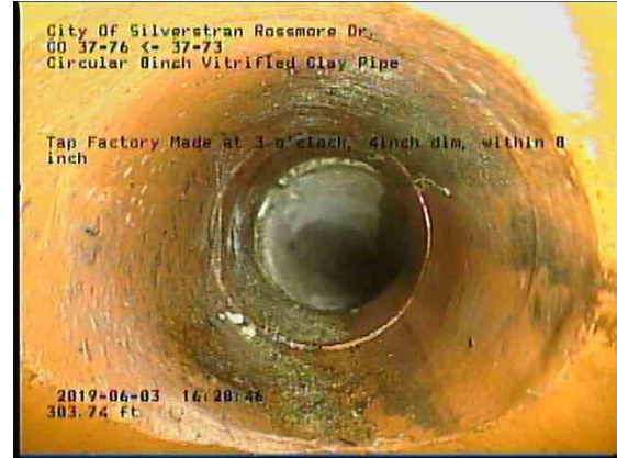
92003d04-6211-41c2-968a-1deb72576397_20190603_16312_3_828.jpg, 00:18:47, 303.74ft Tap Factory Made at 3 o'clock, 4inch dim, within 8 inch
