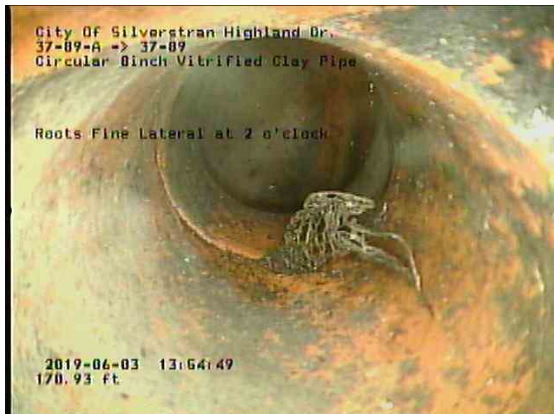
3e79ccac-b4e7-4f25-8204-92605086ebbe_20190603_135726_397.jpg, 00:17:30, 170.93ft Roots Fine Lateral at 2 o'clock
