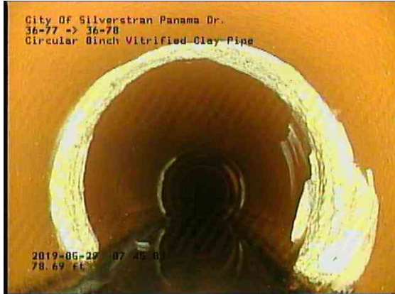
4cad1372-cc26-43ed-aea4-784793960e52_20190529_074736_851.jpg, 00:08:00, 79.85ft Deposits Attached Encrustation, 5% of cross sectional area from 7 o'clock to 5 o'clock, within 8 inch
