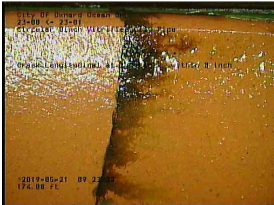
63680215-e72c-441a-857e-45dddba39d1_20190521_092602_832.jpg, 00:08:53, 174.08ft Crack Longitudinal at 1 o'clock, within 8 inch
