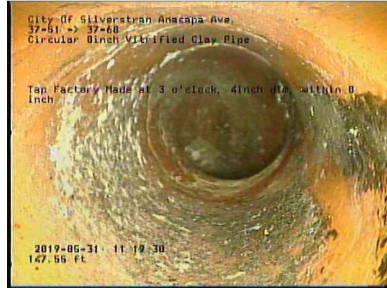
45a319b9-c594-4cc0-b51f-14f2ce87cf96_20190531_112207_072.jpg, 00:07:13, 147.55ft Tap Factory Made at 3 o'clock, 4inch dim, within 8 inch
