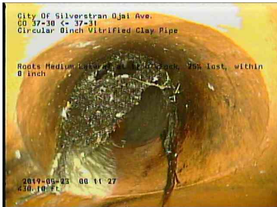
d2df6b6d-c6f6-4efd-a15e-08a3131319ab_20190523_081400_224.jpg, 00:27:26, 430.10ft Roots Medium Lateral at 11 o'clock, 25% lost, within 8 inch
