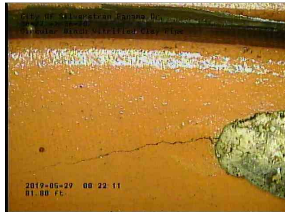
33b5cdbd-81c0-4b21-8e21-8f3dc9129e9e_20190529_082445_336.jpg, 00:10:03, 81.80ft Fracture Multiple from 2 o'clock to 7 o'clock, within 8 inch
