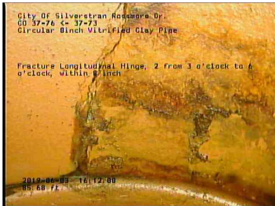
12ee4e9a-8af2-4ce9-b917-794cda158ff8_20190603_161445_835.jpg, 00:05:41, 85.68ft Fracture Longitudinal Hinge, 2 from 3 o'clock to 6 o'clock, within 8 inch
