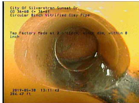
f5ede0d9-6ff0-4b72-89c9-bb24c209bdaa_20190530_131417_994.jpg, 00:15:55, 284.47ft Tap Factory Made at 2 o'clock, 4inch dim, within 8 inch
