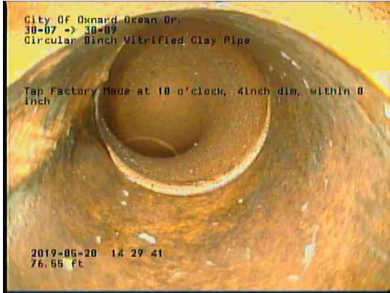
ab90cfa2-1149-4fbf-9923-de41c21aacb8_20190520_143211_690.jpg, 00:07:55, 76.55ft Tap Factory Made at 10 o'clock, 4inch dim, within 8 inch
