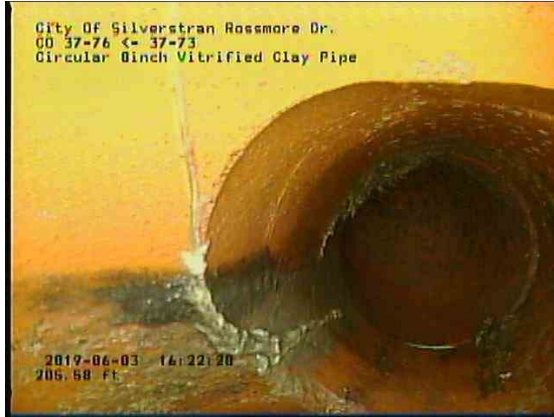
25d32a26-f39d-45fb-8b0a-5339a0e9564d_20190603_162505_447.jpg, 00:13:25, 205.58ft Roots Fine Lateral at 10 o'clock
