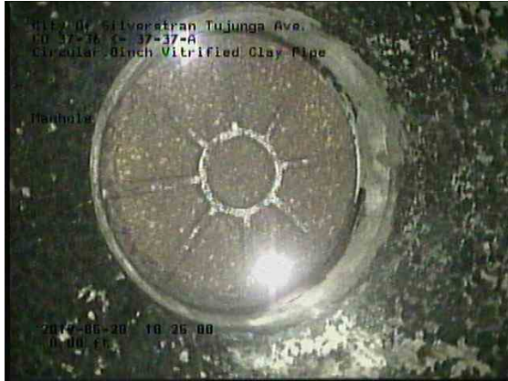
3187303d-c90b-43d4-9562-afe4a07ce747_20190528_102733_536.jpg, 00:00:01, 0.00ft Manhole / 37-37-A
