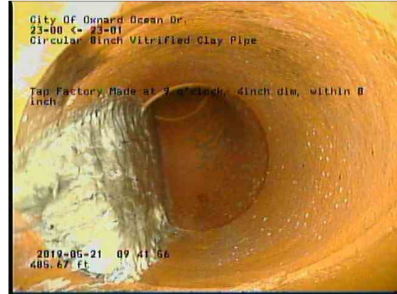
c23c4a5b-7ff8-413a-a149-3db9875a38eb_20190521_094426_134.jpg, 00:25:18, 485.67ft Tap Factory Made at 9 o'clock, 4inch dim, within 8 inch
