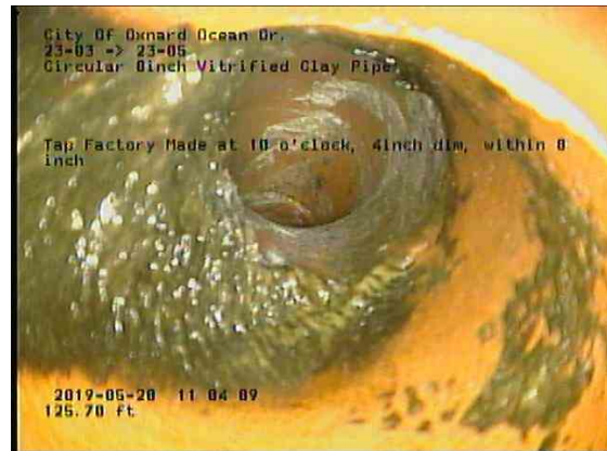
e8a3a889-e43f-4ebc-821f-f6c25e151619_20190520_110639_174.jpg, 00:09:08, 125.70ft Tap Factory Made at 10 o'clock, 4inch dim, within 8 inch
