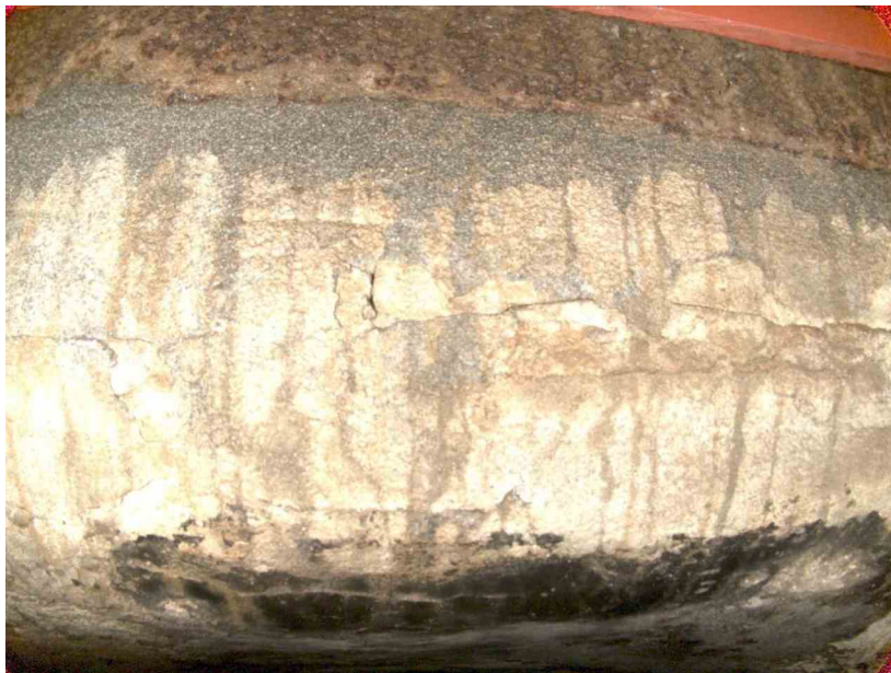
37-39_e3463806_251b_4a10_8598_66aa7b2b50ab_d42f4c79-438b-47a5-a7b6-eb8b41b884d7_P12.jpg, , 0.25 Fracture Longitudinal at 6 o'clock, within 8 inch
