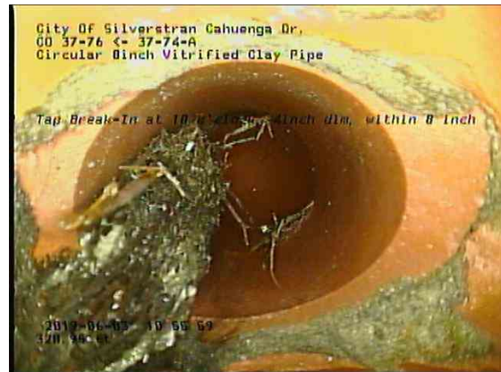
1f118b91-e65a-4fb1-adcb-e5cf3b761c61_20190603_105835_264.jpg, 00:20:55, 320.95ft Tap Break-In at 10 o'clock, 4inch dim, within 8 inch
