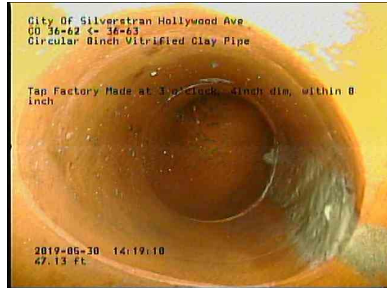
10726aeb-e1f7-4e67-93ac-0be0c7318d91_20190530_142145_683.jpg, 00:05:57, 47.13ft Tap Factory Made at 3 o'clock, 4inch dim, within 8 inch
