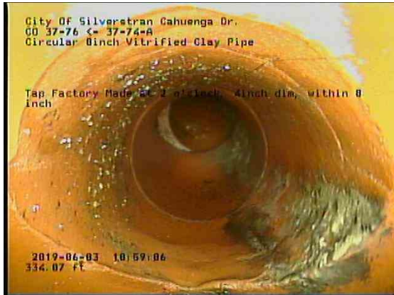
8b12378f-4054-407a-a16b-fdf505aa86da_20190603_110142_667.jpg, 00:22:27, 334.07ft Tap Factory Made at 2 o'clock, 4inch dim, within 8 inch
