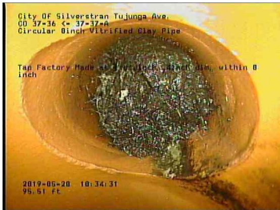
5a61fbd4-d1a6-4a1b-a303-a33b234e3653_20190528_103704_871.jpg, 00:06:25, 95.51ft Tap Factory Made at 1 o'clock, 4inch dim, within 8 inch
