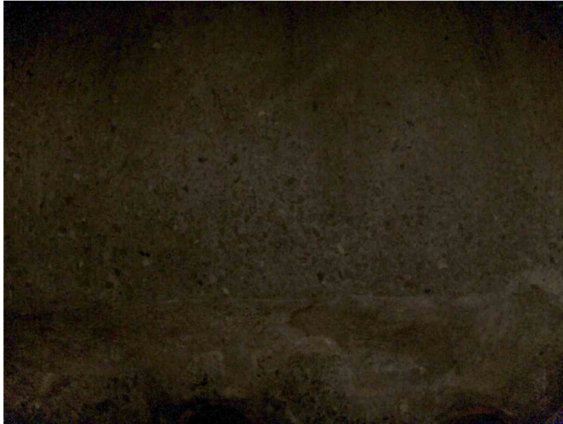
23-03_caf8412c_d397_4fc6_88c9_a9658e397a0b_7b234076-fa6b-4044-bb5d-1f03e63d504a_P12.jpg, , 5.52 Surface Aggregate Visible, from 05 to -01 o'clock, within 8 inch
