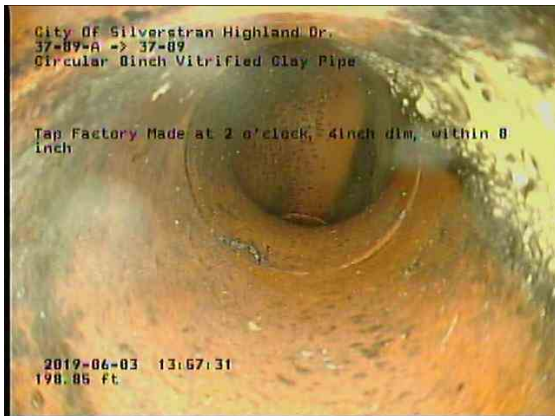
929d05b9-c0b5-4392-b702-fa8a64e5348f_20190603_140007_892.jpg, 00:19:39, 198.85ft Tap Factory Made at 2 o'clock, 4inch dim, within 8 inch
