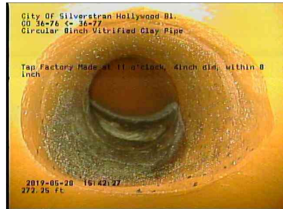
e670947b-55a6-466f-b6a6-8093e1cccdfb_20190528_154501_508.jpg, 00:14:47, 272.25ft Tap Factory Made at 11 o'clock, 4inch dim, within 8 inch
