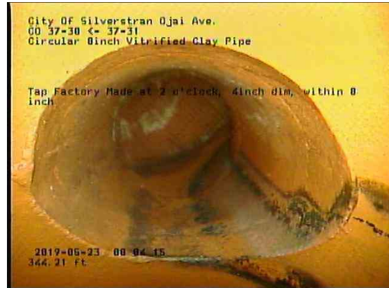
ccc697e8-08ef-4de2-b37a-4d9b32168a80_20190523_080648_199.jpg, 00:22:03, 344.21ft Tap Factory Made at 2 o'clock, 4inch dim, within 8 inch
