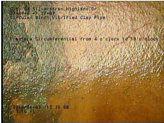
2a62dad1-8fea-44a4-b66d-9250c9a860cc_20190603_133737_478.jpg, 00:02:41, 3.15ft Fracture Circumferential from 4 o'clock to 10 o'clock
