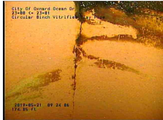
4b3dfa1c-ddf3-4434-a720-5a650ddf39ba_20190521_092636_578.jpg, 00:08:53, 174.08ft Crack Longitudinal at 1 o'clock, within 8 inch
