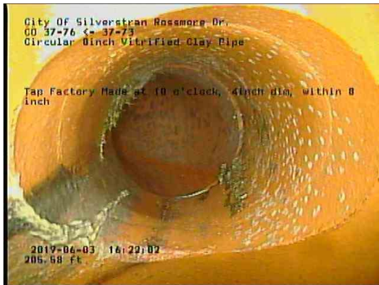
e07fb510-c49c-4313-9d80-4729120041a4_20190603_162439_995.jpg, 00:13:23, 205.58ft Tap Factory Made at 10 o'clock, 4inch dim, within 8 inch
