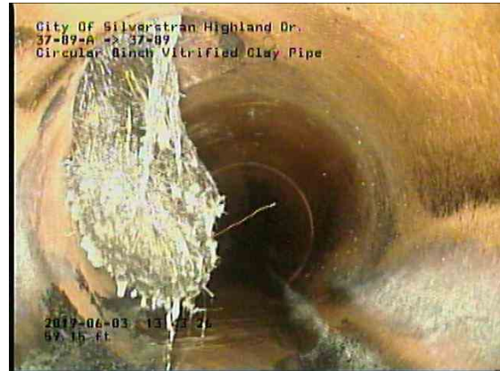
50d63618-ce2b-45f1-9ef5-9663706931e2_20190603_134603_002.jpg, 00:07:58, 59.96ft Roots Tap Lateral at 10 o'clock, 50% of cross sectional area, within 8 inch
