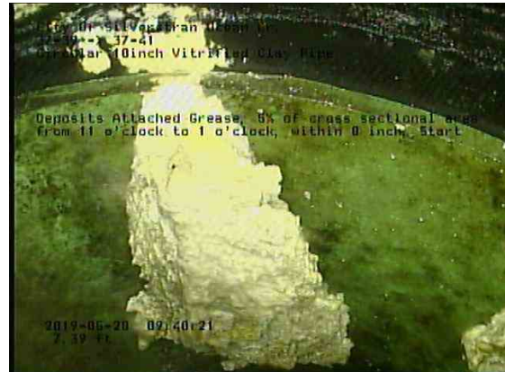
3fd36d85-65e8-4741-8fc4-daebe1d8b4f6_20190528_094254_517.jpg, 00:01:06, 7.39ft Deposits Attached Grease, 5% of cross sectional area from 11 o'clock to 1 o'clock, within 8 inch, Start
