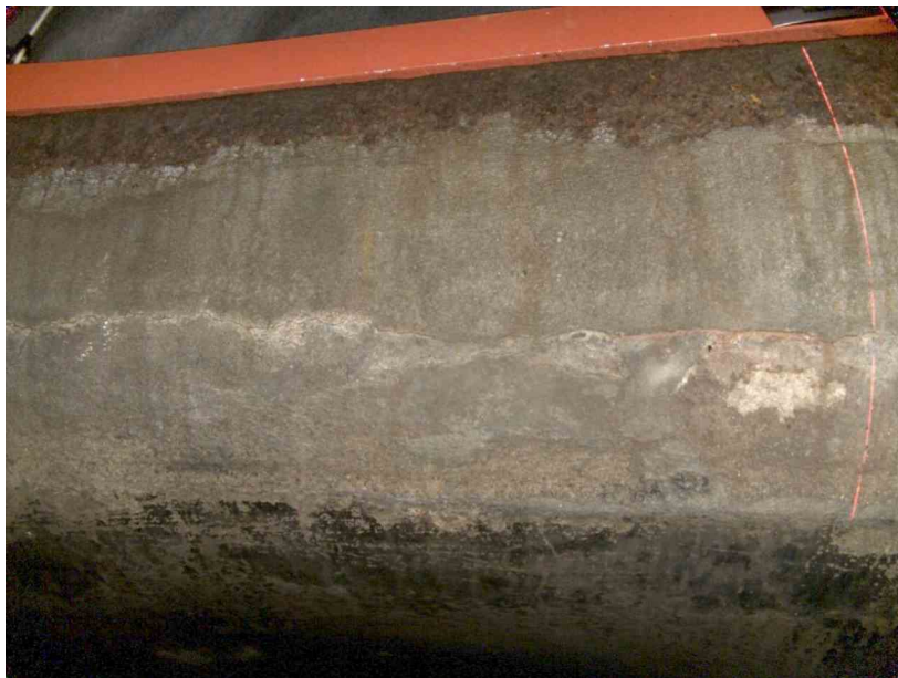
23-01_e8346f74_246f_46bb_9af3_39d1c680baea_0a91a2fe-5873-4644-83be-e99d7e157e37_P12.jpg, , 0.30 Crack Circumferential from 12 o'clock to 12 o'clock, within 8 inch
