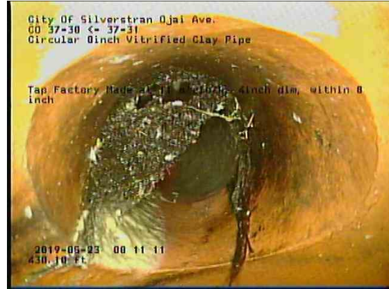
221ccd57-69fc-485b-8100-e8fa6ed67b9a_20190523_081344_119.jpg, 00:27:24, 430.10ft Tap Factory Made at 11 o'clock, 4inch dim, within 8 inch
