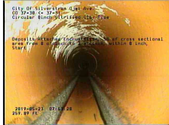
c99fbe0d-9dbf-49b7-bb57-5bda61d5c3b3_20190523_075600_907.jpg, 00:15:03, 259.89ft Deposits Attached Encrustation, 5% of cross sectional area from 8 o'clock to 2 o'clock, within 8 inch, Start
