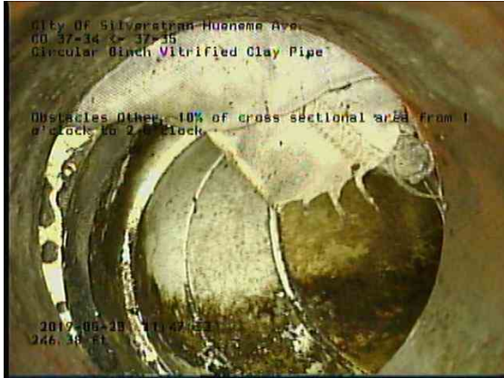
e69da673-911c-4985-a325-4850f98c7e8a_20190523_115006_721.jpg, 00:16:32, 246.38ft Obstacles Other, 10% of cross sectional area from 1 o'clock to 2 o'clock / IN WYE
