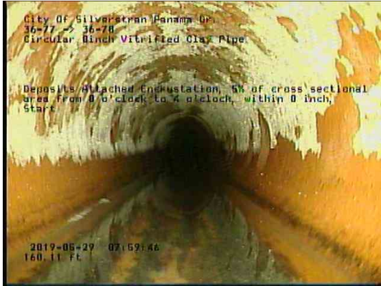
202bbf92-b75d-4a55-aa06-c4bfadd4dd36_20190529_080220_842.jpg, 00:16:46, 160.11ft Deposits Attached Encrustation, 5% of cross sectional area from 8 o'clock to 4 o'clock, within 8 inch, Start
