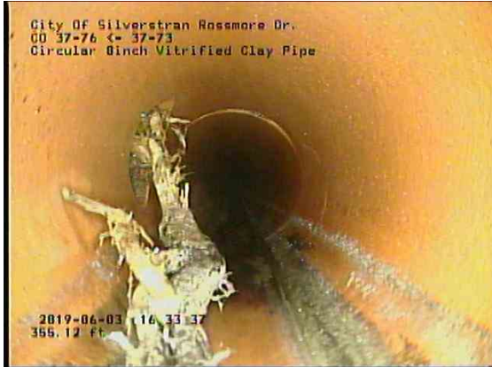
b3d41275-34d8-4d68-a4fd-6e2b020bf2fd_20190603_163614_743.jpg, 00:22:32, 356.62ft Roots Tap Lateral from 9 o'clock to 10 o'clock, 85% of cross sectional area
