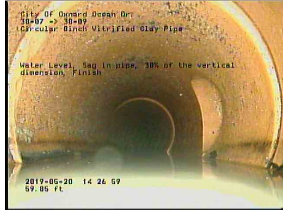
ead8fe43-14b5-4ad4-be9a-3e13f8f0a907_20190520_142929_500.jpg, 00:06:31, 59.85ft Water Level, Sag in pipe, 30% of the vertical dimension, Finish
