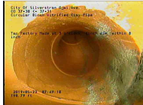
0eb29288-6d88-46c1-82d9-06f83c6f92f5_20190523_075142_546.jpg, 00:11:47, 198.79ft Tap Factory Made at 3 o'clock, 4inch dim, within 8 inch
