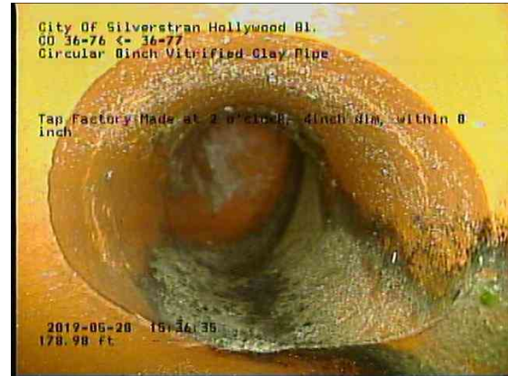
8eeb1b72-5530-446d-8d9b-ff52c1033e47_20190528_153909_515.jpg, 00:09:55, 178.98ft Tap Factory Made at 2 o'clock, 4inch dim, within 8 inch
