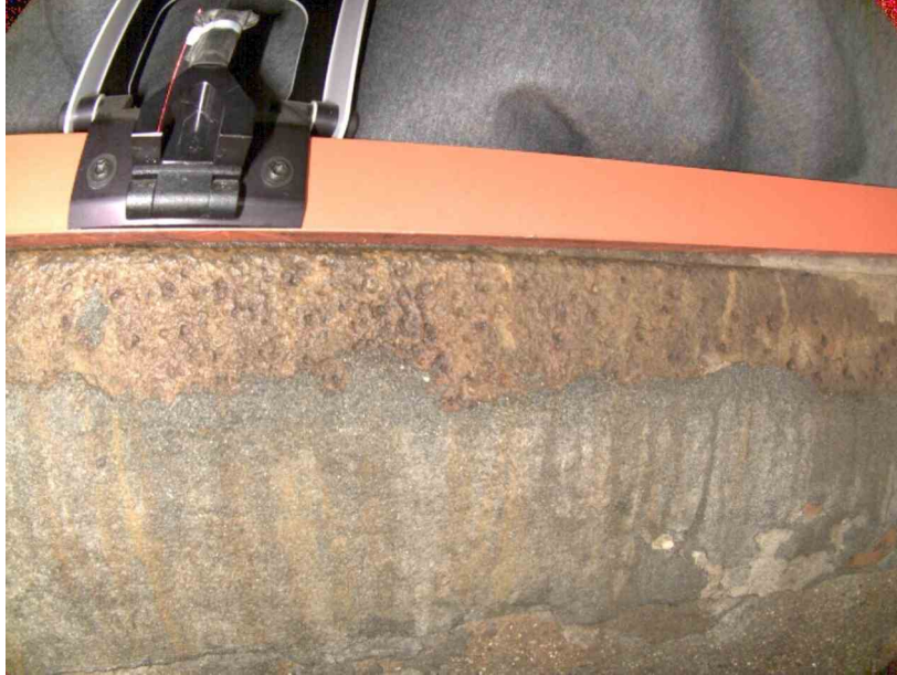
28-09_649da561_021a_4b6c_b8b5_5695380ff438_47b6dd48-897f-4927-b742-b77f48d8bb36_P12.jpg, , 0.03 Surface Roughness Increased, from 06 to -01 o'clock, within 8 inch, S01
