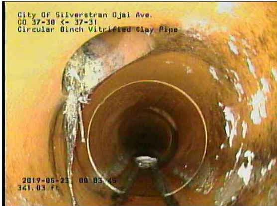
c1c2534d-9fdb-46ed-96d0-d61e8187925f_20190523_080618_319.jpg, 00:21:31, 341.79ft Roots Medium Lateral at 11 o'clock, 25% lost, within 8 inch
