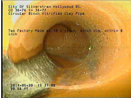
e09e6243-dbc-44b4-a4ac-246994f2f717_20190528_153342_217.jpg, 00:05:10, 98.56ft Tap Factory Made at 10 o'clock, 4inch dim, within 8 inch
