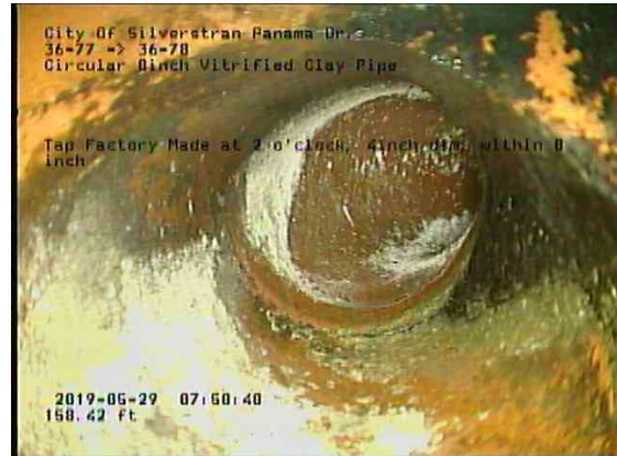
f9722d82-7e21-41c9-a407-e7e08477ee24_20190529_080122_395.jpg, 00:16:19, 158.42ft Tap Factory Made at 2 o'clock, 4inch dim, within 8 inch
