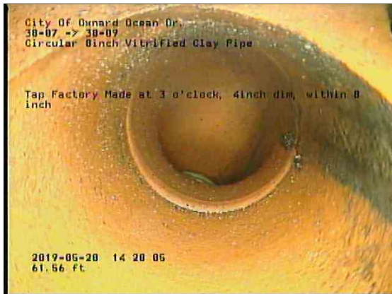
e87c69de-64c6-45a5-a396-160b85ead0c8_20190520_143035_412.jpg, 00:06:35, 61.56ft Tap Factory Made at 3 o'clock, 4inch dim, within 8 inch
