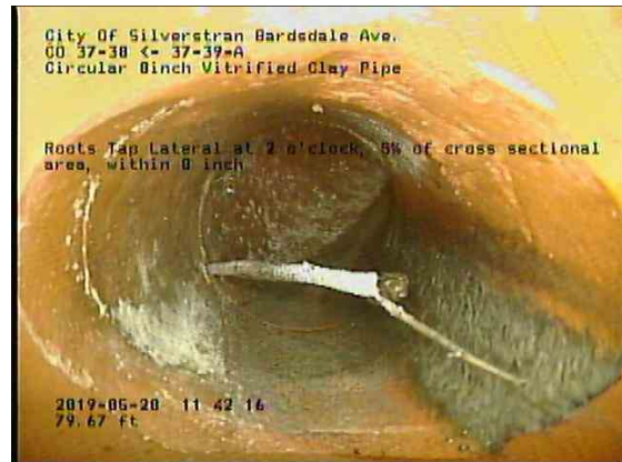
9623719a-cea0-406b-8256-a52497ef9549_20190528_114450_771.jpg, 00:05:33, 79.67ft Roots Tap Lateral at 2 o'clock, 5% of cross sectional area, within 8 inch
