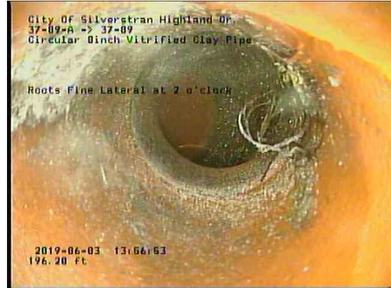
d92a4354-8497-4757-84e2-7a4b652669ef_20190603_135930_171.jpg, 00:19:10, 196.20ft Roots Fine Lateral at 2 o'clock
