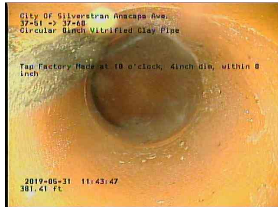
f88a06e0-040c-4880-94de-217867e1c938_20190531_114624_231.jpg, 00:23:24, 381.41ft Tap Factory Made at 10 o'clock, 4inch dim, within 8 inch
