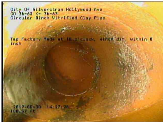
2b435157-b36b-4535-b15c-98131e4b6308_20190530_143001_201.jpg, 00:13:02, 180.57ft Tap Factory Made at 9 o'clock, 4inch dim, within 8 inch
