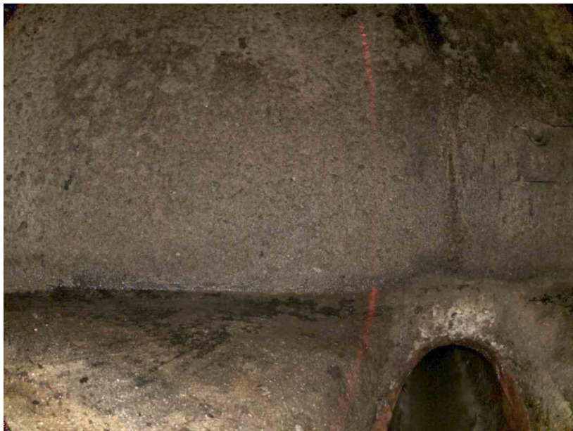
37-89-A_b79949af_46fc_4028_94b0_26ae49ec5641_e4783387-ff88-4695-9728-0f5a51522fba_P12.jpg, , 9.36 Surface Aggregate Visible at 6 o'clock, within 8 inch
