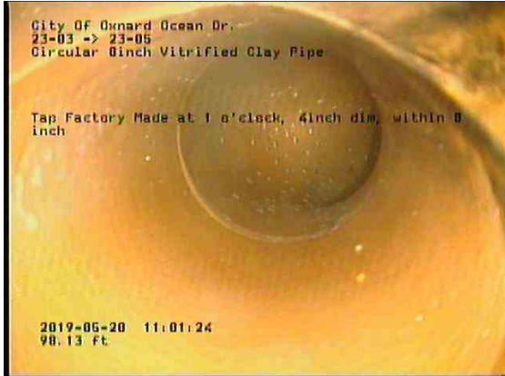
64628eda-a1b0-4364-a563-fc39eaf90479_20190520_110354_636.jpg, 00:06:52, 98.13ft Tap Factory Made at 1 o'clock, 4inch dim, within 8 inch
