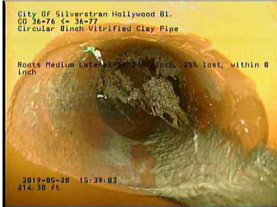
185000c2-3afd-4323-9445-ae5c1f83d867_20190528_154138_071.jpg, 00:11:48, 214.30ft Roots Medium Lateral at 2 o'clock, 25% lost, within 8 inch
