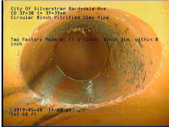
2bb2ed61-0b9d-4bc1-95c5-9c3d1fa144f2_20190528_115222_224.jpg, 00:11:27, 167.58ft Tap Factory Made at 11 o'clock, 4inch dim, within 8 inch
