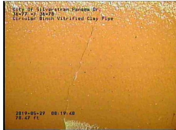
10583926-98e8-4007-b70f-60beb77da837_20190529_082214_837.jpg, 00:06:39, 78.47ft Crack Longitudinal at 3 o'clock, within 8 inch
