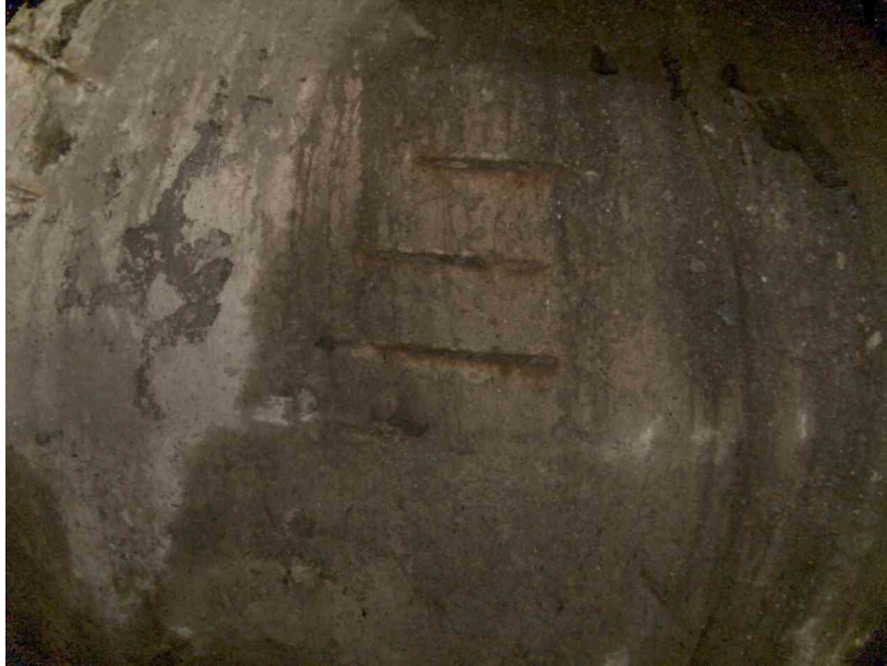
28-09_649da561_021a_4b6c_b8b5_5695380ff438_45944e11-9aa9-4c5e-8023-ea428999f8aa_P12.jpg, , 2.98 Surface Reinforcement Corroded, from 10 to -01 o'clock, within 8 inch
