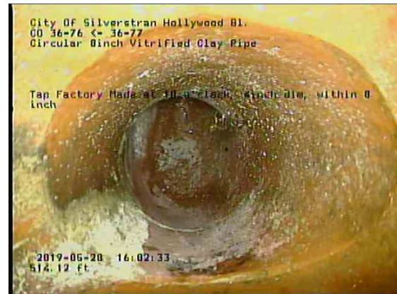
5fe63f10-7af3-4595-a221-a45245c92fca_20190528_160507_596.jpg, 00:30:43, 514.12ft Tap Factory Made at 10 o'clock, 4inch dim, within 8 inch
