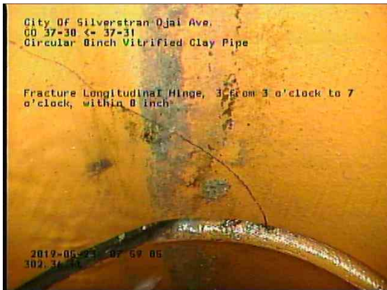
357cfa61-c518-44d1-87ca-3fa53e60bb97_20190523_080137_803.jpg, 00:18:06, 302.36ft Fracture Longitudinal Hinge, 3 from 3 o'clock to 7 o'clock, within 8 inch
