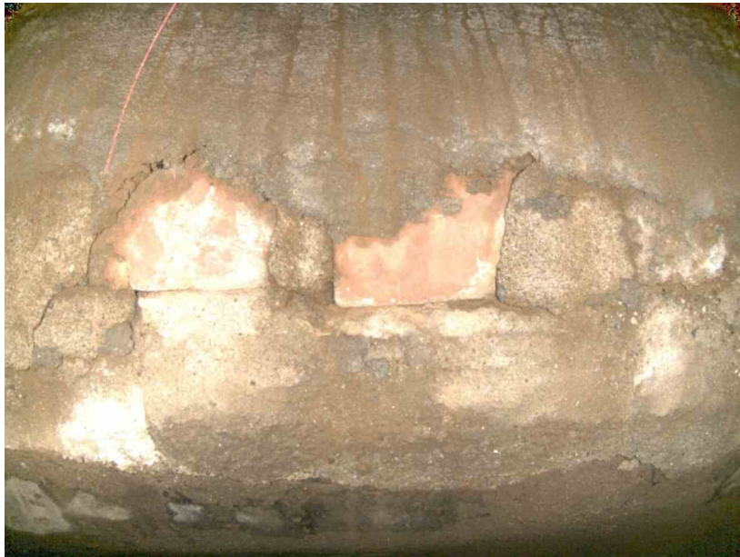
23-03_caf8412c_d397_4fc6_88c9_a9658e397a0b_14a69846-3e4b-43b0-9bb7-fb919f07bbf2_P12.jpg, , 0.40 Surface Roughness Increased, from 08 to -01 o'clock, within 8 inch, S01
