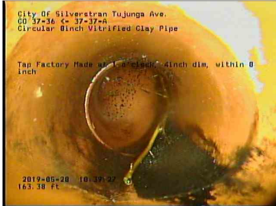
f911bcff-7f1b-4407-9cb1-e9533e1afd5e_20190528_104200_177.jpg, 00:09:47, 163.38ft Tap Factory Made at 1 o'clock, 4inch dim, within 8 inch
