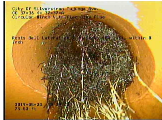
1eabff86-f80b-478c-bac3-c868169d560c_20190528_103315_110.jpg, 00:04:00, 75.52ft Roots Ball Lateral at 2 o'clock, 70% lost, within 8 inch
