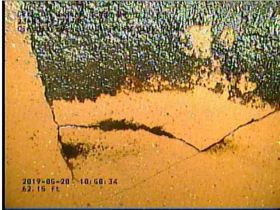
fcc5c6b5-d1ab-4535-8d5c-531b5251c740_20190520_110104_565.jpg, 00:04:07, 62.14ft Crack Longitudinal Hinge, 2 from 2 o'clock to 4 o'clock, within 8 inch
