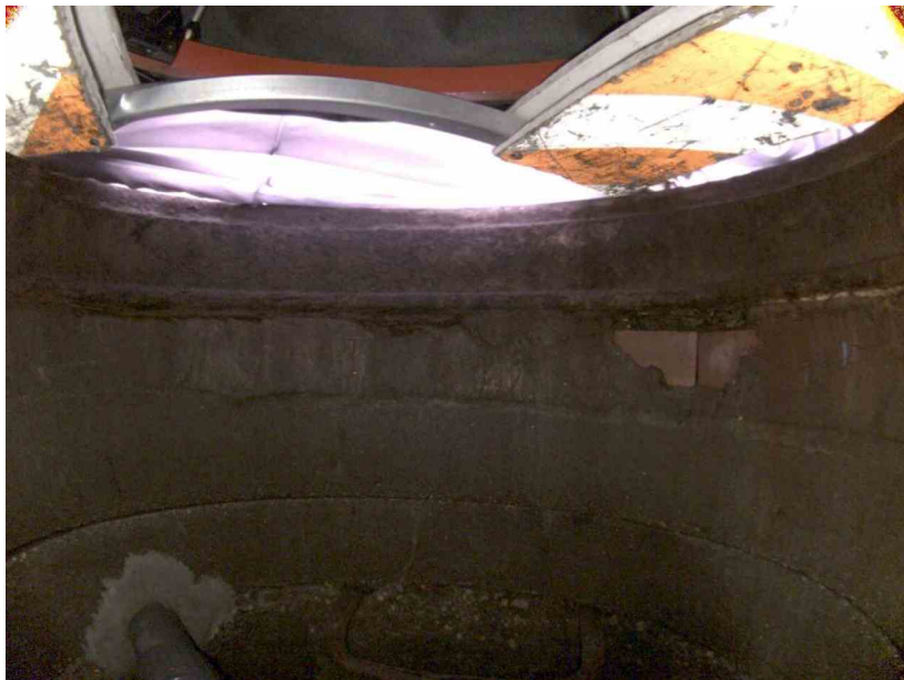
36-82_d8b17f0a_c20d_4a90_8fc5_f6b02c187456_0d644e19-155f-4653-83f7-90f999386221_P12.jpg, , 0.16 Surface Aggregate Missing at 3 o'clock, within 8 inch
