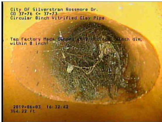
e6c070ec-29ff-4e2a-ae56-c3339a679b76_20190603_163519_172.jpg, 00:22:10, 354.22ft Tap Factory Made Capped at 2 o'clock, 4inch dim, within 8 inch
