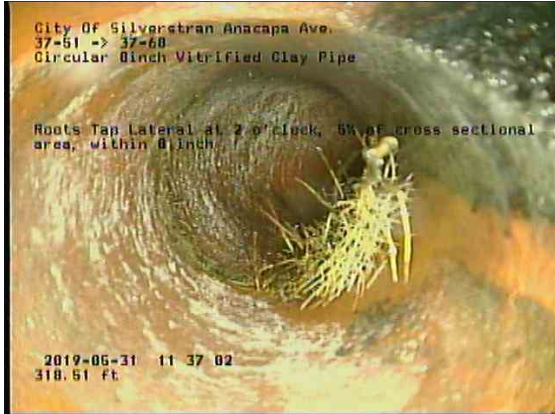
208dd375-5b84-4251-a399-c23cf3a01879_20190531_113939_506.jpg, 00:19:17, 318.51ft Roots Tap Lateral at 2 o'clock, 5% of cross sectional area, within 8 inch
