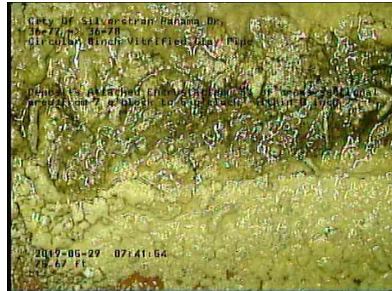
f505f14c-6b5b-4d7b-aaf1-176fb2f33a31_20190529_074428_164.jpg, 00:05:51, 75.64ft Deposits Attached Encrustation, 5% of cross sectional area from 7 o'clock to 5 o'clock, within 8 inch
