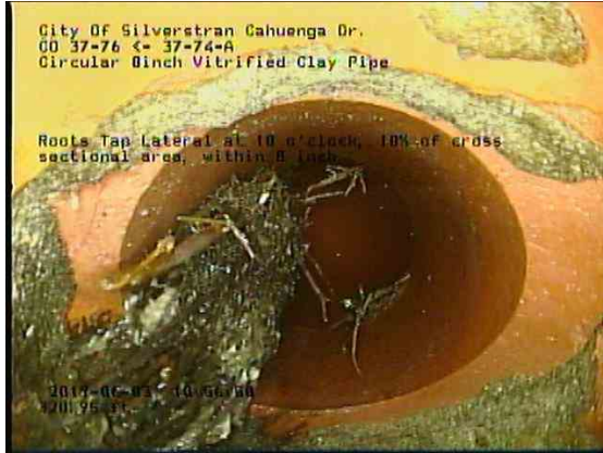
4c6fcb6c-6921-4a2e-9b71-8dbd8a42b66d_20190603_105926_335.jpg, 00:21:14, 320.95ft Roots Tap Lateral at 10 o'clock, 10% of cross sectional area, within 8 inch
