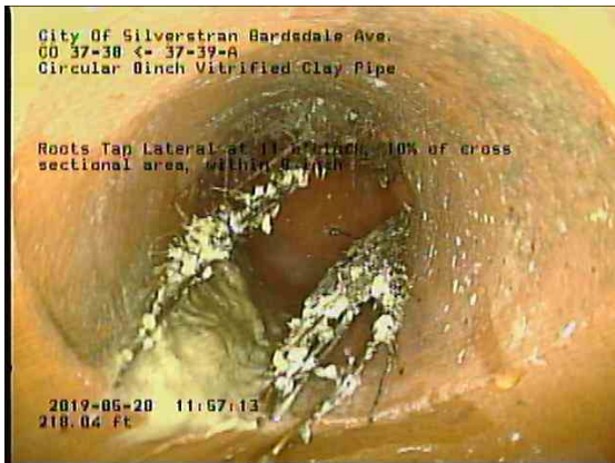
439a2d4f-5019-4ecc-b279-998ea7e268bc_20190528_115947_283.jpg, 00:16:36, 218.04ft Roots Tap Lateral at 11 o'clock, 10% of cross sectional area, within 8 inch
