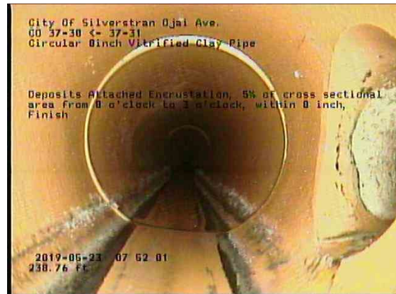
188c21a6-41ca-4a10-b13a-1cdaab6a515b_20190523_075434_363.jpg, 00:13:59, 238.76ft Deposits Attached Encrustation, 5% of cross sectional area from 8 o'clock to 3 o'clock, within 8 inch, Finish
