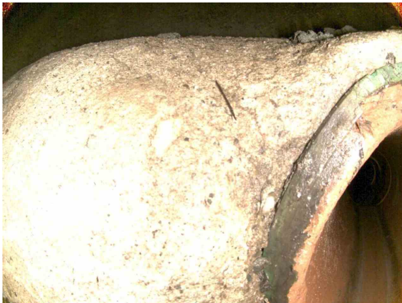
23-01_e8346f74_246f_46bb_9af3_39d1c680baea_e1109055-309b-430d-9a2d-31ce9fce9a0c_P12.jpg, , 6.45 Surface Roughness Increased from 12 o'clock to 12 o'clock, within 8 inch
