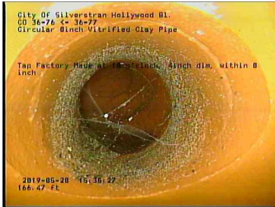
c0e57f1b-6419-48a2-92b9-ad419f0fa96b_20190528_153801_747.jpg, 00:08:56, 166.47ft Tap Factory Made at 10 o'clock, 4inch dim, within 8 inch
