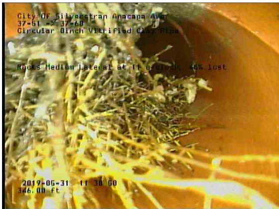
63aec12c-723f-490b-8d1c-566042ae6ff6_20190531_114126_890.jpg, 00:20:41, 346.00ft Roots Medium Lateral at 11 o'clock, 45% lost
