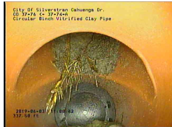
e2f09161-3a81-41c2-a90f-ae41d375e78e_20190603_110318_308.jpg, 00:23:08, 338.27ft Cleanout Mainline / CO 37-76
