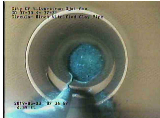
73a19e65-5d4e-44b2-9f48-91d79a1d8d99_20190523_073930_278.jpg, 00:02:11, 0.46ft Tap Factory Made at 6 o'clock, 8inch dim, within 8 inch
