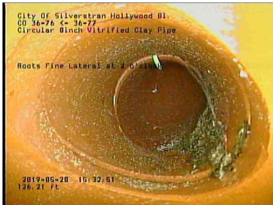
26f58a61-35e5-4ed6-8018-14b1d66e5b3f_20190528_153526_108.jpg, 00:06:36, 126.21ft Roots Fine Lateral at 2 o'clock
