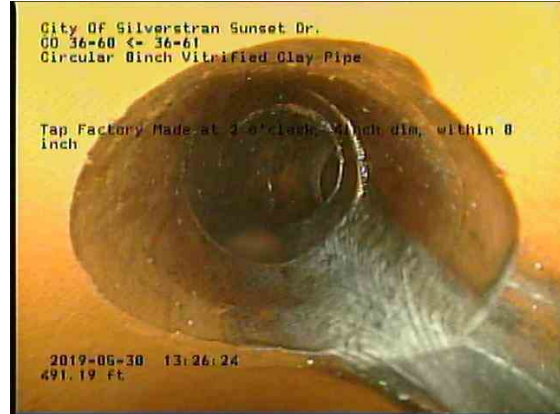
d2426945-55c6-4208-8de4-900754de15f3_20190530_132859_775.jpg, 00:27:14, 491.18ft Tap Factory Made at 2 o'clock, 4inch dim, within 8 inch
