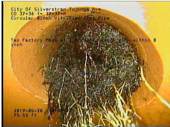
c2f82421-43da-46f3-983f-ec4d492fd609_20190528_103300_469.jpg, 00:03:57, 75.52ft Tap Factory Made at 2 o'clock, 4inch dim, within 8 inch
