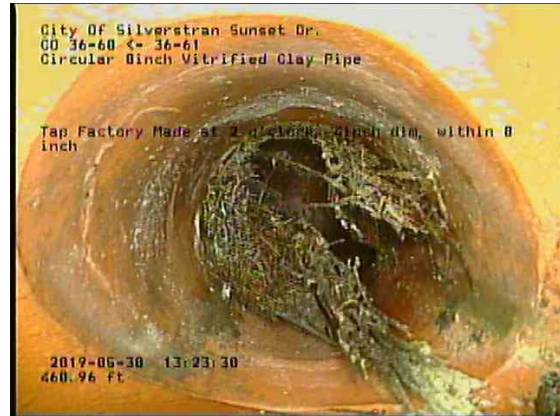
55d46e42-0cbe-4326-9fa2-0c4cb29b31c5_20190530_132605_536.jpg, 00:25:24, 460.96ft Tap Factory Made at 2 o'clock, 4inch dim, within 8 inch
