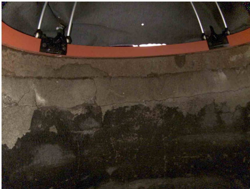
37-74-A_b7daeb13_42d1_4279_a6a1_58685002b84e_45779d46-ff56-4f6b-949a-5e76576667d8_PL12.jpg, , 0.10 Crack Circumferential from 1 o'clock to 5 o'clock, within 8 inch
