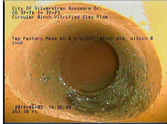
52a55016-0b53-4851-9004-23d958f55695_20190603_162817_744.jpg, 00:16:08, 253.30ft Tap Factory Made at 2 o'clock, 4inch dim, within 8 inch
