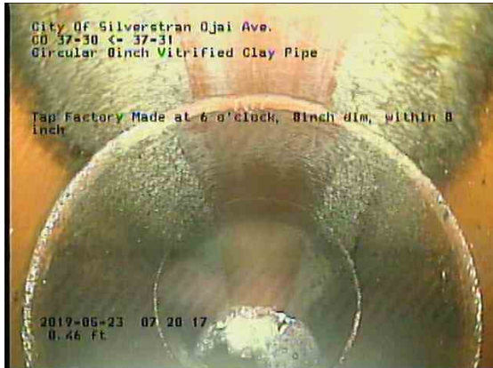
86ebb2ad-0484-470c-92b2-7f2d3cecff6f_20190523_073050_177.jpg, 00:02:11, 0.46ft Tap Factory Made at 6 o'clock, 8inch dim, within 8 inch
