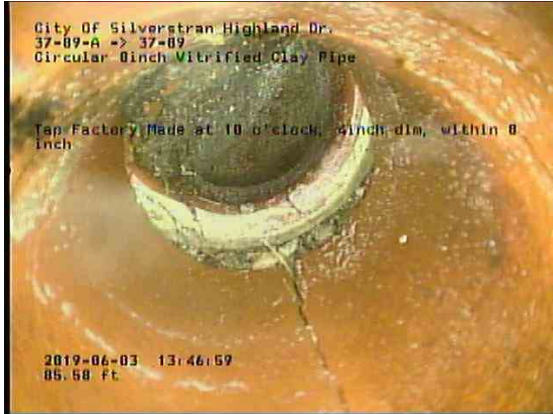
0b5cfe83-87f8-4c54-a294-e0fa3ba0a0eb_20190603_134936_587.jpg, 00:10:54, 85.58ft Tap Factory Made at 10 o'clock, 4inch dim, within 8 inch
