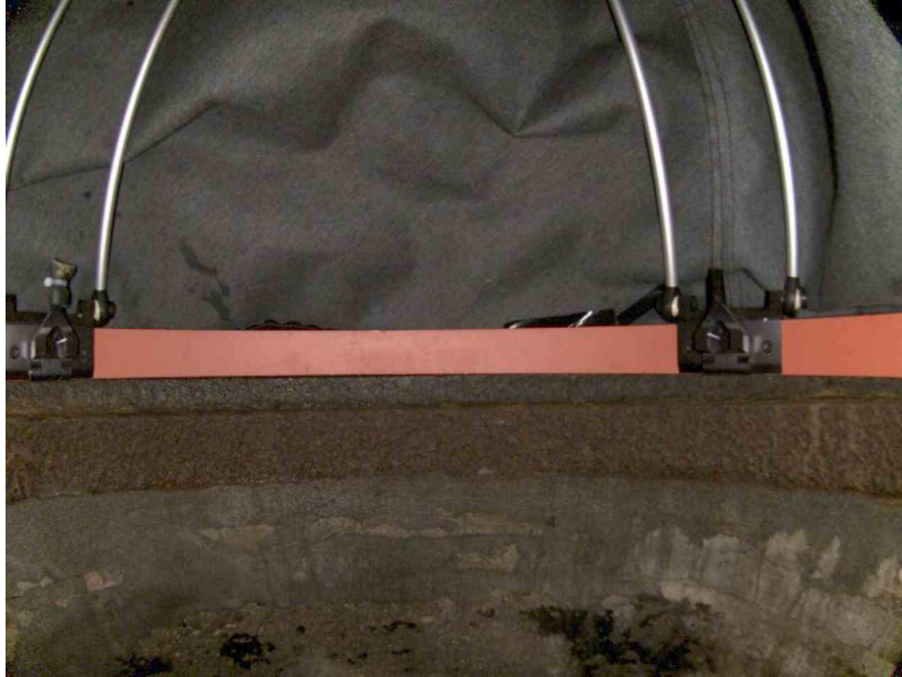
37-39_e3463806_251b_4a10_8598_66aa7b2b50ab_a542e92e-682c-4f5c-a856-3c2bc2bf61a5_P12.jpg, , -0.62 Reversal Inspection
