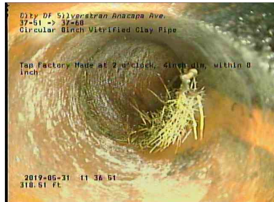
ce85b232-ebb2-4f2d-a674-859966ea95f6_20190531_113927_103.jpg, 00:19:15, 318.51ft Tap Factory Made at 2 o'clock, 4inch dim, within 8 inch
