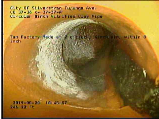
a39a7575-2463-43d1-b3db-ef39731ab5f0_20190528_104830_496.jpg, 00:14:30, 246.22ft Tap Factory Made at 2 o'clock, 4inch dim, within 8 inch
