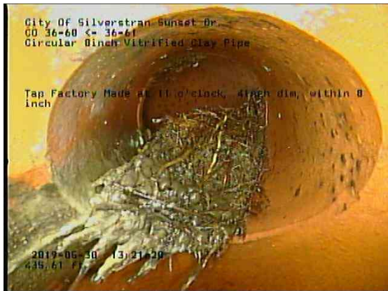
8944d6e5-3e9c-40c9-9c46-ae3f80b41f48_20190530_132355_821.jpg, 00:23:59, 435.61ft Tap Factory Made at 11 o'clock, 4inch dim, within 8 inch
