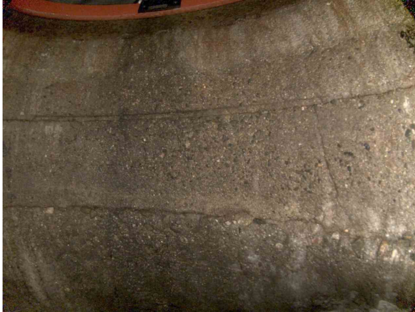
36-61_cd22f785_8cc2_4e9f_ab8d_76fe60c0a5c6_b460dca5-b116-401f-8542-ed9b64b2c492_P12.jpg, , 0.75 Crack Longitudinal at 3 o'clock, within 8 inch
