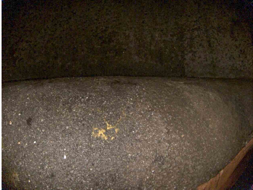
36-63_91085e16_b10b_42df_8305_4acc6363b0ef_106fe174-0aa6-45b6-b675-8d3bbcd553b8_P12.jpg, , 8.99 Surface Roughness Increased from 12 o'clock to 12 o'clock, within 8 inch, Finish
