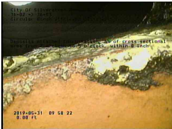
bd87fbb8-09cd-4665-a4cb-acc04b508233_20190531_100058_766.jpg, 00:00:50, 0.00ft Deposits Attached Encrustation, 5% of cross sectional area from 7 o'clock to 5 o'clock, within 8 inch
