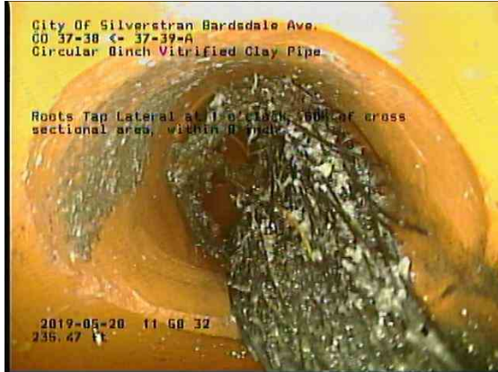
3fbe4892-5f24-4b27-a57b-3c3ca77a4214_20190528_120106_688.jpg, 00:17:27, 235.47ft Roots Tap Lateral at 1 o'clock, 50% of cross sectional area, within 8 inch
