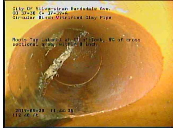
70ee7421-d518-4631-855f-44b290d85c19_20190528_114659_147.jpg, 00:07:19, 112.40ft Roots Tap Lateral at 11 o'clock, 5% of cross sectional area, within 8 inch
