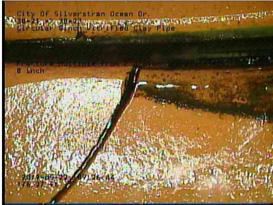
d7c08aa0-b28f-4676-a923-41e2a1677904_20190522_092915_187.jpg, 00:11:15, 176.27ft Fracture Multiple from 7 o'clock to 2 o'clock, within 8 inch
