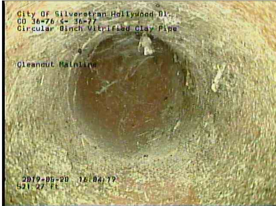
4a09cf2d-b8ac-4a08-ae42-07648ef3d65c_20190528_160654_013.jpg, 00:31:41, 521.27ft Cleanout Mainline / CO 36-76
