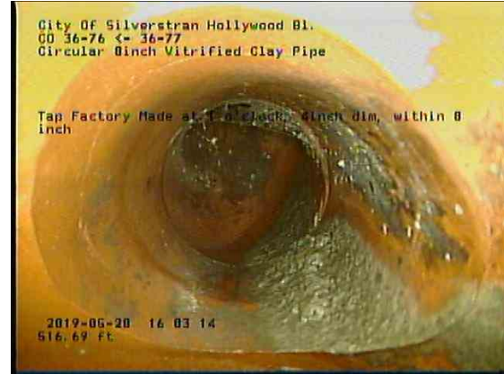
205f4e36-3f87-4da0-a2cd-d8f7be74d2a3_20190528_160548_927.jpg, 00:31:08, 516.69ft Tap Factory Made at 1 o'clock, 4inch dim, within 8 inch
