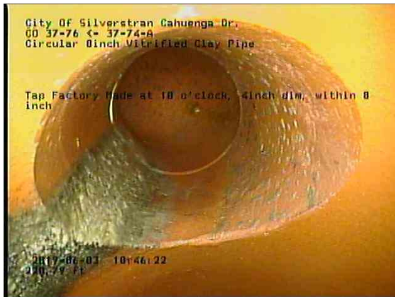
a57c0766-4221-490e-9789-87899798aef3_20190603_104858_452.jpg, 00:14:49, 220.78ft Tap Factory Made at 10 o'clock, 4inch dim, within 8 inch
