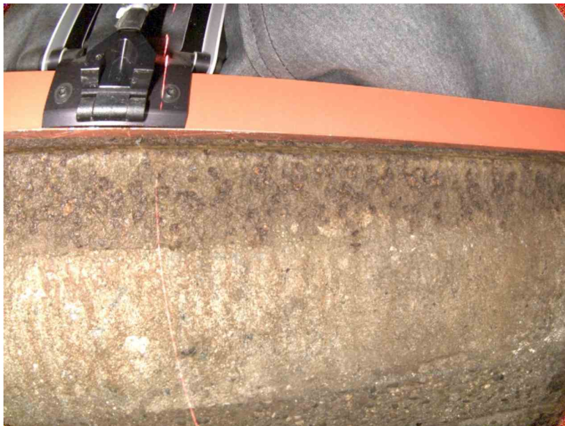
36-61_cd22f785_8cc2_4e9f_ab8d_76fe60c0a5c6_f381b45e-8070-4224-a25f-4b3e7d0261ed_P12.jpg, , 0.00 Surface Roughness Increased from 12 o'clock to 12 o'clock, within 8 inch, Start
