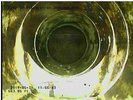
883dfe1e-52ef-4e5b-8f8a-82dda1d66682_20190531_115820_366.jpg, 00:33:35, 554.47ft Tee Connection at 6 o'clock, 8"inch vertical, 8"inch horizontal
