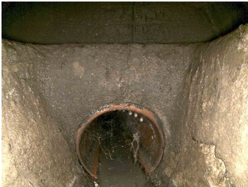
36-77_0025346e_a47e_4222_b655_3956a2432d2c_77e5ec00-e6ee-4b58-9de2-7dbc3d7dad61_P12.jpg, , 6.39 Crack Longitudinal at 1 o'clock, within 8 inch
