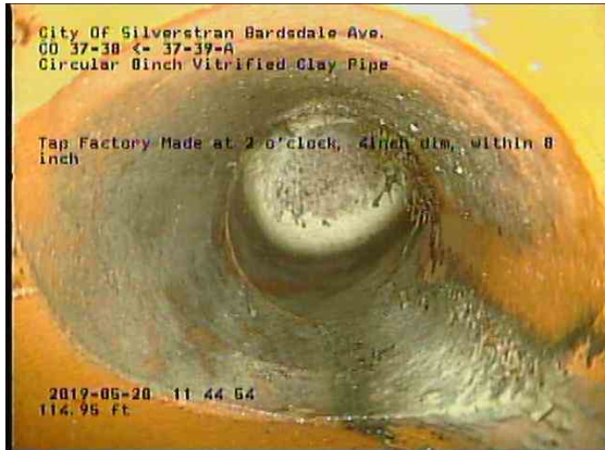
fa26ab0f-5f2b-410b-9a3f-a614bba6f010_20190528_114728_314.jpg, 00:07:39, 114.95ft Tap Factory Made at 2 o'clock, 4inch dim, within 8 inch
