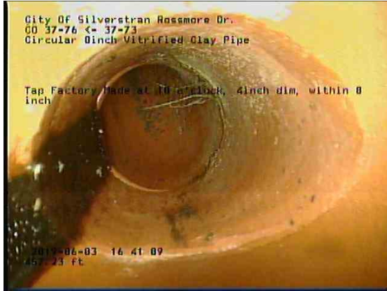
113c0a90-14ef-4729-8e90-fcbf6806e4a1_20190603_164346_150.jpg, 00:28:49, 457.23ft Tap Factory Made at 10 o'clock, 4inch dim, within 8 inch
