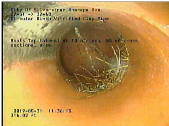
2340189d-11fe-40d4-81e9-ed38f640c8e4_20190531_113852_557.jpg, 00:18:50, 316.02ft Roots Tap Lateral at 10 o'clock, 5% of cross sectional area
