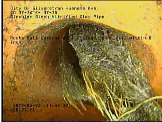
a1d3bb1c-70e1-4a05-afee-932a611d2749_20190523_120212_680.jpg, 00:26:55, 430.22ft Roots Ball Lateral at 1 o'clock, 65% lost, within 8 inch
