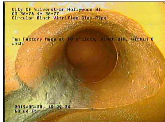
f391f559-5e3e-4aa4-9126-b2cbfaba2d73_20190528_153158_756.jpg, 00:03:35, 60.64ft Tap Factory Made at 10 o'clock, 4inch dim, within 8 inch
