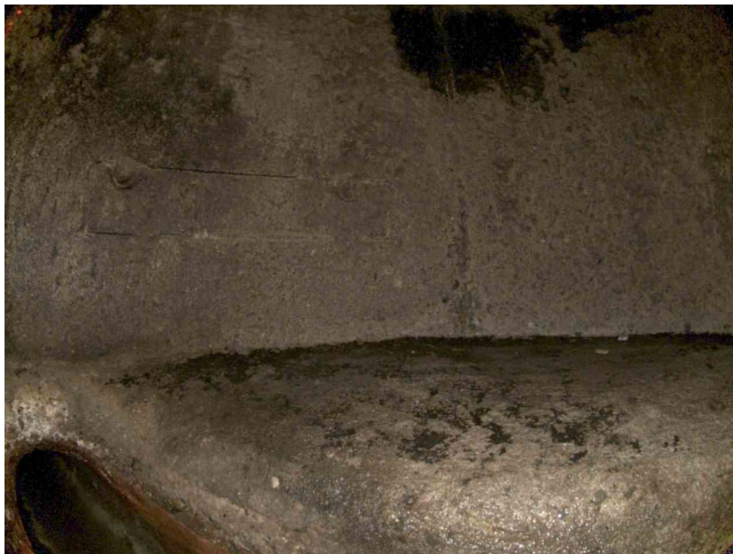
37-89-A_b79949af_46fc_4028_94b0_26ae49ec5641_a945008b-5325-4d7e-8664-792337a22581_P12.jpg, , 9.72 Surface Roughness Increased from 12 o'clock to 12 o'clock, within 8 inch, Finish
