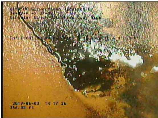
6f9dbcf8-2629-4335-9bc7-64cca41c0594_20190603_142003_529.jpg, 00:32:12, 366.88ft Infiltration Weeper from 3 o'clock to 4 o'clock
