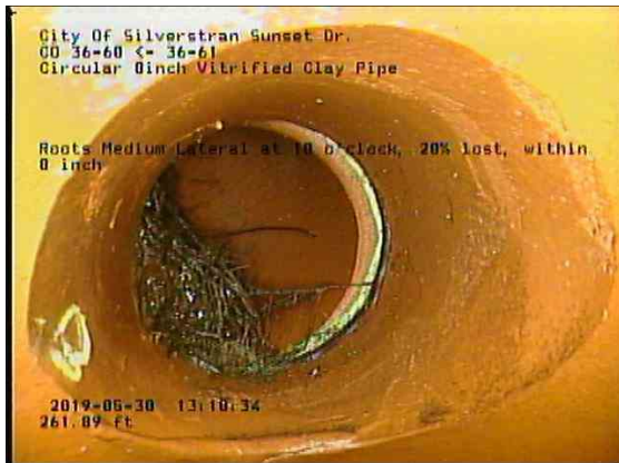
e58061f2-cec8-4652-ac6c-efc3bcdeccef_20190530_131309_970.jpg, 00:14:55, 261.89ft Roots Medium Lateral at 10 o'clock, 20% lost, within 8 inch
