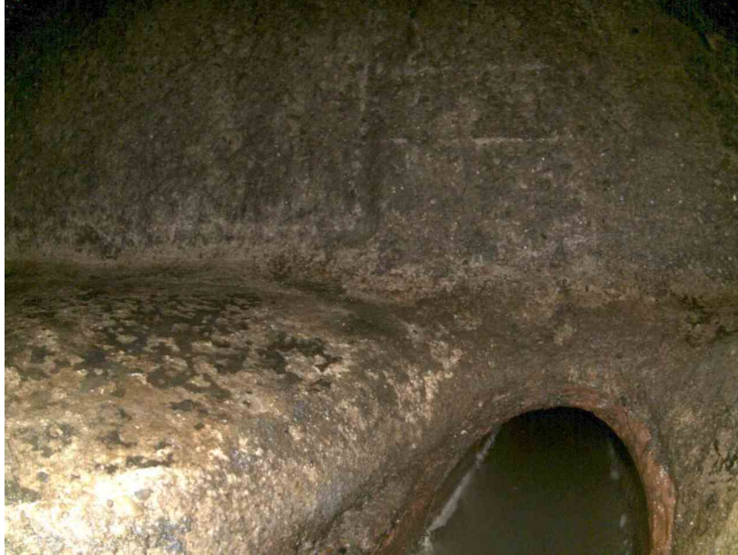
38-21_d8133f19_15ad_4f3f_8ad3_1a1fbd3e9bcc_7d94c4b9-1f0e-4e30-b78c-a42c2e01df47_P12.jpg, , 6.86 Surface Roughness Increased from 12 o'clock to 12 o'clock, within 8 inch, Finish
