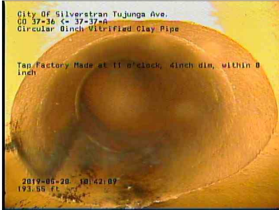
35227d7a-57ef-4e02-bf0c-b969ee44b11_20190528_104442_183.jpg, 00:11:31, 193.55ft Tap Factory Made at 11 o'clock, 4inch dim, within 8 inch
