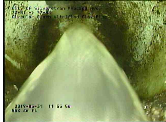
faaac870-5ef5-464f-ba7a-f2ee1add9107_20190531_115833_033.jpg, 00:33:35, 554.47ft Tee Connection at 6 o'clock, 8"inch vertical, 8"inch horizontal
