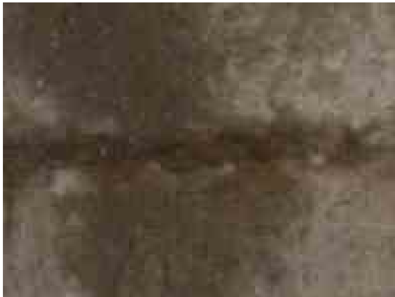
28-09_649da561_021a_4b6c_b8b5_5695380ff438_bbc57b83-8037-4a5b-8b09-f94d6c96ff7a_P11.jpg, , 3.01 Surface Reinforcement Corroded, from 04 to -01 o'clock, within 8 inch
