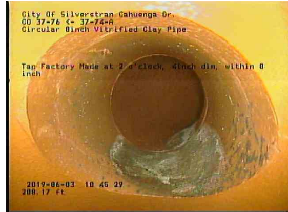
b6ee990d-490f-4579-b56e-d3a5621cdf01_20190603_104805_186.jpg, 00:14:07, 208.17ft Tap Factory Made at 2 o'clock, 4inch dim, within 8 inch
