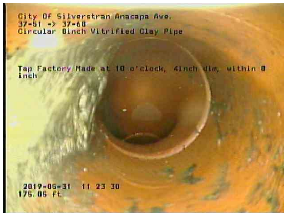
2fe60ae8-e01e-40f6-974f-0f6aa2a65d86_20190531_112607_372.jpg, 00:08:58, 175.05ft Tap Factory Made at 10 o'clock, 4inch dim, within 8 inch
