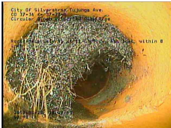
de9e618e-7430-4cba-8592-b36071f867ae_20190528_103146_829.jpg, 00:02:57, 57.90ft Roots Ball Lateral at 11 o'clock, 65% lost, within 8 inch
