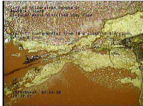
10b32819-2ad5-4c11-bc3d-bf25e90cbf2e_20190529_075654_604.jpg, 00:13:23, 117.39ft Crack Circumferential from 10 o'clock to 1 o'clock, within 8 inch
