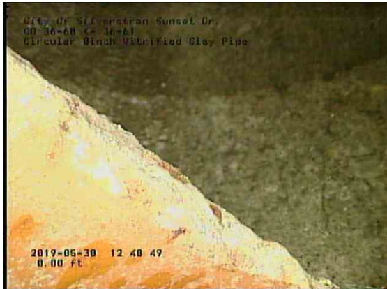
2208eff4-8889-4c5a-bf8e-90ffd584196d_20190530_125124_883.jpg, 00:00:35, 0.00ft Broken from 10 o'clock to 4 o'clock
