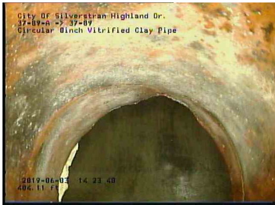
7e12b2ae-0fa3-40ed-af84-c8a30ed615b9_20190603_142625_037.jpg, 00:36:38, 404.11ft Crack Circumferential from 8 o'clock to 4 o'clock, within 8 inch
