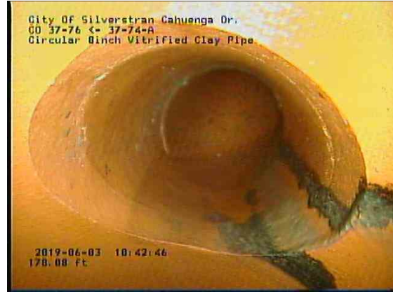
ee68511e-1e23-40e2-b6ef-44bf940c8785_20190603_104522_865.jpg, 00:12:25, 178.08ft Tap Factory Made at 2 o'clock, 4inch dim, within 8 inch
