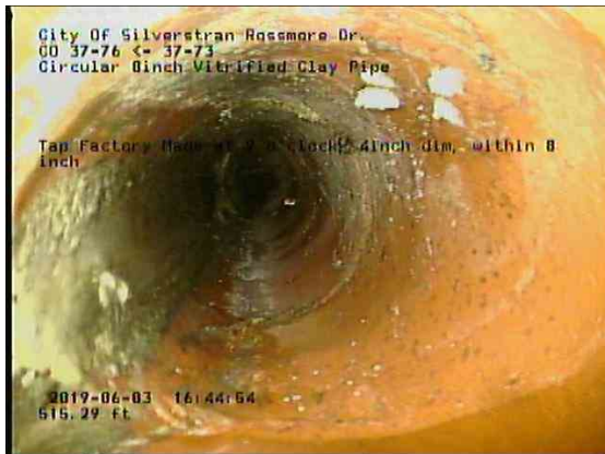
0cd1cbcc-0c14-475d-9153-6230ba0c3168_20190603_164731_709.jpg, 00:31:50, 515.29ft Tap Factory Made at 9 o'clock, 4inch dim, within 8 inch
