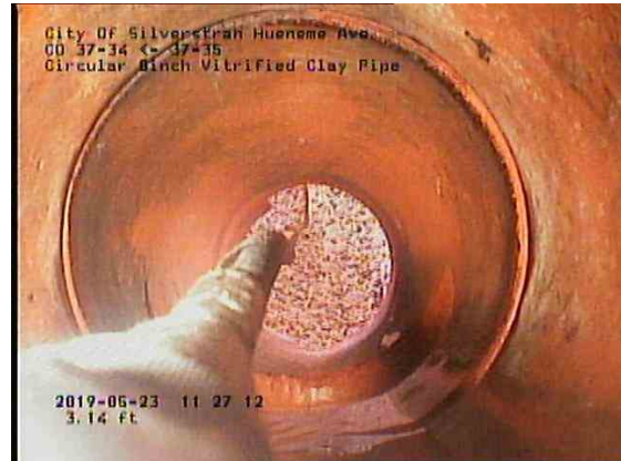
d0c59d53-4f3f-4166-a27a-8aaef57d6b7_20190523_112945_730.jpg, 00:00:56, 0.52ft Tap Factory Made at 6 o'clock, 8inch dim, within 8 inch
