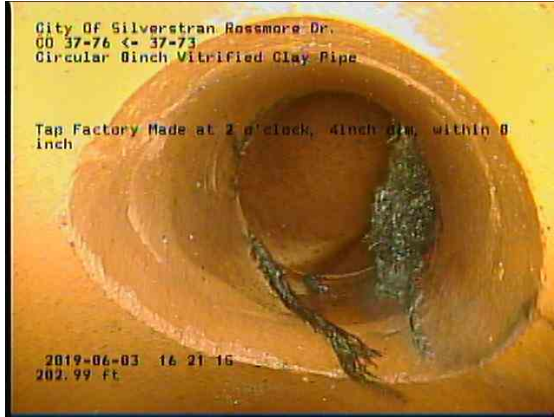
553975f3-0d33-4c8e-ab3b-8053f5930c58_20190603_162352_981.jpg, 00:12:59, 202.99ft Tap Factory Made at 2 o'clock, 4inch dim, within 8 inch
