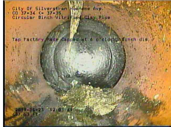
cbf28fd8-eb39-414d-a87d-bb2eb2df8c88_20190523_120622_846.jpg, 00:29:26, 437.53ft Tap Factory Made Capped at 6 o'clock, 8inch dim
