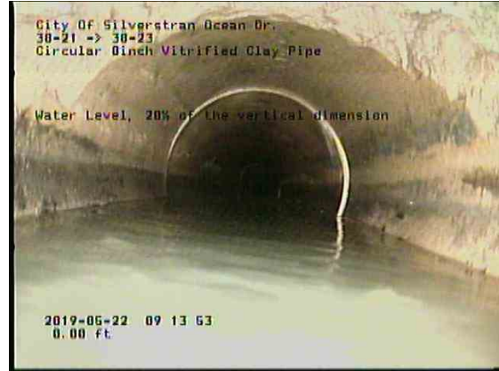
802ed06c-7377-4231-b918-7ca7edcb3199_20190522_091624_649.jpg, 00:00:11, 0.00ft Water Level, 20% of the vertical dimension
