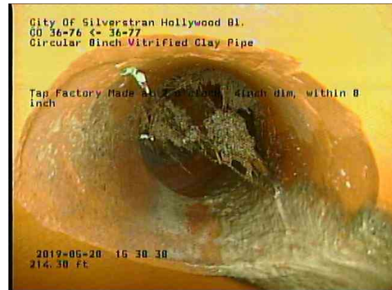
19541ddd-3206-46c6-ac2b-8f8ea1eb302b_20190528_154112_823.jpg, 00:11:44, 214.30ft Tap Factory Made at 2 o'clock, 4inch dim, within 8 inch
