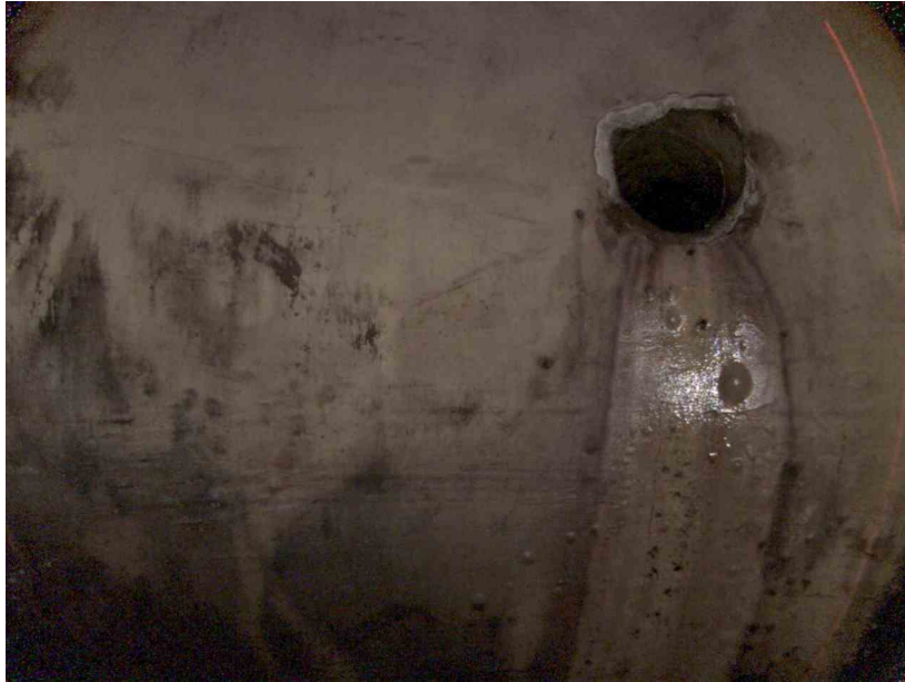
37-89_b7b73460_144a_4a36_a05d_2d26ddf59287_9894b9ec-1349-4f86-a48a-e26b06d462bb_P12.jpg, , 6.62 Lining Failure Blistered at 9 o'clock, within 8 inch
