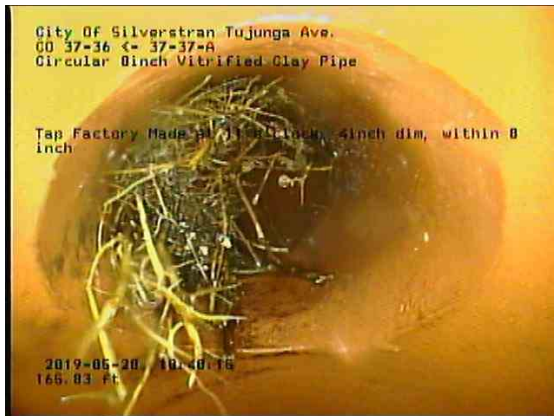
259f230c-15c6-4d42-a3d0-dec16efbad22_20190528_104248_954.jpg, 00:10:10, 165.83ft Tap Factory Made at 11 o'clock, 4inch dim, within 8 inch
