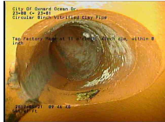
77c2eb96-0959-4b44-9300-169a166df241_20190521_094910_742.jpg, 00:29:17, 555.41ft Tap Factory Made at 11 o'clock, 4inch dim, within 8 inch
