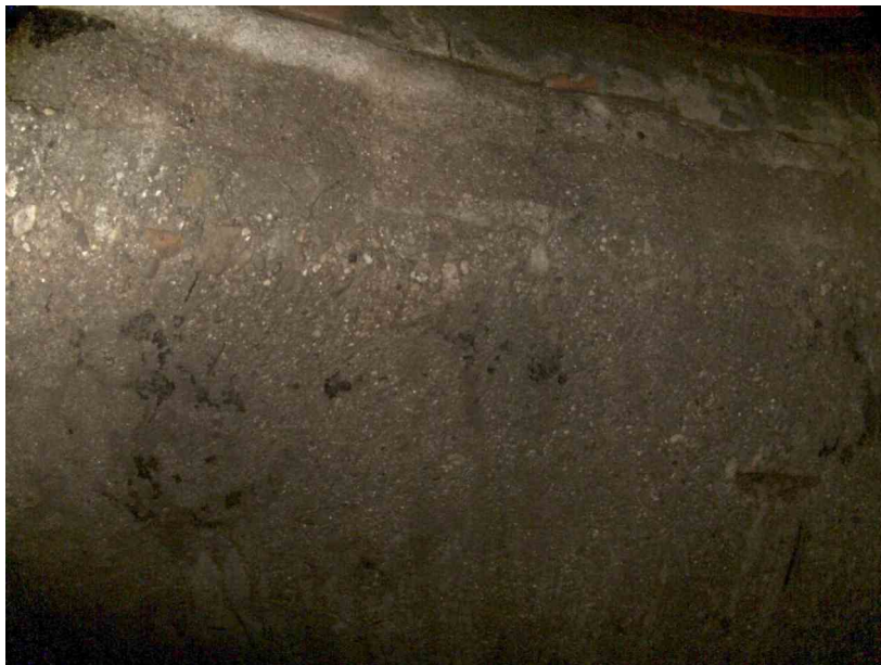
23-05_07f89197_7dd0_4207_a0d5_4ab641627b63_df37b7ec-0ba7-4166-b649-d9fde31d91b6_P12.jpg, , 1.28 Surface Reinforcement Corroded at 11 o'clock, within 8 inch
