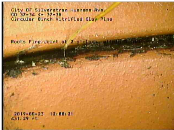
b0fa45fe-046c-413d-bba5-de3570ca966c_20190523_120254_872.jpg, 00:27:28, 431.29ft Roots Fine Joint at 2 o'clock, within 8 inch
