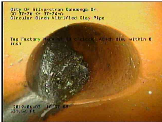
0de055f5-2654-4959-b198-457ee7377040_20190603_110035_876.jpg, 00:22:05, 331.54ft Tap Factory Made at 10 o'clock, 4inch dim, within 8 inch
