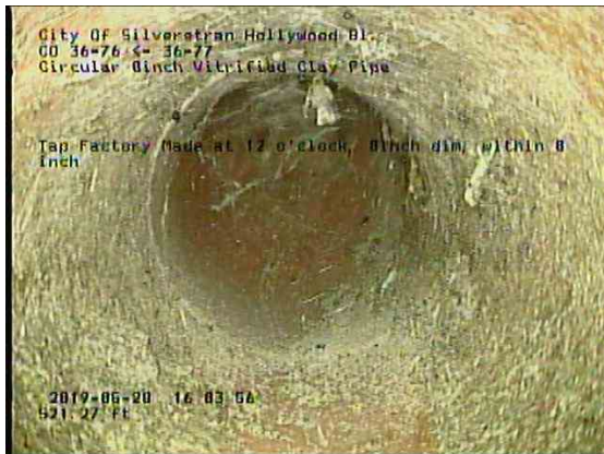
e963faff-8528-4596-950c-4c671c94368b_20190528_160630_275.jpg, 00:31:38, 521.27ft Tap Factory Made at 12 o'clock, 8inch dim, within 8 inch
