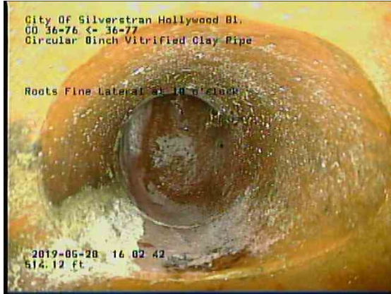
fa9d8b08-818f-4138-8a76-31c5955e51e4_20190528_160517_022.jpg, 00:30:45, 514.12ft Roots Fine Lateral at 10 o'clock
