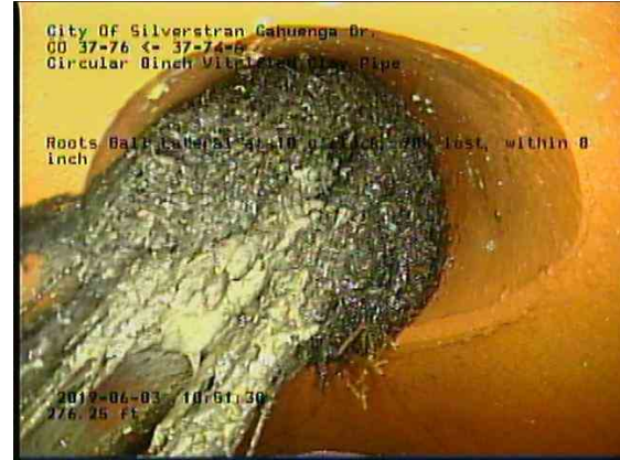
5a55c837-4dce-469d-884a-cca8959da58a_20190603_105406_262.jpg, 00:17:53, 276.25ft Roots Ball Lateral at 10 o'clock, 90% lost, within 8 inch
