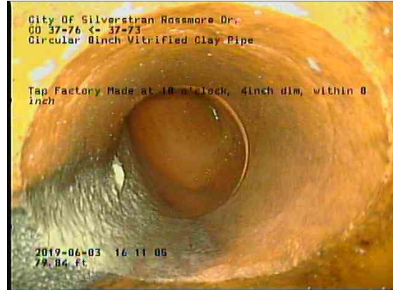
6b798b55-bc68-4acb-8005-21b54d84eafd_20190603_161342_919.jpg, 00:04:53, 79.84ft Tap Factory Made at 10 o'clock, 4inch dim, within 8 inch
