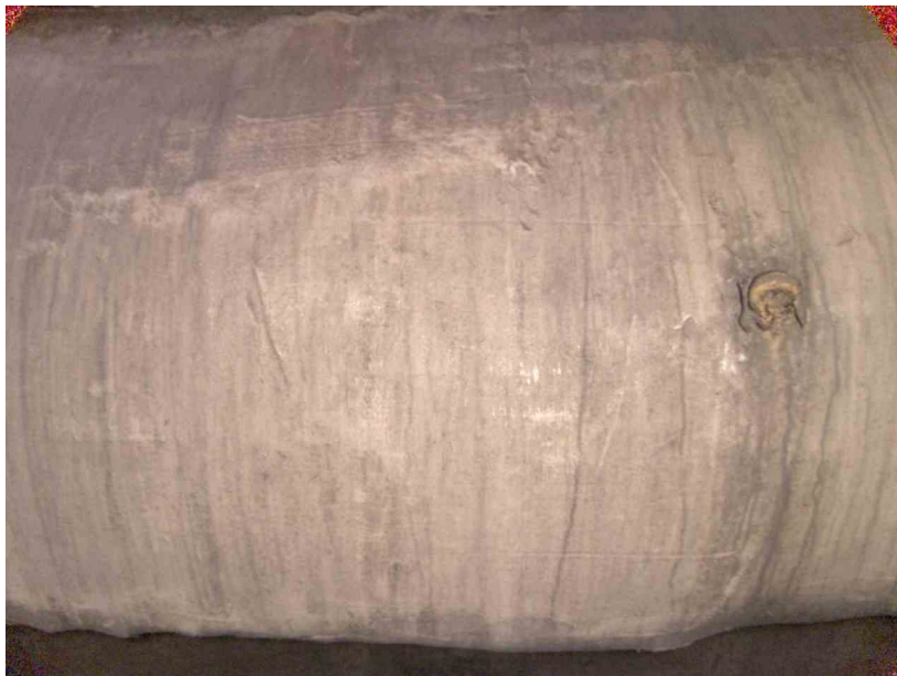
37-89_b7b73460_144a_4a36_a05d_2d26ddf59287_4b2498f2-a6f4-40ea-a2fd-8922a026abcd_P12.jpg, , 1.09 Lining Failure Delaminating at 7 o'clock, within 8 inch
