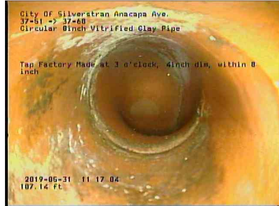
debdce89-2e68-45f8-b371-1e600aa8b477_20190531_111941_465.jpg, 00:05:00, 107.14ft Tap Factory Made at 3 o'clock, 4inch dim, within 8 inch
