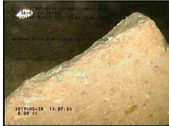
049f7848-bfcf-4778-9f44-0f4429b35483_20190530_140959_798.jpg, 00:00:35, 0.00ft Broken from 7 o'clock to 4 o'clock
