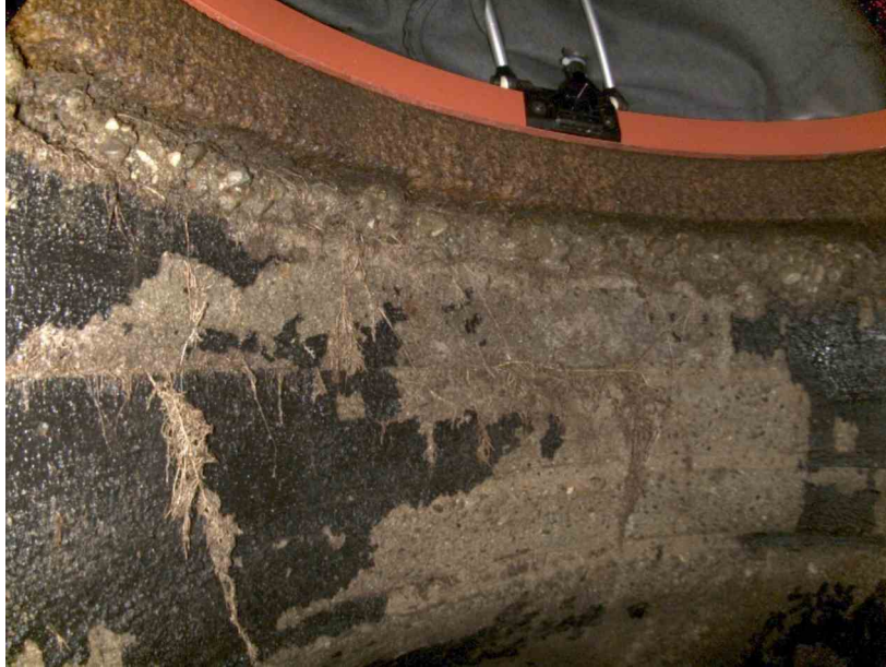
37-89-A_b79949af_46fc_4028_94b0_26ae49ec5641_8a0b00ee-7a80-43b3-819d-5ee4896b024f_P12.jpg, , 0.55 Roots Fine Joint at 11 o'clock, within 8 inch
