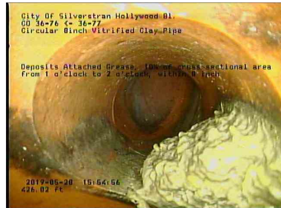
7b518f61-f80f-4c11-8bac-601964c6675e_20190528_155729_472.jpg, 00:25:06, 426.02ft Deposits Attached Grease, 10% of cross sectional area from 1 o'clock to 2 o'clock, within 8 inch / In WYE
