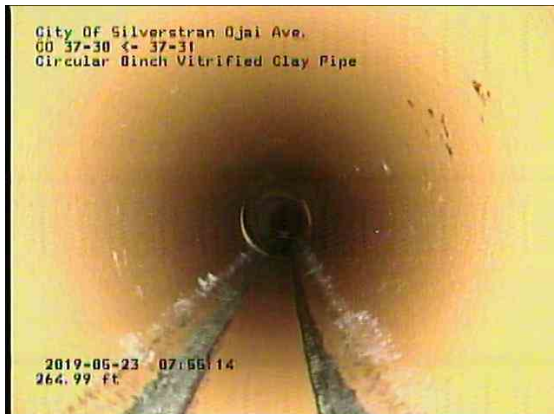
0137e18f-bed0-43af-b6ff-637721f8e659_20190523_075746_976.jpg, 00:15:25, 264.98ft Deposits Attached Encrustation, 5% of cross sectional area from 8 o'clock to 2 o'clock, within 8 inch, Finish
