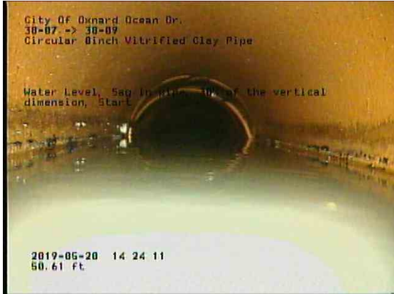
22f3dc8c-0bf7-4c0a-8485-e0b1e5a0f22e_20190520_142641_786.jpg, 00:04:42, 50.61ft Water Level, Sag in pipe, 30% of the vertical dimension, Start
