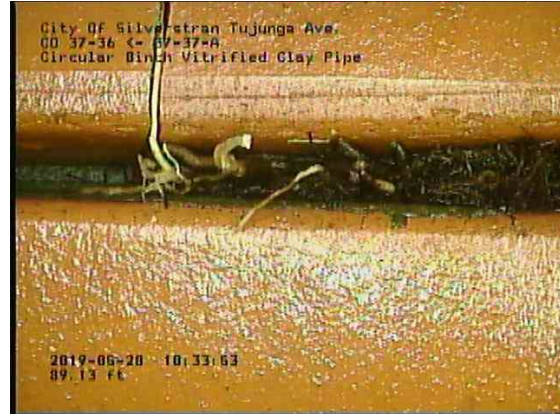
d55b6651-9f25-4b2e-8ba0-c2e6b7e156d2_20190528_103626_303.jpg, 00:05:50, 89.13ft Roots Tap Joint from 3 o'clock to 5 o'clock, 5% of cross sectional area, within 8 inch
