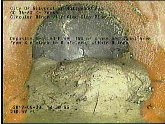
08e3bdb3-c547-440d-9ce2-4f488b39d18b_20190530_143330_797.jpg, 00:15:20, 210.59ft Deposits Settled Fine, 15% of cross sectional area from 4 o'clock to 8 o'clock, within 8 inch / AT END OF PIPE
