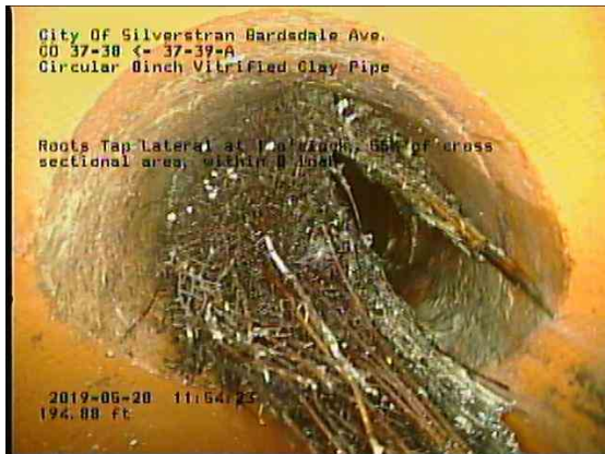
24d36d81-4ea5-4bc7-8580-171333341682_20190528_115657_519.jpg, 00:14:25, 194.88ft Roots Tap Lateral at 1 o'clock, 55% of cross sectional area, within 8 inch
