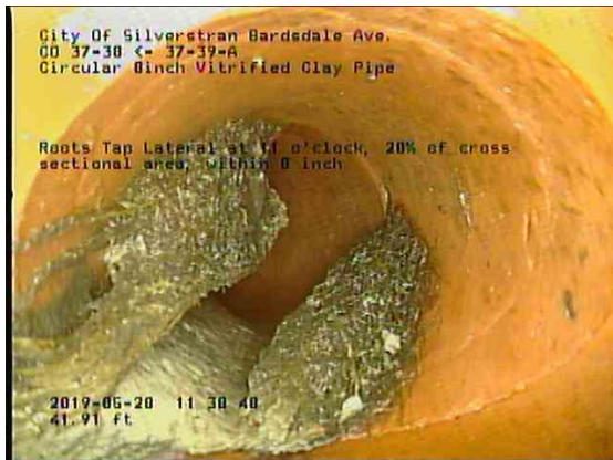
6c7bf4ef-8359-42ec-9a63-d3c4f7994cb1_20190528_114122_348.jpg, 00:02:46, 41.91ft Roots Tap Lateral at 11 o'clock, 20% of cross sectional area, within 8 inch
