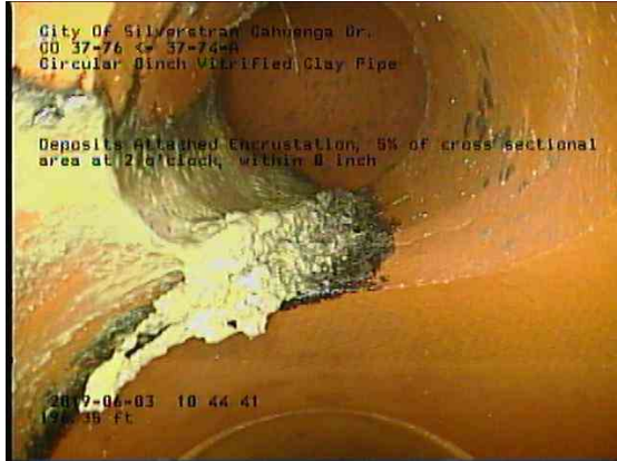
3229ddbc-891d-46c7-a420-7b6a2e498a32_20190603_104717_593.jpg, 00:13:28, 196.35ft Deposits Attached Encrustation, 5% of cross sectional area at 2 o'clock, within 8 inch / IN WYE
