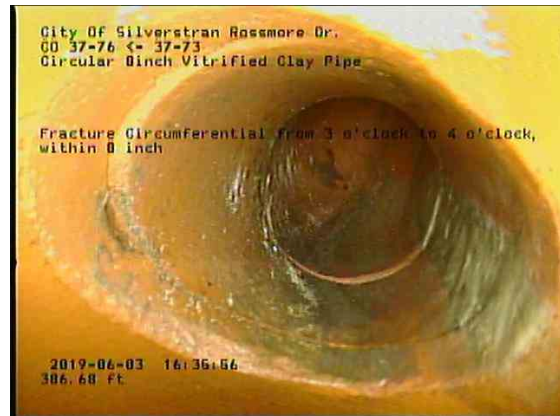
c6886c92-6e49-43dd-8be3-d7e56b1682c7_20190603_163833_325.jpg, 00:24:35, 386.68ft Fracture Circumferential from 3 o'clock to 4 o'clock, within 8 inch / IN WYE
