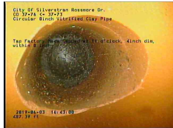
f353751a-6612-4e35-aaed-0af51fb0fe4a_20190603_164537_347.jpg, 00:30:17, 487.39ft Tap Factory Made Capped at 11 o'clock, 4inch dim, within 8 inch
