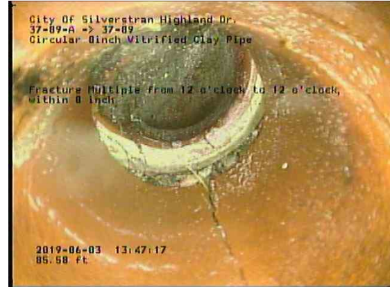
93ef1b56-c4ba-4a02-9ab2-22508033f8b0_20190603_134954_286.jpg, 00:10:56, 85.58ft Fracture Multiple from 12 o'clock to 12 o'clock, within 8 inch / IN WYE
