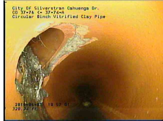
9b0aabdb-3716-4215-b85a-31473ba5324c_20190603_105937_479.jpg, 00:21:14, 320.95ft Roots Tap Lateral at 10 o'clock, 10% of cross sectional area, within 8 inch
