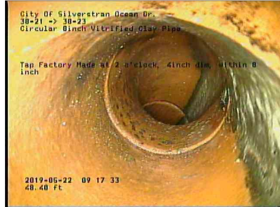
517f4d73-9525-42e9-87d3-69c238d120e3_20190522_092004_691.jpg, 00:03:20, 48.40ft Tap Factory Made at 2 o'clock, 4inch dim, within 8 inch
