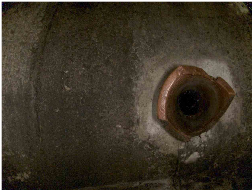
36-61_cd22f785_8cc2_4e9f_ab8d_76fe60c0a5c6_445111ff-880c-4507-bf53-d0cfc50823d2_P12.jpg, , 4.57 Broken at 3 o'clock, within 8 inch
