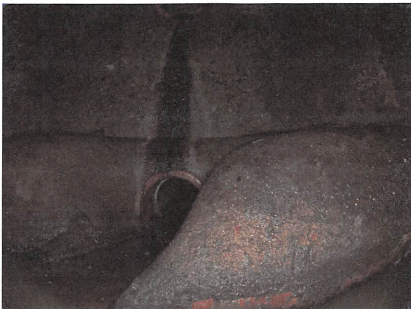
37-68_bc075bf7_3f28_485d_aaf8_7573fec9cbd6_7ffa3598-f871-4d67-9c66-1222b789523f_P12.jpg, , 9.06 Surface Roughness Increased from 12 o'clock to 12 o'clock, within 8 inch, Finish
