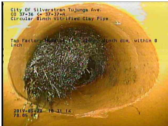
1c4fd1a7-fe72-48bc-a7d4-268d43c293fe_20190528_103347_331.jpg, 00:04:24, 78.05ft Tap Factory Made at 11 o'clock, 4inch dim, within 8 inch
