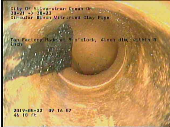
3e924574-cf32-4c76-ae7d-934d7194c926_20190522_091928_507.jpg, 00:02:52, 46.18ft Tap Factory Made at 9 o'clock, 4inch dim, within 8 inch
