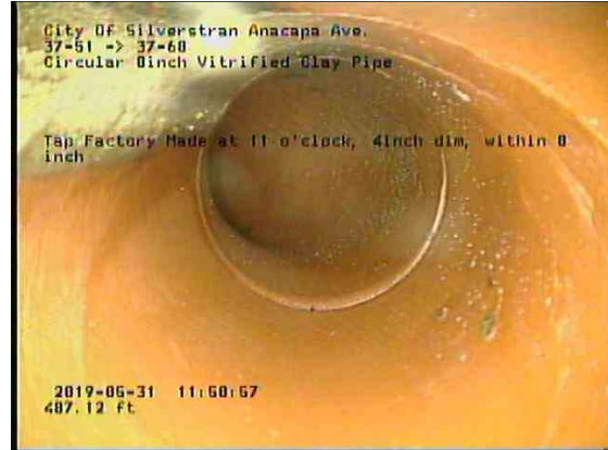
9cbe547f-de9c-43a4-b0d9-7363ad9cd042_20190531_115334_119.jpg, 00:29:46, 487.11ft Tap Factory Made at 11 o'clock, 4inch dim, within 8 inch
