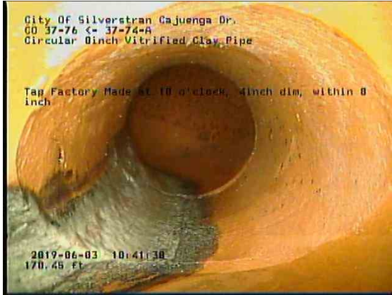
ffe1913b-81f3-481c-901a-68ae10cfc06f_20190603_104414_889.jpg, 00:11:53, 170.45ft Tap Factory Made at 10 o'clock, 4inch dim, within 8 inch
