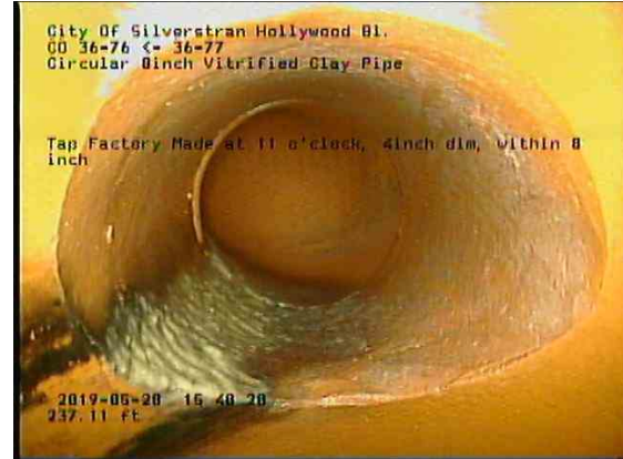
b2a9b32e-3da9-4684-bd3c-4cb0697634ee_20190528_154254_535.jpg, 00:12:56, 237.11ft Tap Factory Made at 11 o'clock, 4inch dim, within 8 inch
