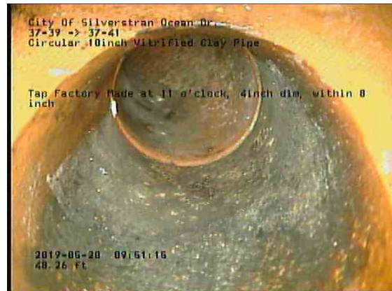
2264be18-31f8-472d-b8a1-86ef3c3d7800_20190528_095348_277.jpg, 00:04:28, 48.25ft Tap Factory Made at 11 o'clock, 4inch dim, within 8 inch
