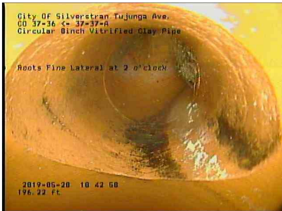
dd03a388-54a3-4bf5-9bd7-d31b7c3586e0_20190528_104531_161.jpg, 00:11:57, 196.22ft Roots Fine Lateral at 2 o'clock
