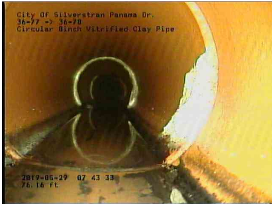
05338be0-a8cd-4747-b27d-8fe4261dde16_20190529_074606_945.jpg, 00:06:50, 76.90ft Deposits Attached Encrustation, 5% of cross sectional area from 3 o'clock to 5 o'clock, within 8 inch
