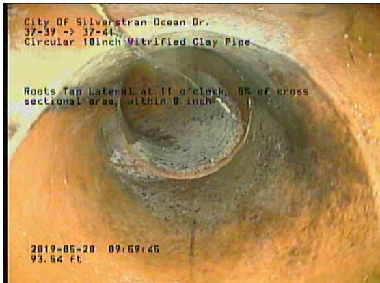
3450ade4-7d82-4ef7-a00c-298becd997ae_20190528_100218 _172.jpg, 00:06:23, 93.54ft Roots Tap Lateral at 11 o'clock, 5% of cross sectional area, within 8 inch
