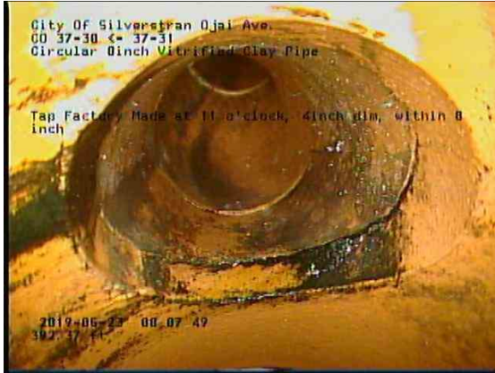
41e36f61-f4bc-43ec-8b81-40c9261d6e0d_20190523_081021_829.jpg, 00:24:54, 392.37ft Tap Factory Made at 11 o'clock, 4inch dim, within 8 inch
