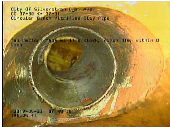
ac64df33-4339-47cd-b811-df8248b30ef7_20190523_075108_264.jpg, 00:11:21, 196.23ft Tap Factory Made at 11 o'clock, 4inch dim, within 8 inch
