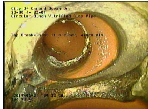
b4bca342-6ee4-4e3e-9dbd-a1af64d6952f_20190521_093628_878.jpg, 00:17:48, 334.98ft Tap Break-In at 11 o'clock, 4inch dim
