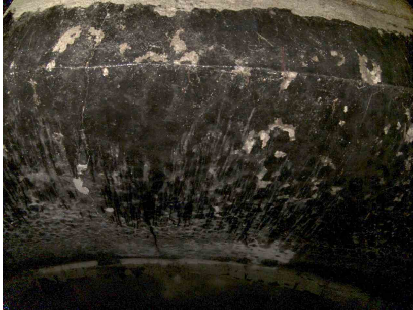
37-37-A_f72c6802_8707_4f2c_ab45_dae33749b1ef_dfbea1d7-f8d9-486f-9717-9852637f3dce_P12.jpg, , 1.13 Fracture Longitudinal at 8 o'clock, within 8 inch
