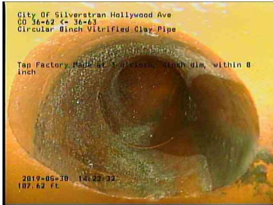
8126748b-e581-4d30-bfa6-e451d8d9b827_20190530_142507_952.jpg, 00:08:51, 107.62ft Tap Factory Made at 3 o'clock, 4inch dim, within 8 inch
