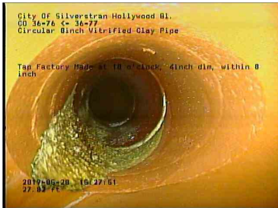
d87cf45c-85cd-4785-b0cc-1ed4334b09bd_20190528_153025_511.jpg, 00:02:10, 27.82ft Tap Factory Made at 10 o'clock, 4inch dim, within 8 inch
