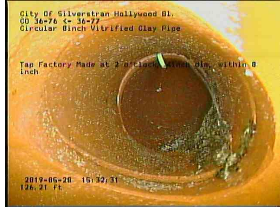
befaaea7-10aa-45a1-ab58-d68d4a3d355d_20190528_153505_347.jpg, 00:06:25, 126.21ft Tap Factory Made at 2 o'clock, 4inch dim, within 8 inch
