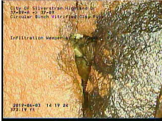
a7ef19e3-a34b-419d-84ad-87eba618bfd2_20190603_142200_896.jpg, 00:33:36, 372.19ft Infiltration Weeper at 2 o'clock
