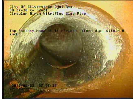
dd6a96c3-53b4-4f22-892a-349a17fdf799_20190523_075958_581.jpg, 00:17:09, 291.78ft Tap Factory Made at 11 o'clock, 4inch dim, within 8 inch
