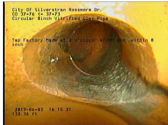
9ed405cd-745c-4d54-9658-2195eeb78141_20190603_161758_421.jpg, 00:08:18, 132.36ft Tap Factory Made at 2 o'clock, 4inch dim, within 8 inch
