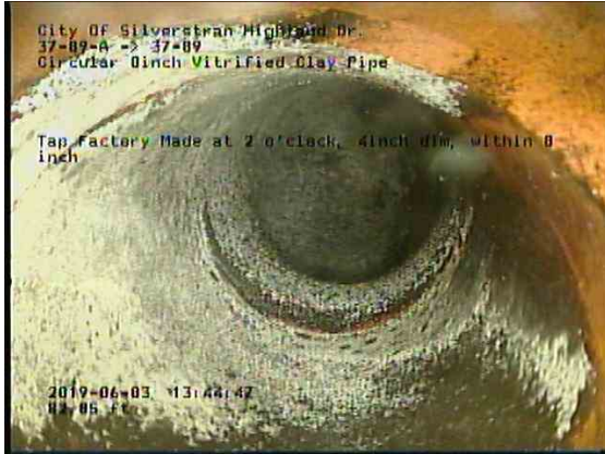
ce9d8a80-85bd-45ac-95cc-5843347ade44_20190603_134723_913.jpg, 00:09:23, 82.85ft Tap Factory Made at 2 o'clock, 4inch dim, within 8 inch
