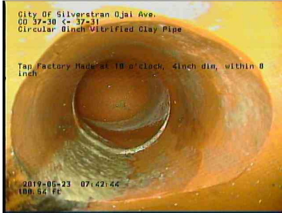
4fa61006-f49e-425e-b70c-5cd349120f48_20190523_074517_094.jpg, 00:06:18, 100.52ft Tap Factory Made at 10 o'clock, 4inch dim, within 8 inch
