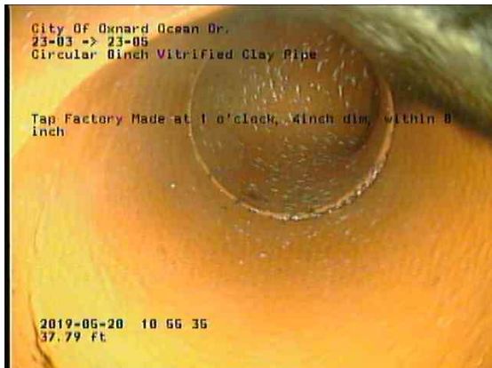
deddc54d-eaf7-4d9a-a688-f67c60210bd7_20190520_105804_932.jpg, 00:01:53, 37.79ft Tap Factory Made at 1 o'clock, 4inch dim, within 8 inch
