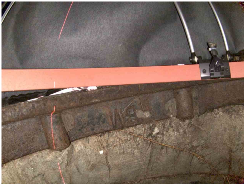
37-39-A_545e9b99_6729_4fa7_8d17_f1c1b7c45969_dce70485-e3a8-458b-be12-30db902776b3_P12.jpg, , 0.19 Roots Fine Joint from 7 o'clock to 9 o'clock, within 8 inch
