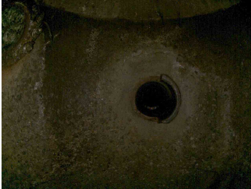
37-35_f6e7d8ee_4d76_46d5_86b4_5a5b78e4e34f_ea693865-090c-408a-ae20-f61122aed053_P12.jpg, , 4.83 Broken at 1 o'clock, within 8 inch
