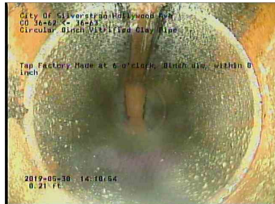
c84ad29a-0377-4601-b028-57865229f460_20190530_141329_205.jpg, 00:01:47, 0.21ft Tap Factory Made at 6 o'clock, 8inch dim, within 8 inch
