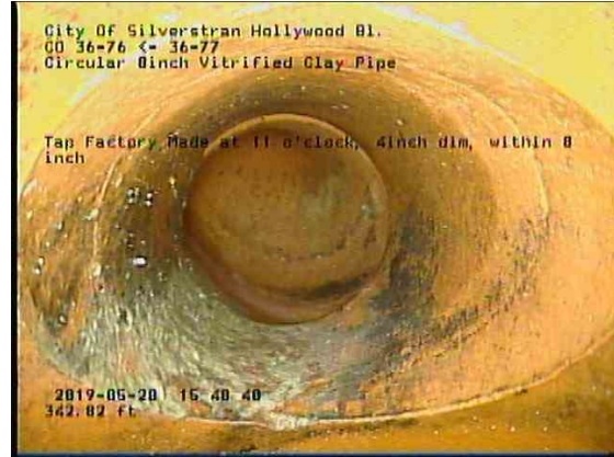
9cd28e29-8235-46a9-9396-8535b1fb634a_20190528_155114_380.jpg, 00:19:56, 342.82ft Tap Factory Made at 11 o'clock, 4inch dim, within 8 inch
