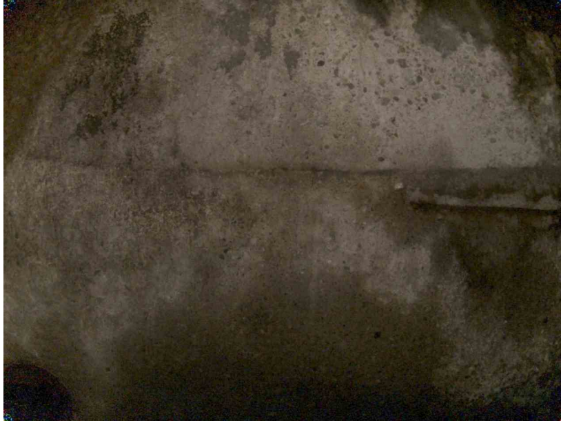
36-63_91085e16_b10b_42df_8305_4acc6363b0ef_3c9fb24c-0144-441a-842a-88af86a4ca94_P12.jpg, , 3.41 Surface Reinforcement Corroded at 7 o'clock, within 8 inch
