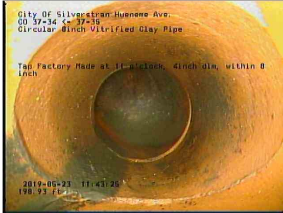
7d9b9ca0-4d13-4272-ac35-6016287206c2_20190523_114523_8_850.jpg, 00:13:42, 198.93ft Tap Factory Made at 11 o'clock, 4inch dim, within 8 inch
