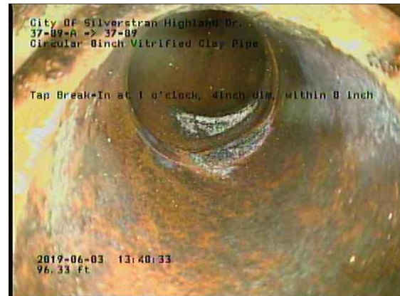
751ab6fd-f1d1-48d8-9fe2-7646fb9dc2db_20190603_135110_513.jpg, 00:12:06, 96.33ft Tap Break-In at 1 o'clock, 4inch dim, within 8 inch
