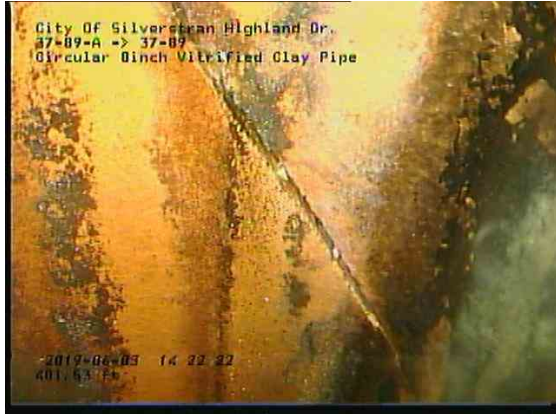
2901239f-e3cb-4134-9d86-e33ce9c7a19a_20190603_142459_687.jpg, 00:36:02, 401.53ft Fracture Spiral from 4 o'clock to 6 o'clock, within 8 inch
