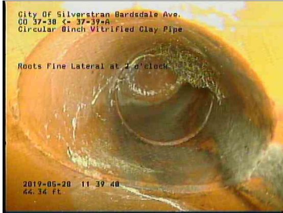
5e5e62d9-934a-48c9-b399-f7e453d832fe_20190528_114214_523.jpg, 00:03:24, 44.34ft Roots Fine Lateral at 2 o'clock
