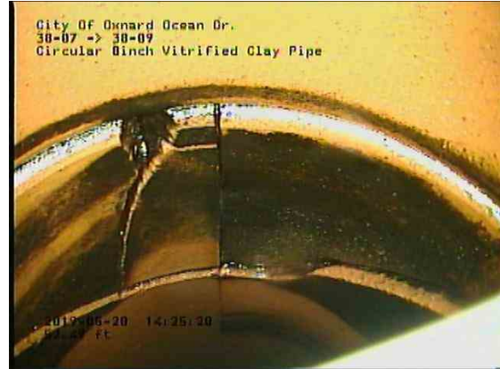
4955873e-29b7-464d-96b0-8ad03ae0977d_20190520_142750_063.jpg, 00:05:13, 52.86ft Broken from 11 o'clock to 3 o'clock, within 8 inch
