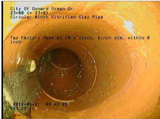
bf54d906-c6c6-4c5d-8458-f91bb54c5576_20190521_094551_959.jpg, 00:26:17, 503.22ft Tap Factory Made at 10 o'clock, 6inch dim, within 8 inch
