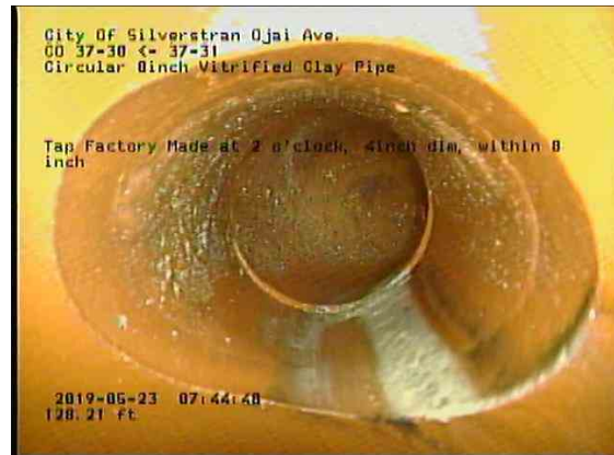
0c3ada3c-9a80-462d-b9e8-c7d782caf675_20190523_074721_067.jpg, 00:07:56, 128.21ft Tap Factory Made at 2 o'clock, 4inch dim, within 8 inch
