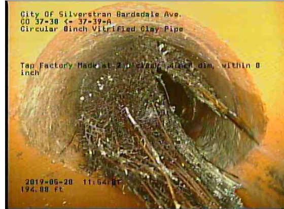
4f2a16a0-15a5-40ea-be0c-5221551049f3_20190528_115634_960.jpg, 00:14:22, 194.88ft Tap Factory Made at 2 o'clock, 4inch dim, within 8 inch
