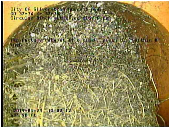
bd27cc9d-834f-48f4-b88e-910919b13de9_20190523_120445_436.jpg, 00:28:42, 434.90ft Tap Factory Made at 11 o'clock, 4inch dim, within 8 inch
