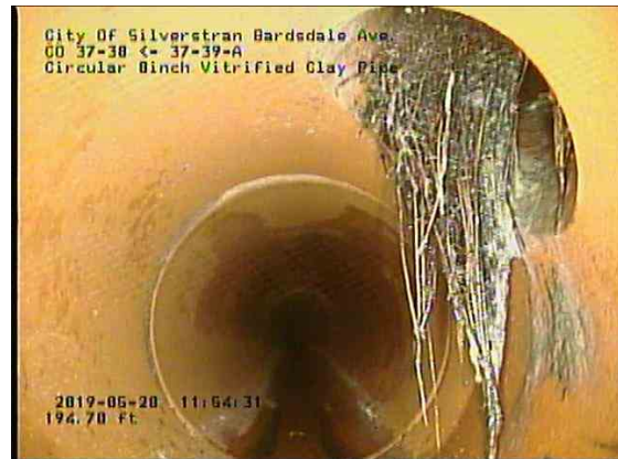
34c69783-c5b5-449a-bb18-560b71335c67_20190528_115705_339.jpg, 00:14:25, 194.88ft Roots Tap Lateral at 1 o'clock, 55% of cross sectional area, within 8 inch
