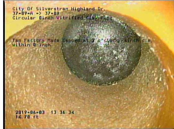
8a04a563-4c17-4786-a53f-123dc068898b_20190603_133910_847.jpg, 00:04:03, 14.70ft Tap Factory Made Capped at 2 o'clock, 4inch dim, within 8 inch
