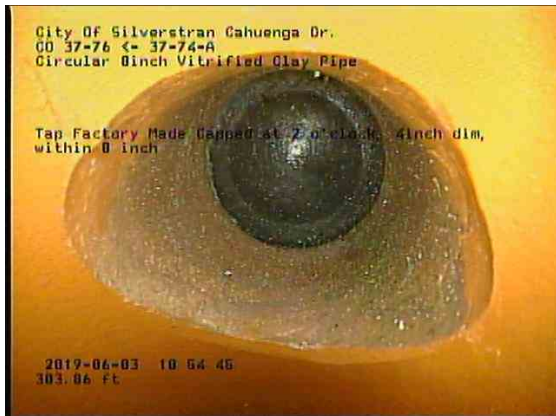
d12a8c9c-22eb-4714-8f15-870383954355_20190603_105721_722.jpg, 00:19:58, 303.86ft Tap Factory Made Capped at 2 o'clock, 4inch dim, within 8 inch
