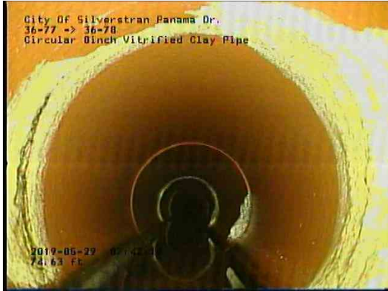
b66e019d-041d-4d27-80cf-c7e8563aedba_20190529_074448_656.jpg, 00:05:51, 75.64ft Deposits Attached Encrustation, 5% of cross sectional area from 7 o'clock to 5 o'clock, within 8 inch
