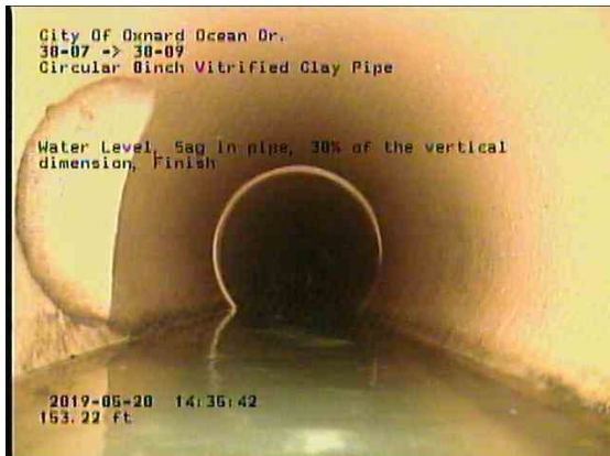
291413a8-d7a7-4de6-bcbd-18e7d9b92a96_20190520_143812_042.jpg, 00:13:02, 153.22ft Water Level, Sag in pipe, 30% of the vertical dimension, Finish
