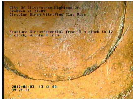
559418bf-d967-4221-9fe8-b4c242aebbf2_20190603_134337_212.jpg, 00:06:10, 39.90ft Fracture Circumferential from 12 o'clock to 12 o'clock, within 8 inch / IN WYE
