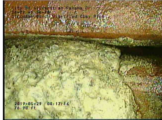
d7fd641b-8bce-4f9c-a67b-de69d430b831_20190529_081948_335.jpg, 00:06:50, 76.90ft Deposits Attached Encrustation, 5% of cross sectional area from 3 o'clock to 5 o'clock, within 8 inch
