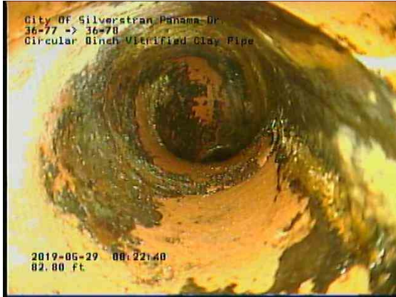
84d5df85-9db7-47d4-ae2c-c53e447ef2d8_20190529_082514_019.jpg, 00:10:42, 82.80ft Tap Factory Made at 3 o'clock, 4inch dim, within 8 inch
