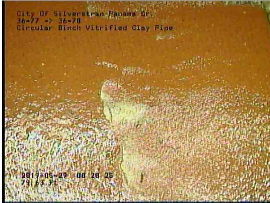
8289c662-ee4e-4ef1-a8ea-da3ad1b51559_20190529_082259_737.jpg, 00:08:34, 79.63ft Crack Longitudinal at 3 o'clock, within 8 inch
