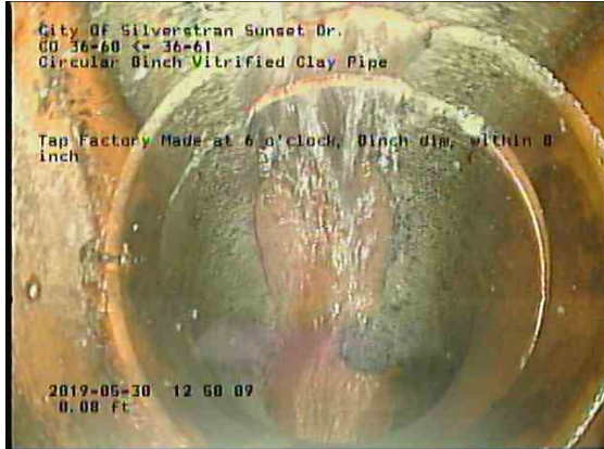
45f613dc-235e-4a94-9817-a5fd99b287d3_20190530_125244_977.jpg, 00:01:32, 0.08ft Tap Factory Made at 6 o'clock, 8inch dim, within 8 inch
